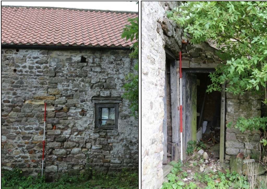
Plates 8 and 9: the vertical wall join between Bay 2 (left) and 3 (right) on the south-west elevation, and the outbuilding at the southern end of this wall
