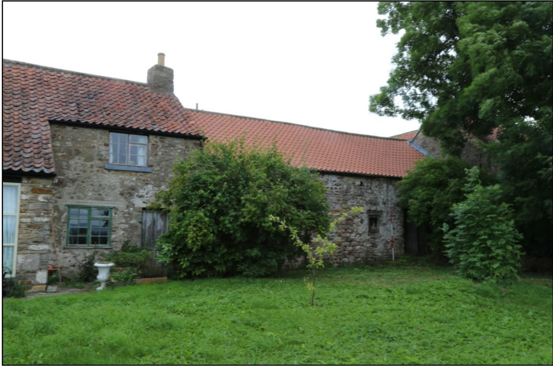
Plate 7: the south-west elevation of the Barn at Lowside Farm, showing Bay 1 (left) to Bay 3 (right)
