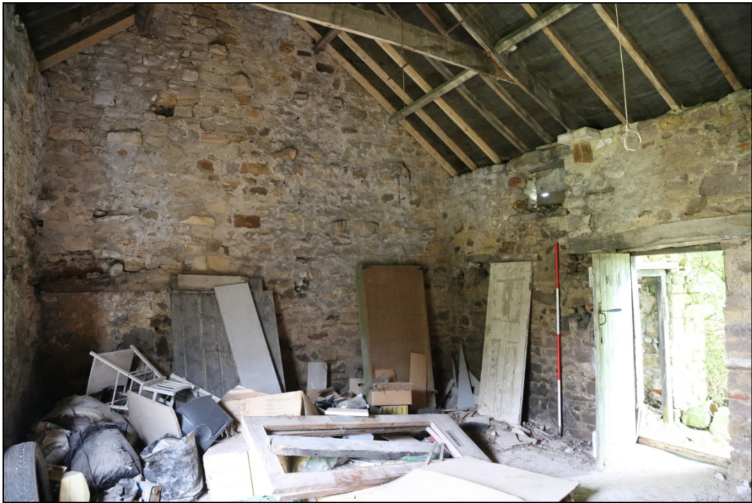
Plate 14: Bay 3, looking south, showing the loft opening on the south-eastern wall, and the door with timber lintel
