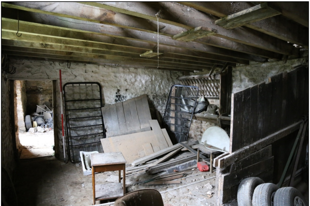
Plate 13: Bay 2G, looking south-east showing the loft joists, and later divisions which were evidence of the use of this space as stables
