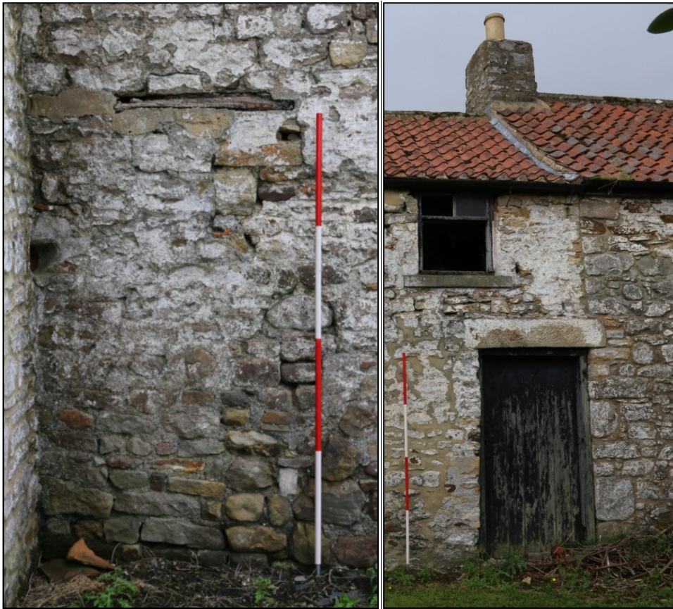
Plates 5 and 6: the blocked doorway in the southern end of the north-east elevation, and the join between Bays 1 and 2, showing the possible position of the cross-passage
