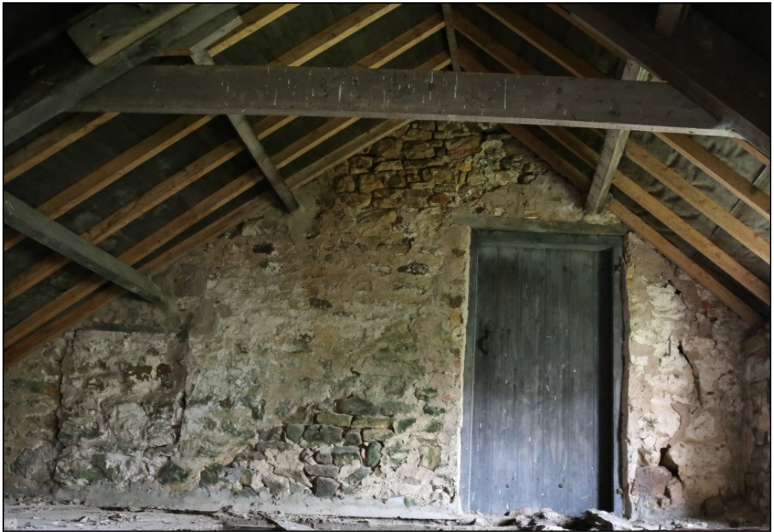
Plate 12: a wall scar showing the roof pitch and chimney outline of the Phase 1 building gable in the north-west wall, truncated by a later doorway
