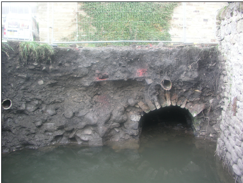
Plate 1: southern end of stone arched culvert, at exit point into open section
