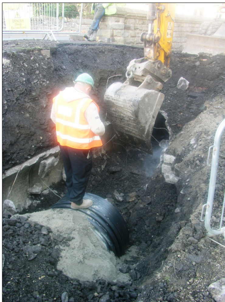
Plate 3: removal of concrete culvert; a short stub of the culvert wall is visible to the right of the concrete culvert
