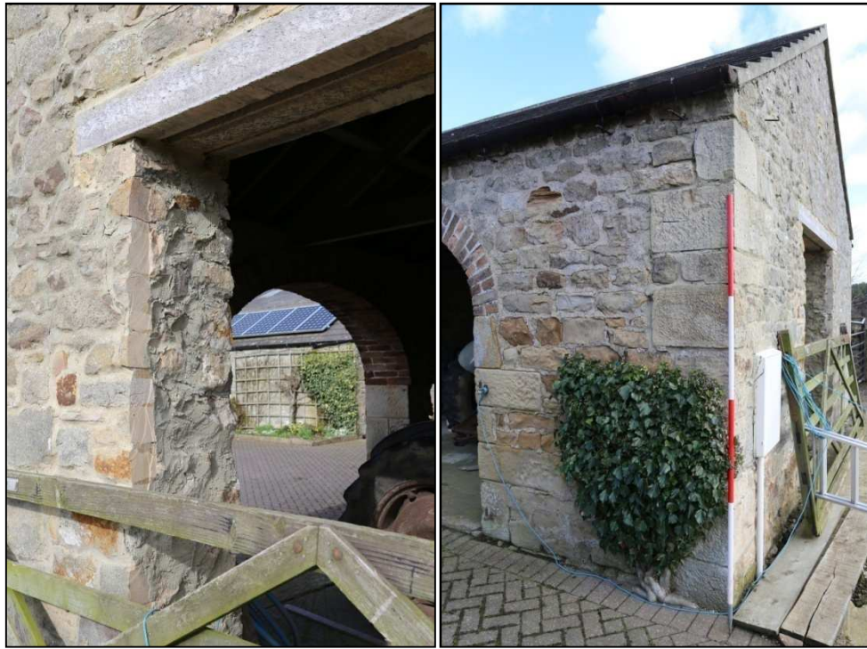
Plates 9 and 10: Opening in the south elevation (a later insertion), and the rebuilt south-west corner of the cart shed, location of the former blacksmith's forge
