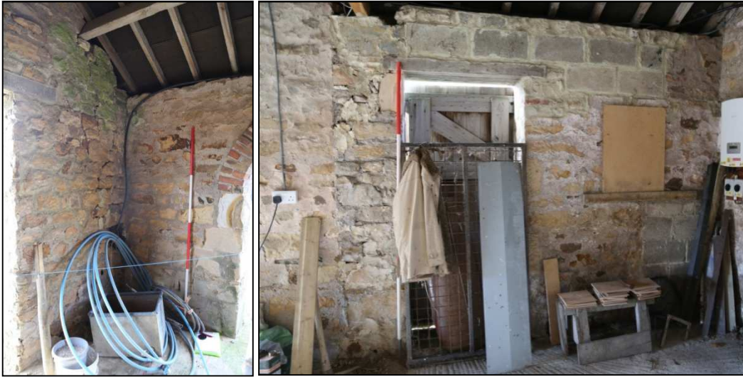
Plates 16 and 17: Partially rebuilt south-west corner of the cart shed, and the north end of the west wall
