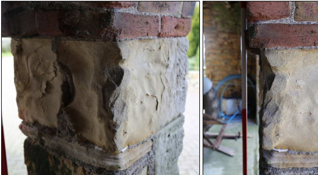
Plates 18 and 19: Severe lamination of stone blocks forming the arch piers
