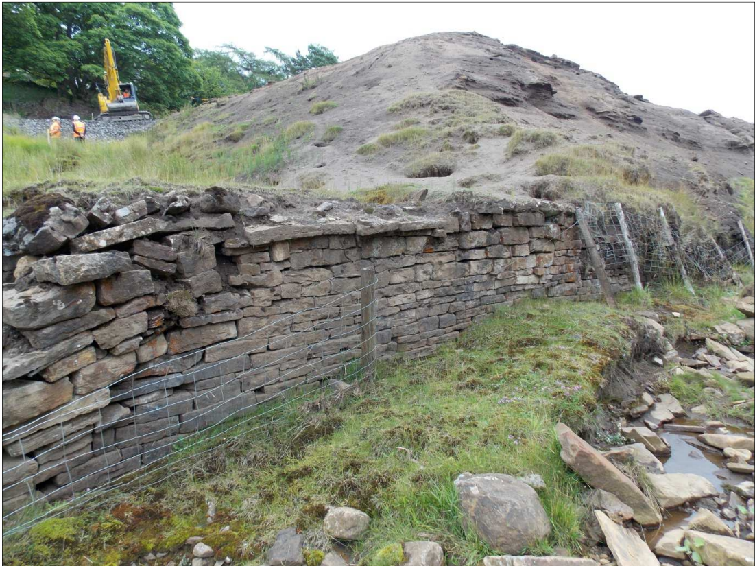
Plate 6. Outer face of river wall showing 'string course' (centre), possibly representing the location of a foot-bridge
