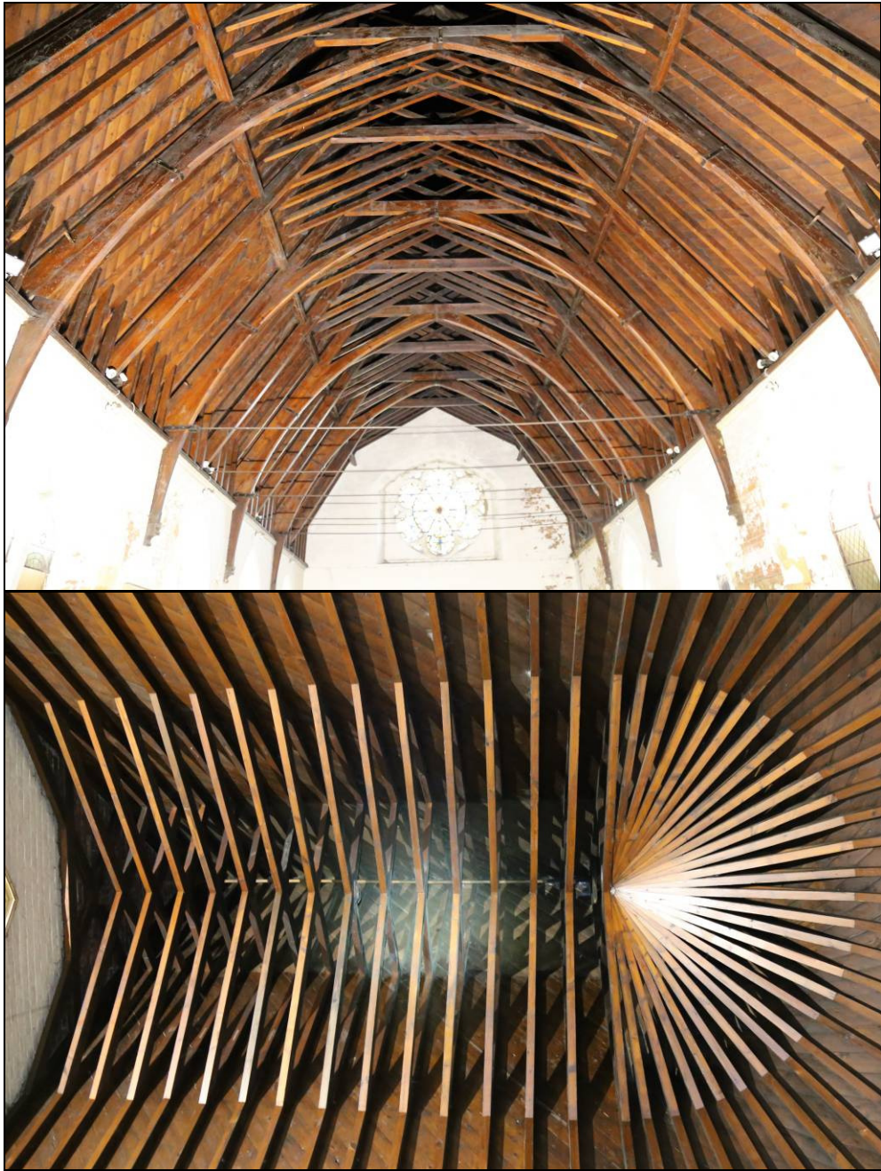
Plate 11: the nave roof, facing west (top) and chancel roof, looking up (bottom)
