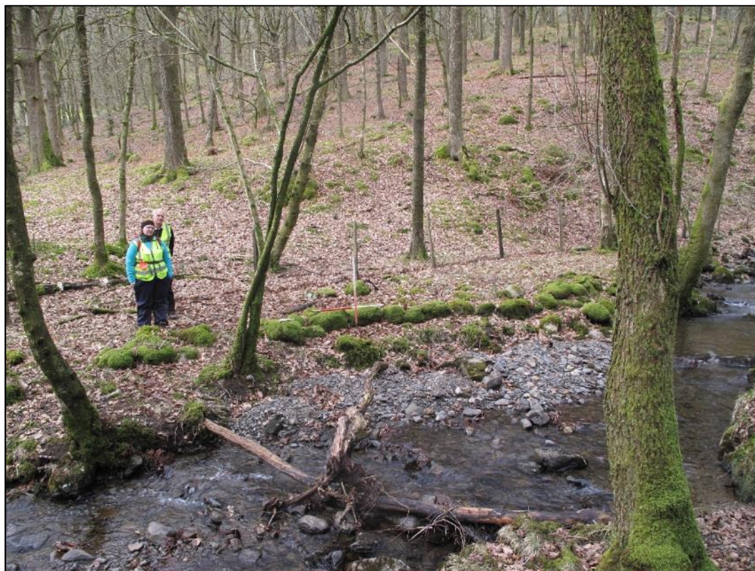
Plate 40: revetment wall (19/006) that would have reinforced a working platform next to the stream that creates a boundary between Linsty Hall and Tom Parrocks woods.
