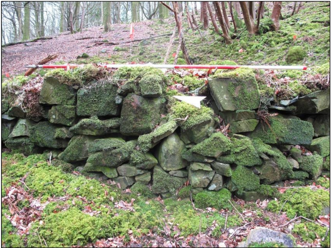
Plate 63: a pitstead on a steep slope is reinforced with a revetment wall.
