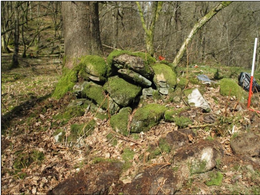
Plate 33: damage to a charcoal burner or bark peeler's hut (18/031) caused by tree growth.
