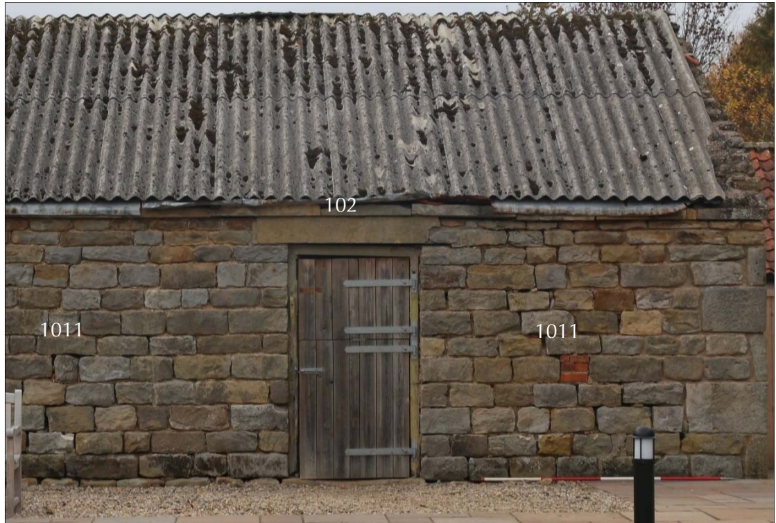
Plate 18: broken lintel above door 102 of the east elevation. On either side of the door are filled niches 1011; the north one is filled with brick, the south with stone.
