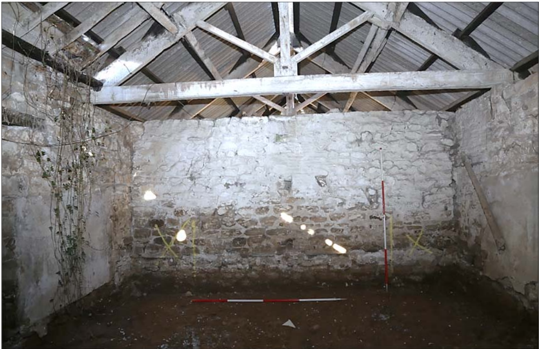
Plate 31: north elevation of room 200. A line of joist holes visible in the centre of the north wall are associated with former stall divisions. Render is visible on both the east and west walls.
