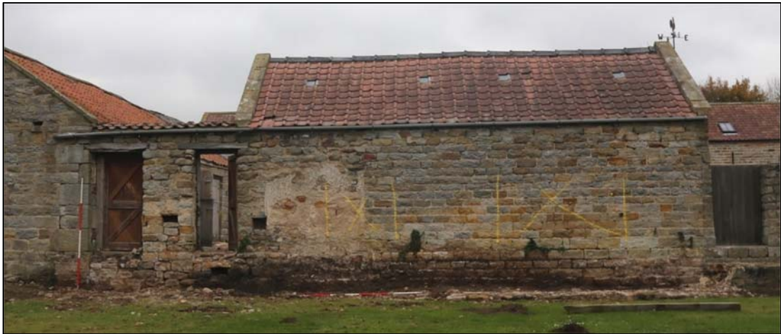
Plate 46: south facing elevation (2500) of the south range, showing the wall footings (2704) of demolished range (2700).
