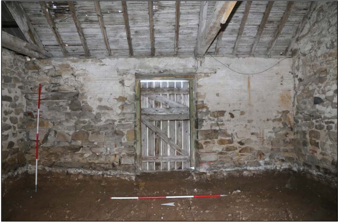
Plates 35: east wall featuring door (302). Evidence of feeding trough (304) still visible in north-east corner, to the left.
