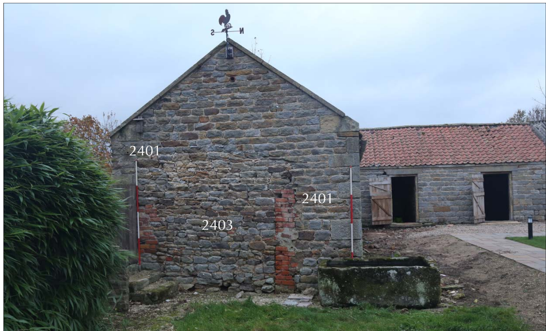
Plate 44: east elevation of the south range showing the walls scar (2401) and the rubble infill (2403).
