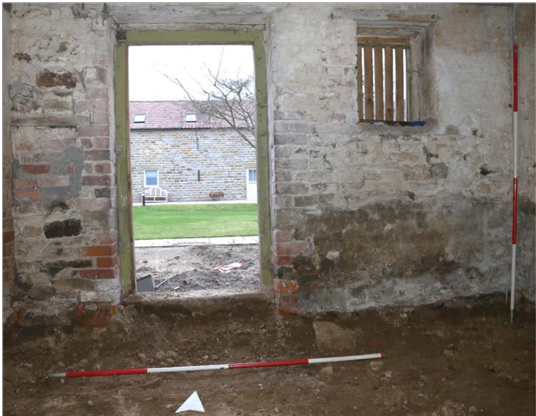
Plate 53: room 2200 looking north, showing door 2201 and window 2202. Note bullnose brick around the door frame.
