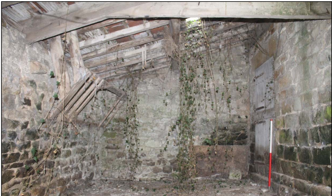
Plate 42: view of the outshot looking north. The hay rack is visible on the west wall along with the roof structure. (Photo by CS Archaeology 2018).
