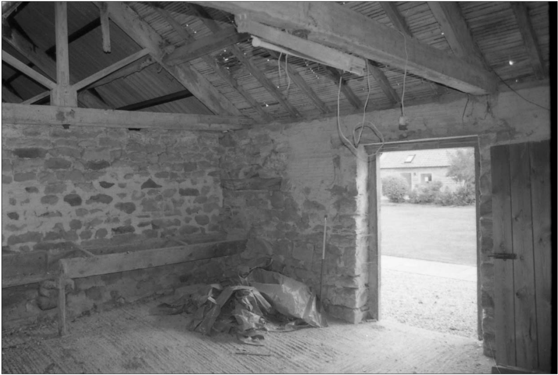
Plate 33: room 300 looking north-east with the feeding trough visible along the north wall and the concrete screed floor in-situ. (Photo by CS Archaeology 2018).
