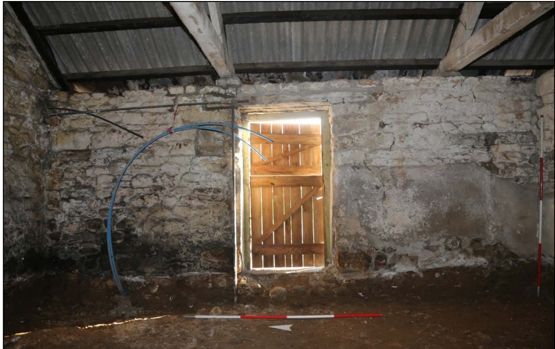
Plate 28: east door (101) with lamp niche (103) visible to the left. The west door (102) has the same layout.
