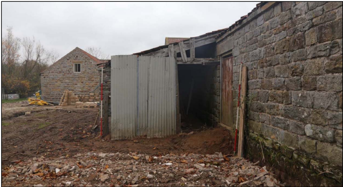
Plate 41: entrance into outshot from the west side of the range, looking north.
