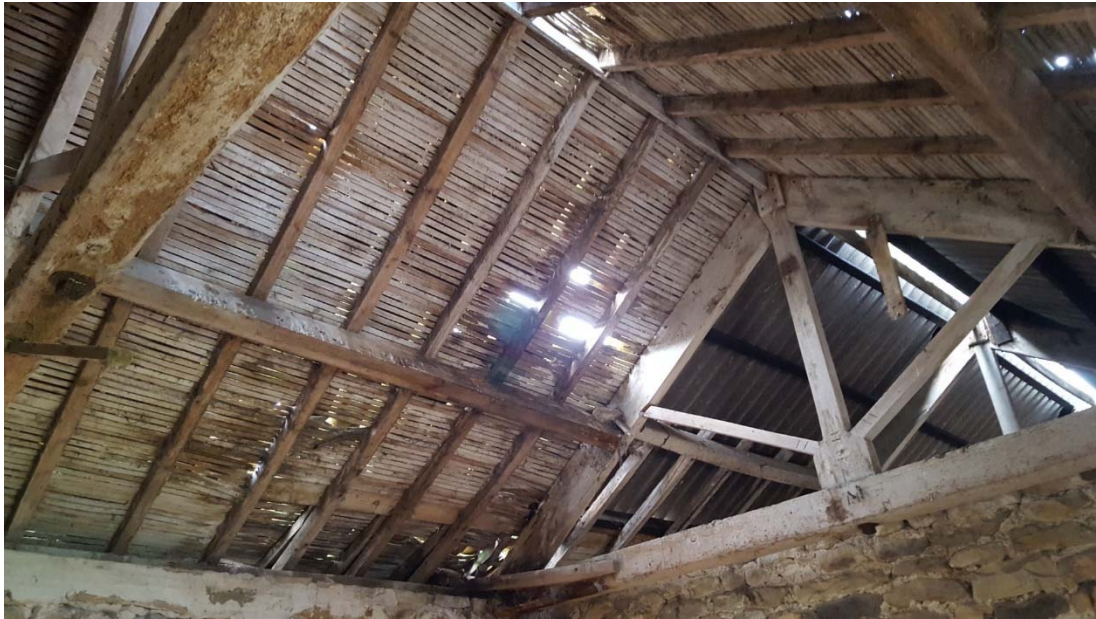
Plate 32: division between corrugated iron roof and lath and plaster roof in room 300.
