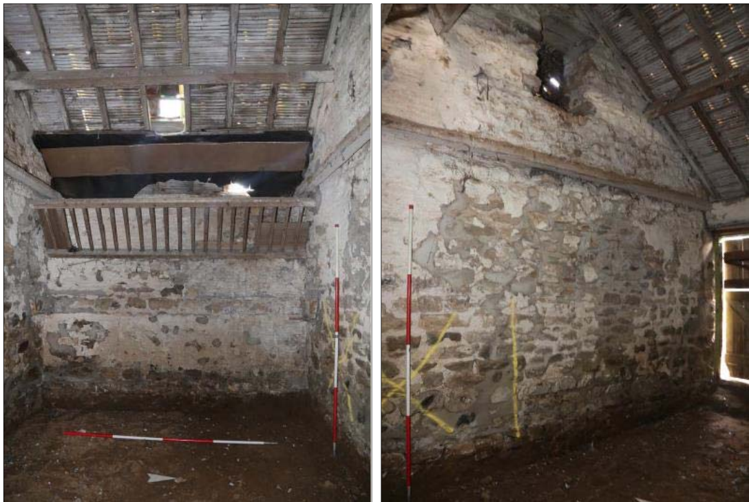
Plates 39 and 40: view of loose box 500 looking west showing in-situ hay rack (502) and oblique view of north dividing wall, showing opening 405 providing access between the two rooms at this level, as well as ventilation.
