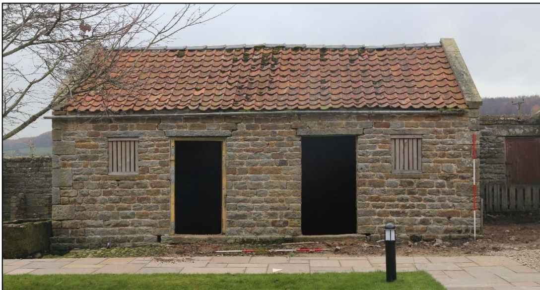
Plate 43: north (front) elevation of the south range (2300). The cobbled pavement (2301) is visible to the left of and behind the horizontal ranging rod.
