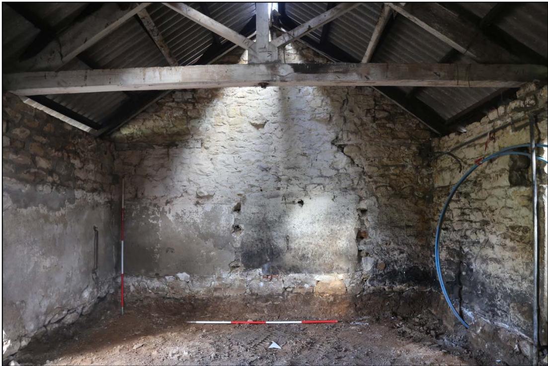
Plate 27: north wall of room 100. Linear joist holes (111) are visible as scars on the wall. Two horizontal timbers (110) are visible in the wall above the joist holes.
