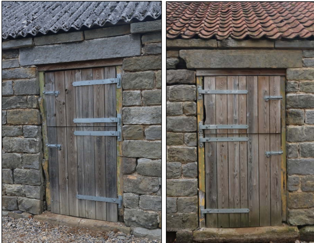
Plates 16 and 17: oblique view of door 202 with the wooden latches (in yellow) on the left side of the door frame (left) and door 401 showing broken lintel (right).
