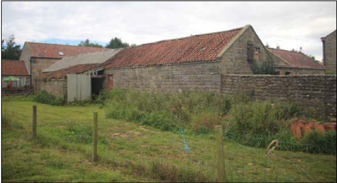
Plate 23: oblique view of west elevation showing build-up of ground deposits along the base of the wall. (Photo by CS Archaeology).
