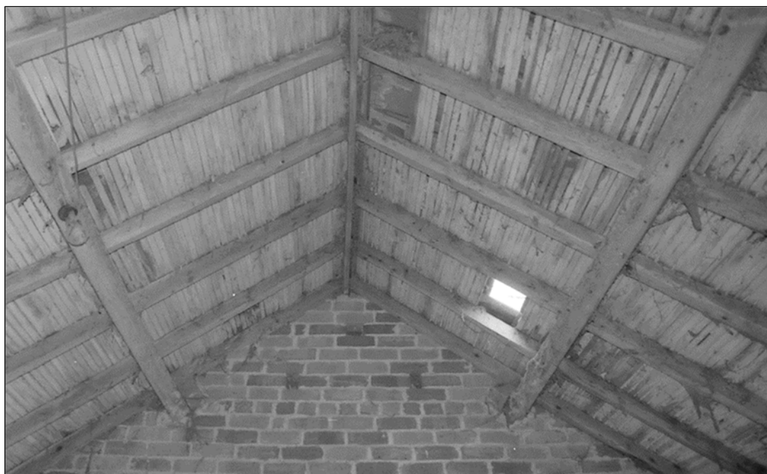
Plate 51: room 2100 roof structure, also visible are the three ventilation holes (2106) and a skylight (2501). (Photo by CS Archaeology 2018).
