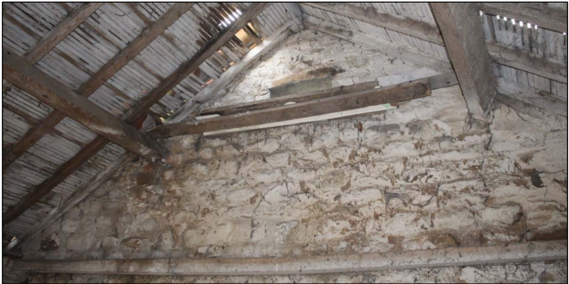
Plate 38: opening (506) on the south gable associated with the dovecot (1201). Below is the protruding tie-beam (504) which supported the hay loft floor. (Photo by CS Archaeology 2018).
