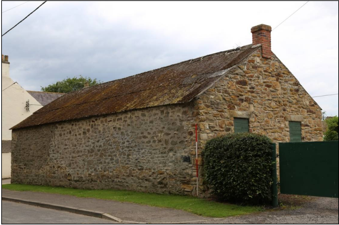
Plate 4: the north gable and eastern elevation of the Cart Shed, showing the original random-coursed rubble stone eastern wall, in comparison to the rebuilt northern wall
