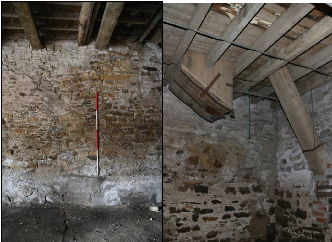
Plates 13 and 14: the vertical scar demonstrating the point from which the wall had been extended or rebuilt, and the timber chutes at the northern end of the interior
