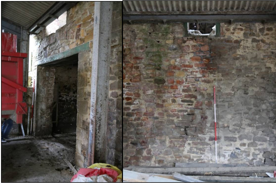
Plates 8 and 9: the doorway with relieving arch above at the northern end of the west elevation and the vertical wall scar demonstrating the point from which the wall was extended/rebuilt at the south end
