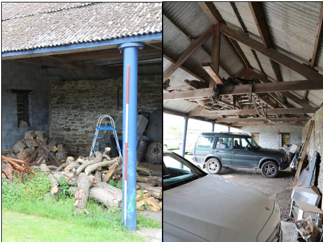
Plates 5 and 6: one of the cast iron posts on the open, west elevation of the Cart Shed, and the interior of the Cart Shed looking north
