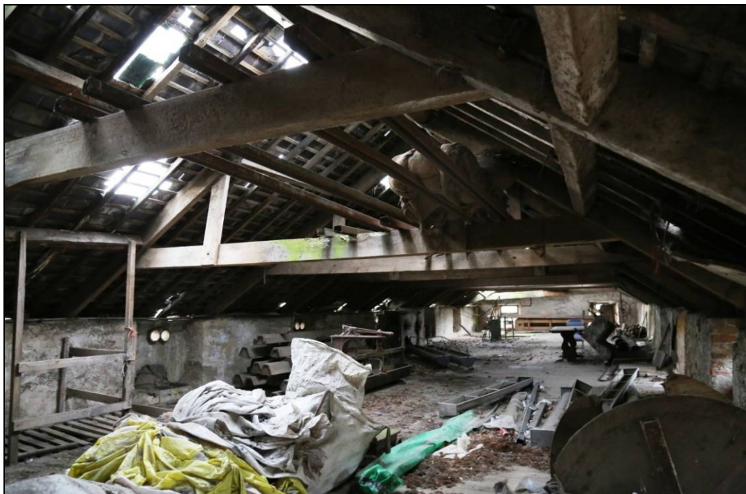
Plate 15: the loft of the Granary, looking south-east, taken from the top of the external stone steps
