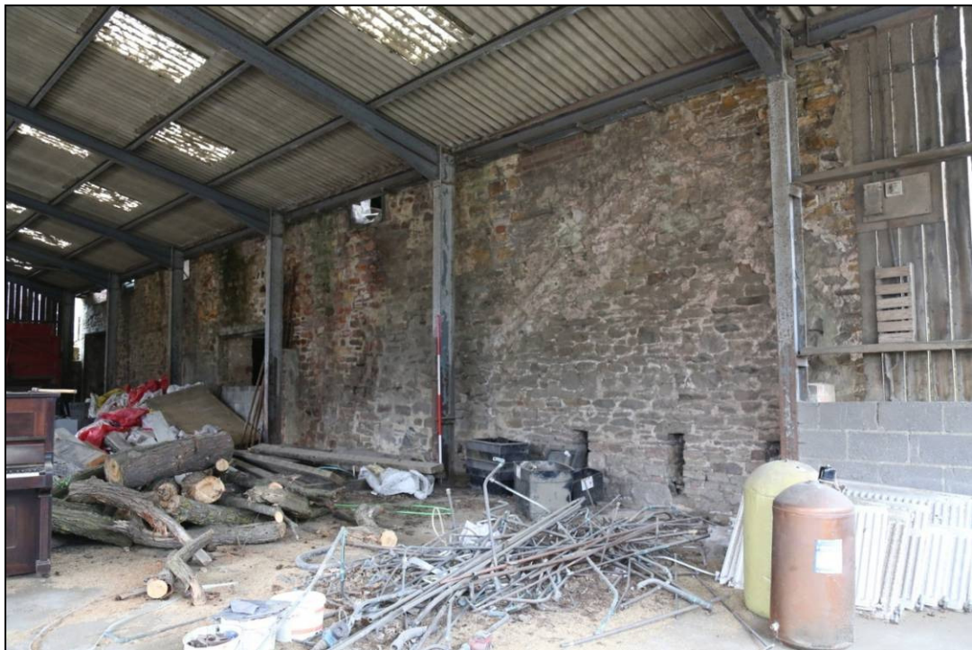
Plate 7: an oblique photograph of the west elevation of the Granary, looking north-east, showing the later rebuild/extension part of the wall, containing wall scar of former building and three slit vents
