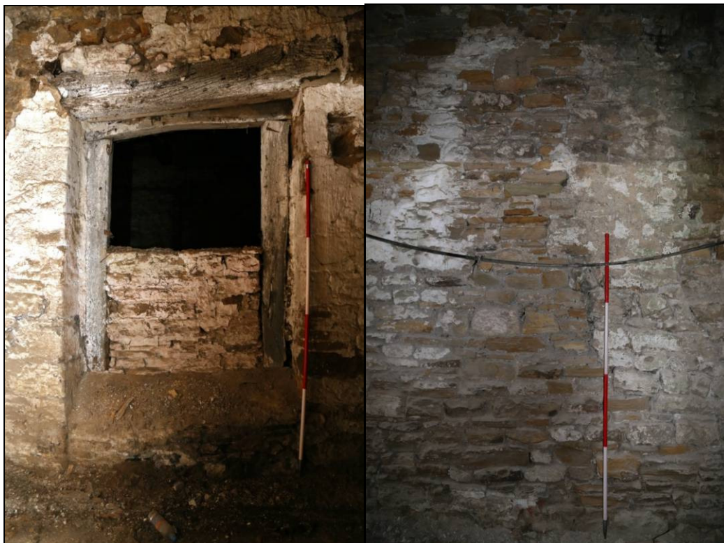
Plates 10 and 11: an original door on the east elevation, with timber lintel and jamb, and the vertical wall scar demonstrating the point at which the wall had been rebuilt/extended at the southern end
