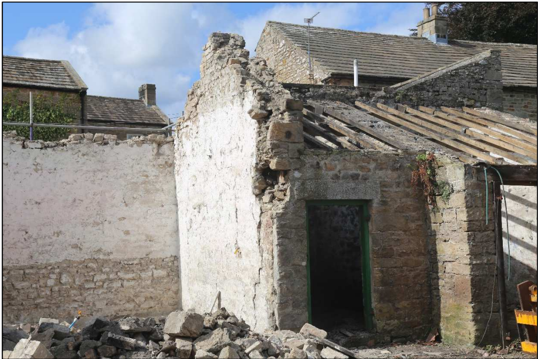
Plate 18: The garage and coal store. The crack in the southern wall indicates where the Phase III replacement joins the original wall.
