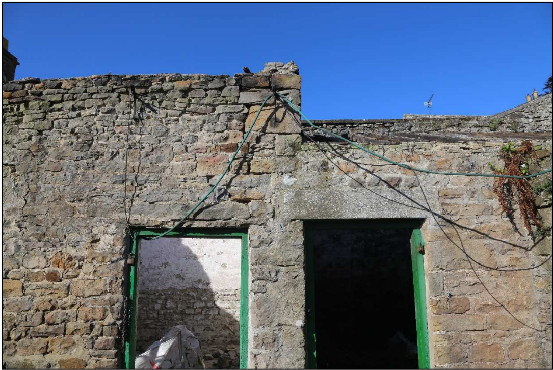
Plate 10: Point where the later 'kitchen' wall was keyed into the walls of the coal store.
