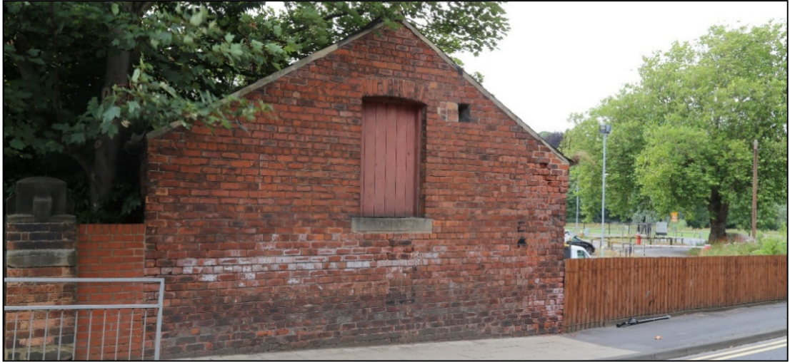
Plate 3: east elevation of the stable with the loading door (1131) and owl hole (1132).
