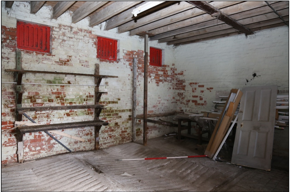
Plate 4: view of corner of the stables looking west. Visible are the louvre windows (1214), stall grooves (1211), drainage channel (1212) and feeding trough remains (1215).
