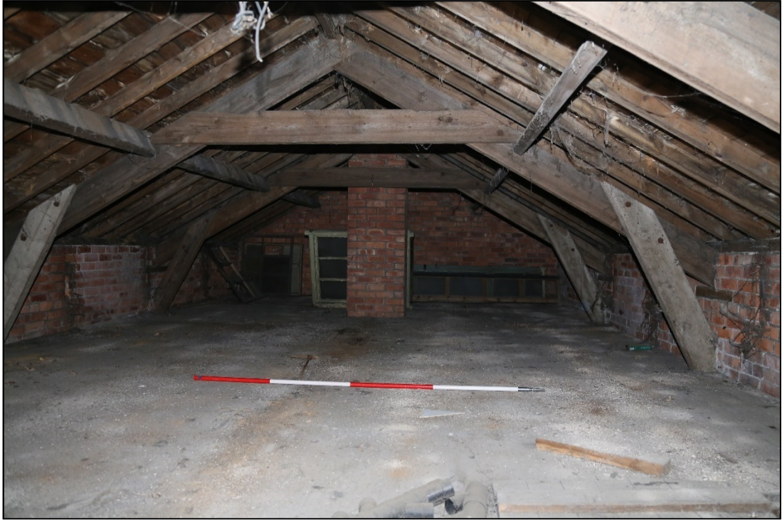
Plate 5: view of the hayloft looking south-west, with the chimney stack (1224) at the rear
