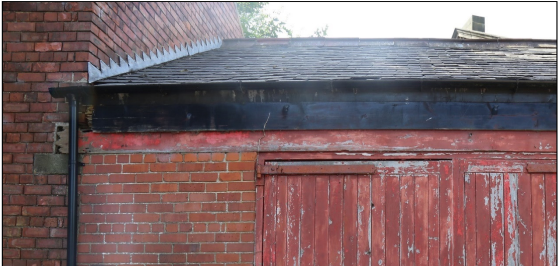
Plate 11: upper east corner of the cart shed where the beam is tied into the stable wall.
