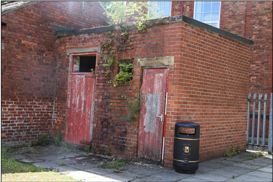
Plate 10: view of the outbuilding looking south onto both doors (3111 and 3112) and the small window (3113). The vent (3114) is barely visible behind some foliage.
