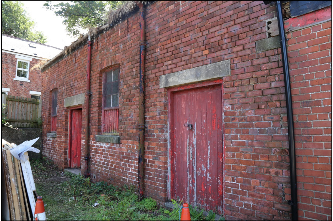
Plate 2: oblique view of the north elevation of the stable block, showing both doors (1111 and 1112), the windows (1113), and the ventilation slits (1114).
