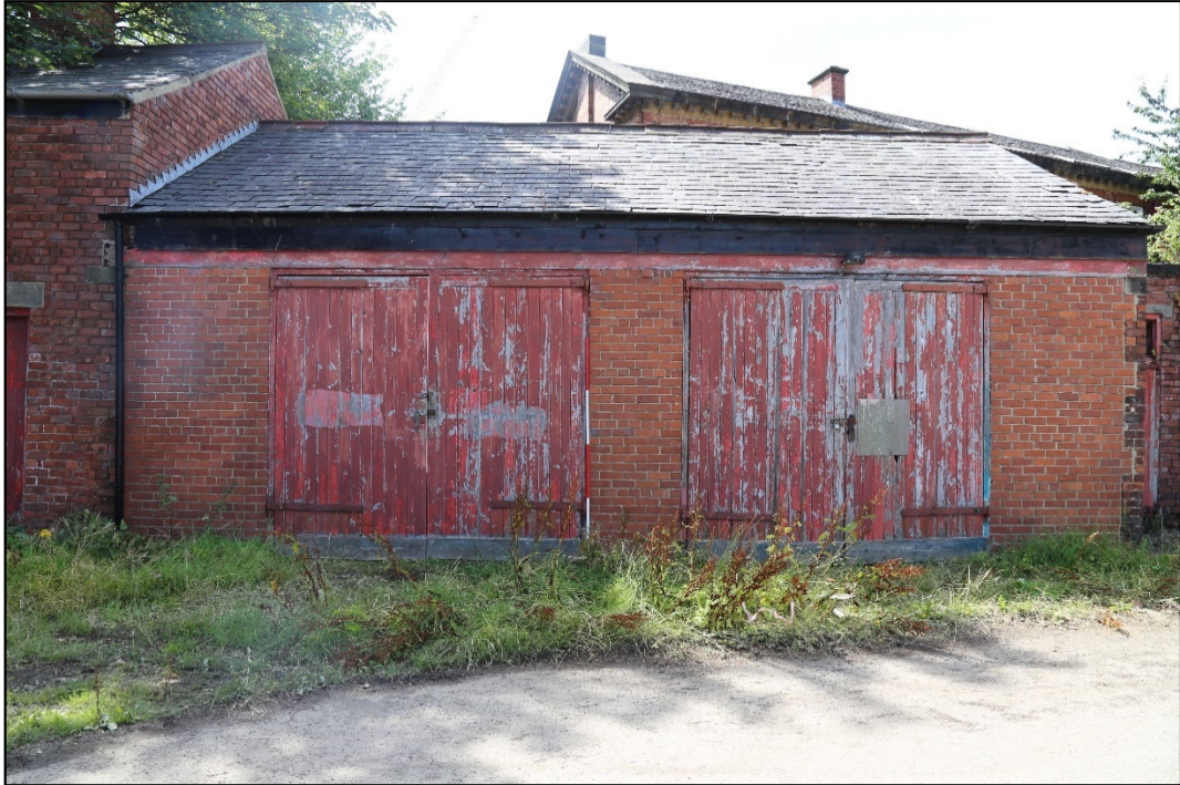
Plate 8: view of the northern elevation of the cart shed showing the two double 'garage' doors (2111).
