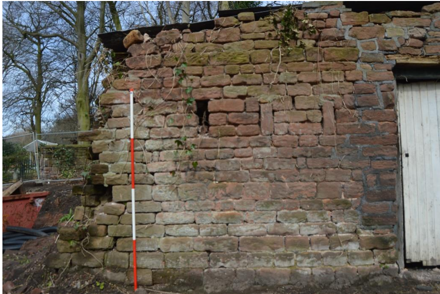
Plate 14: south elevation, west side, showing ventilation slits. View looking north (scale = 2m)
