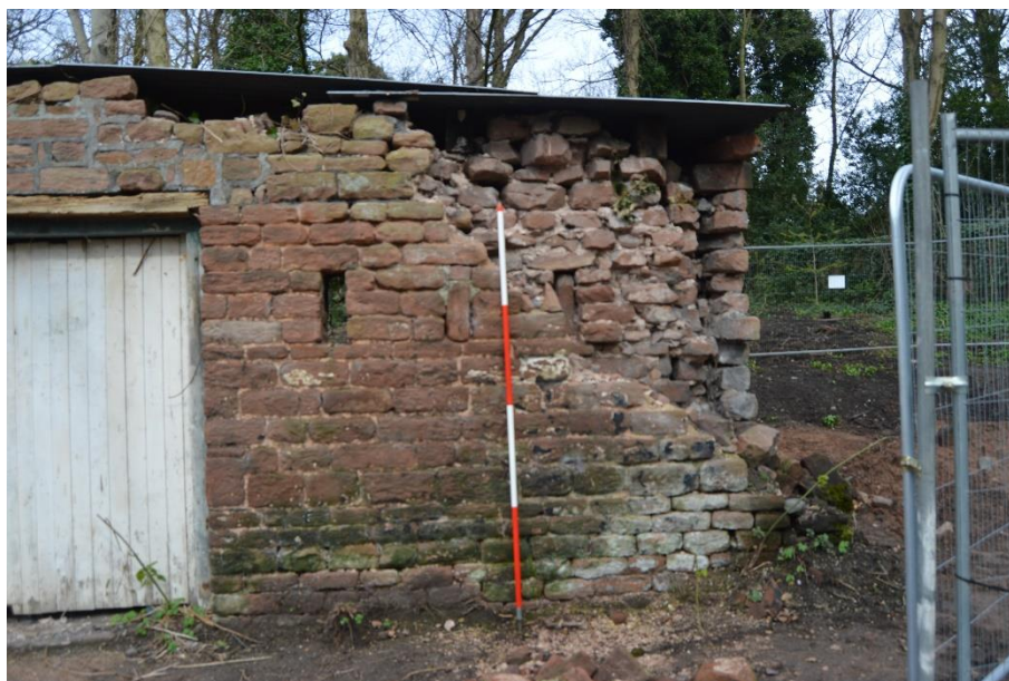
Plate 13: south elevation, east side, showing area of wall collapse. View looking north (scale = 2m)
