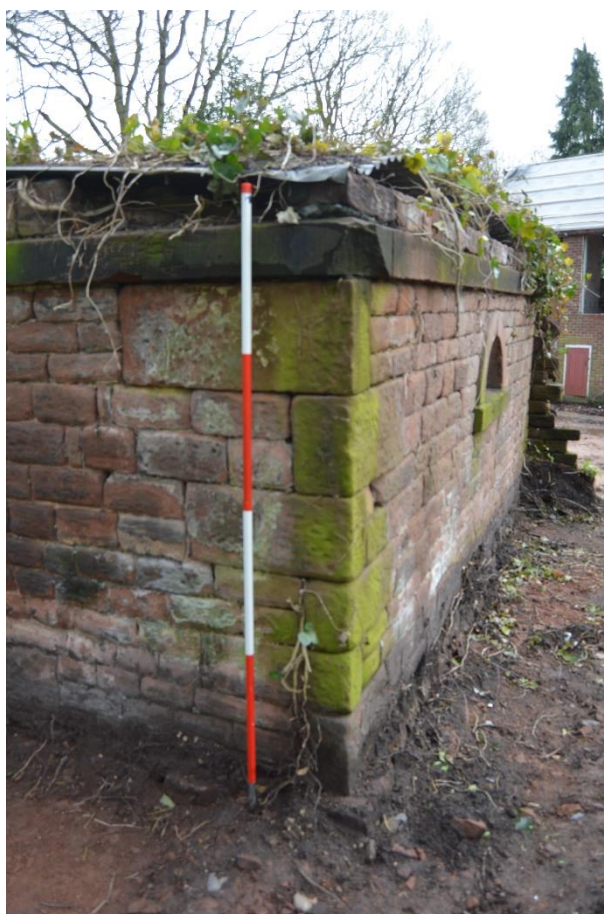
Plate 4: detail of alternating quoins and string course above, north-west corner. View looking south
