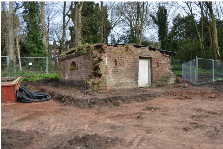
Plate 15: south elevation as seen from the south-west, showing remains of former wall which extended westwards (left of scale). View looking north-east
