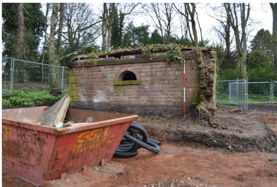
Plate 20: view looking east showing the west elevation and reduced ground level in foreground
