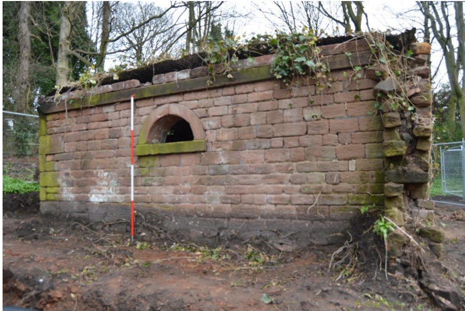
Plate 16: west elevation, with remains of former wall right of photograph. View looking east (scale = 2m)
