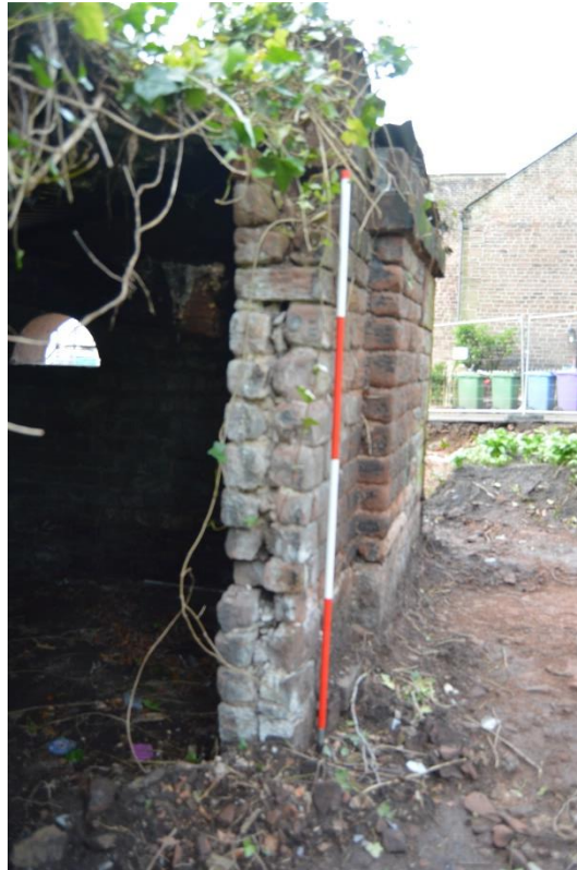
Plate 7: detail of wall thickness (0.3m), doorway in north elevation. View looking west
