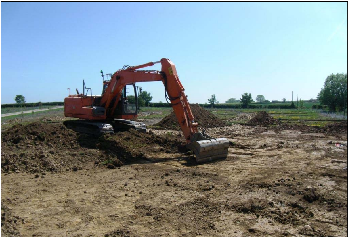
Plate 2: Machine removal of topsoil to the south-west of ASDU Trench 7 (facing east)
