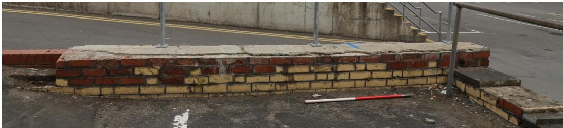
Plate 10: The south, internal elevation D110 of the baths and wash houses looking north.
