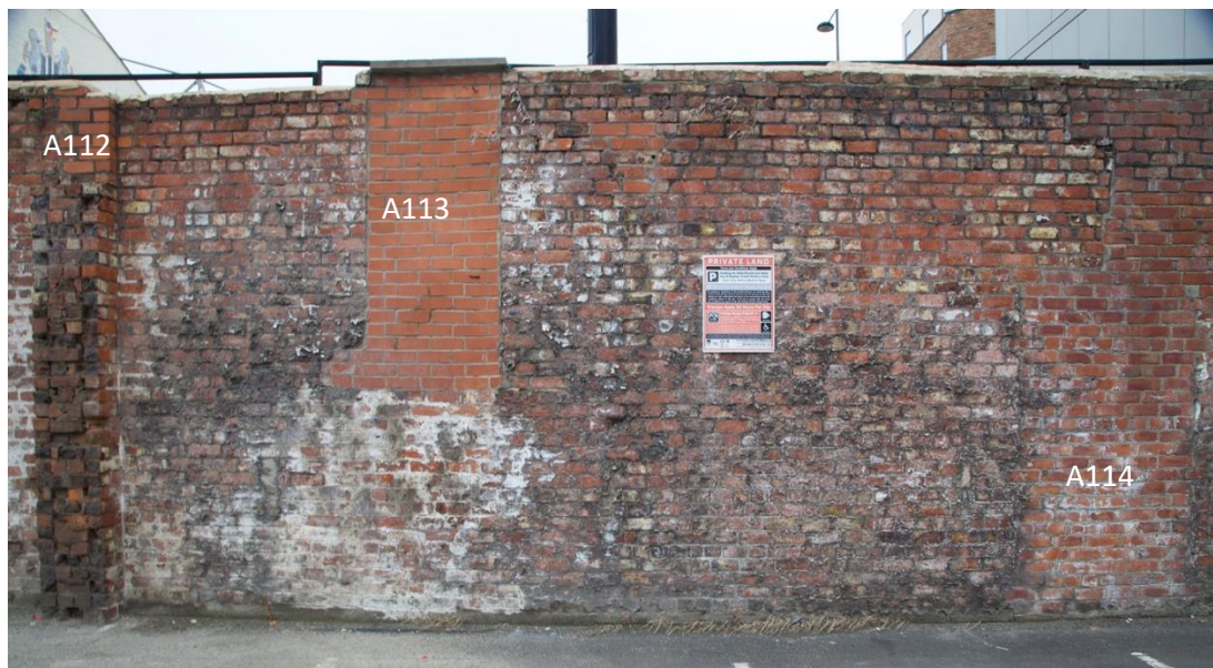
Plate 1: Wall A110 looking north. The wall remains A112 are visible on the left with the blocked door A113 in the centre and the muddled scar A114 on the right.
