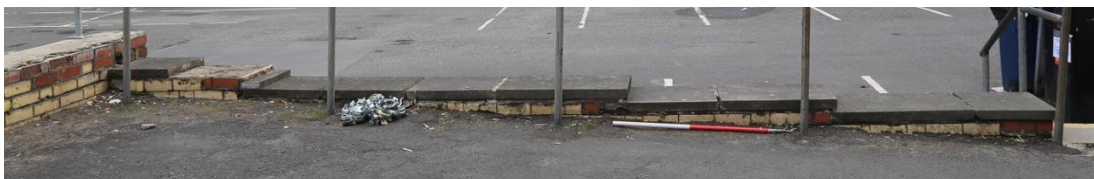
Plate 11: The west, internal elevation 210 of the baths and wash houses looking east.
