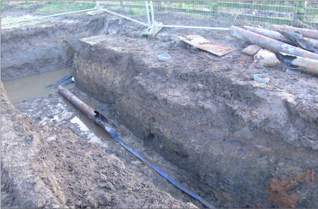
Plate 24: North-facing section of Connector Trench showing continuation of deposits 119, 116, 120 on an oblique north-east to south-west alignment.
