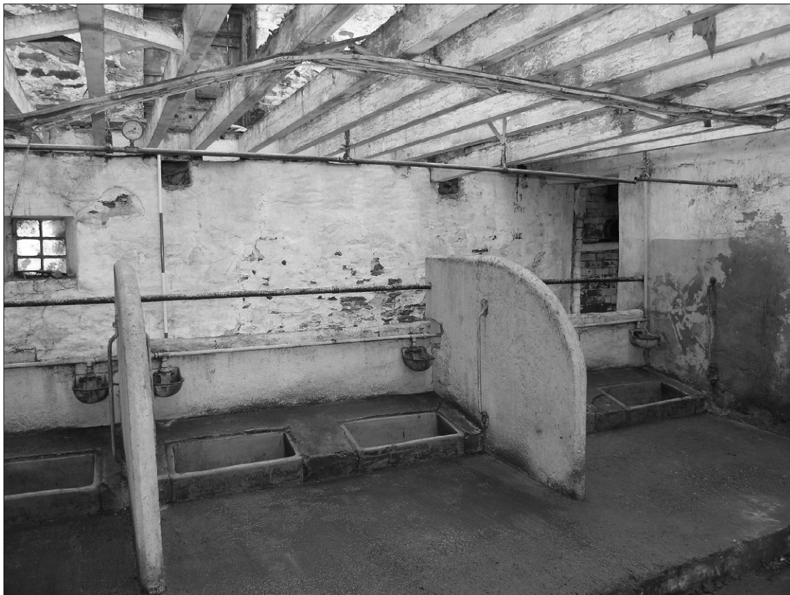
Plate 28 Lane Head Farm South, Capitol Park, Barnsley: cattle stalls in stone barn, looking northeast
