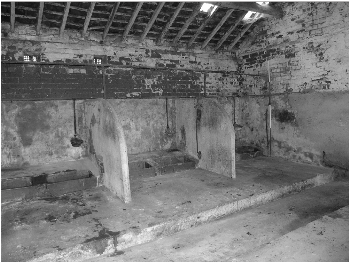
Plate 30 Lane Head Farm South, Capitol Park, Barnsley: cattle stalls in first brick byre, looking northeast
