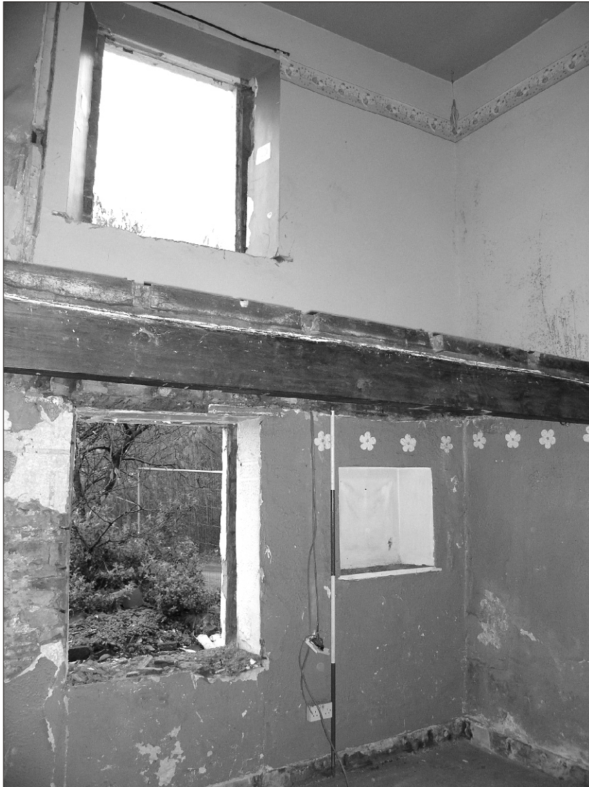
Plate 15 Lane Head Farm South, Capitol Park, Barnsley: ground floor room in western extension, looking southwest. Western window has been blocked to form a cupboard and the former doorway partially blocked to form a window
