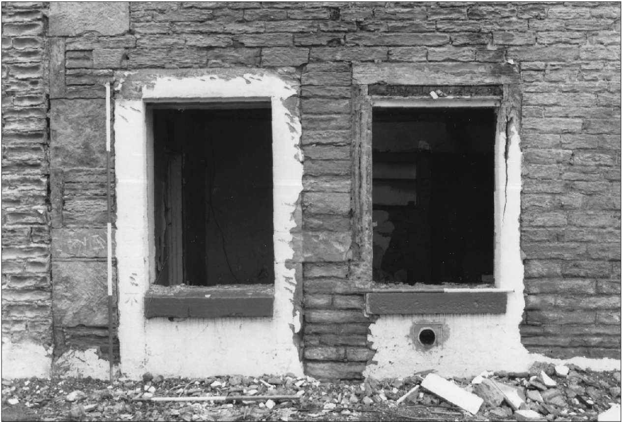
Plate 3 Lane Head Farm South, Capitol Park, Barnsley: original door into the 'cottage' (blocked) and adjacent window
