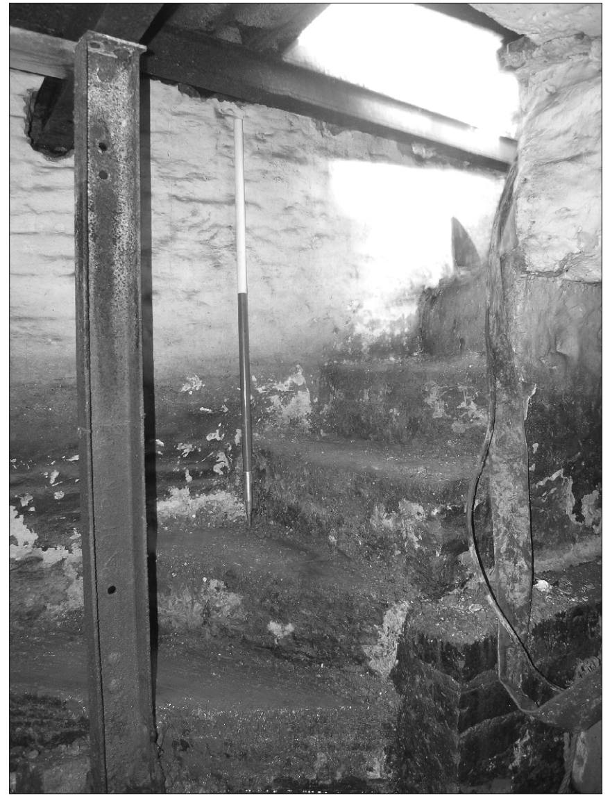
Plate 18 Lane Head Farm South, Capitol Park, Barnsley: stone steps leading down to cellar
