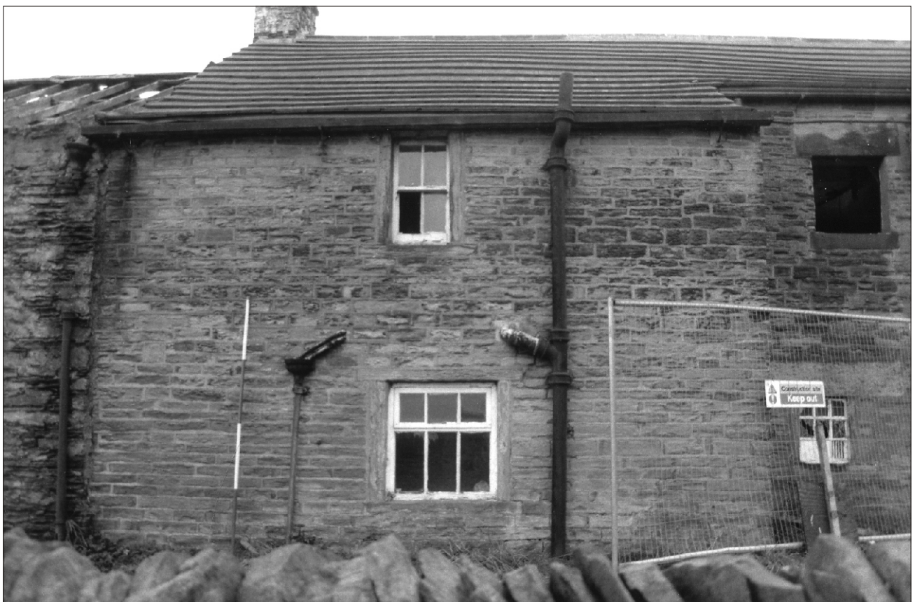
Plate 22 Lane Head Farm South, Capitol Park, Barnsley: north facing elevation of outshot
