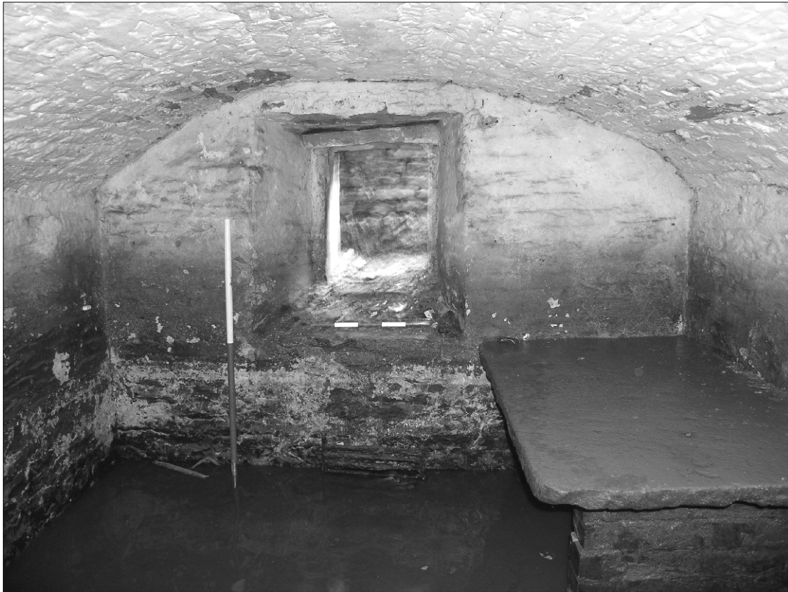
Plate 19 Lane Head Farm South, Capitol Park, Barnsley: view of cellar looking south towards window
