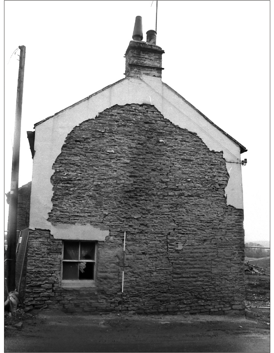
Plate 12 Lane Head Farm South, Capitol Park, Barnsley: western gable end of extension
