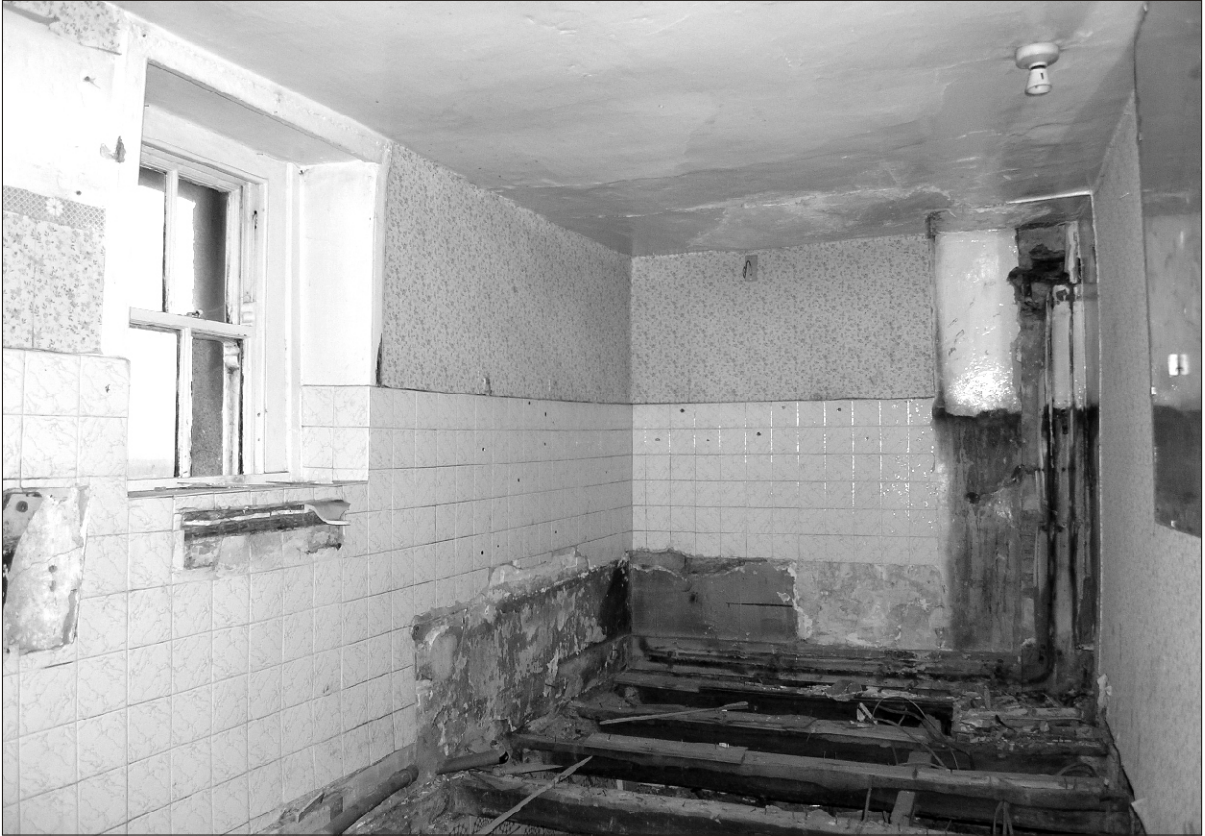
Plate 25 Lane Head Farm South, Capitol Park, Barnsley: first floor room of outshot
