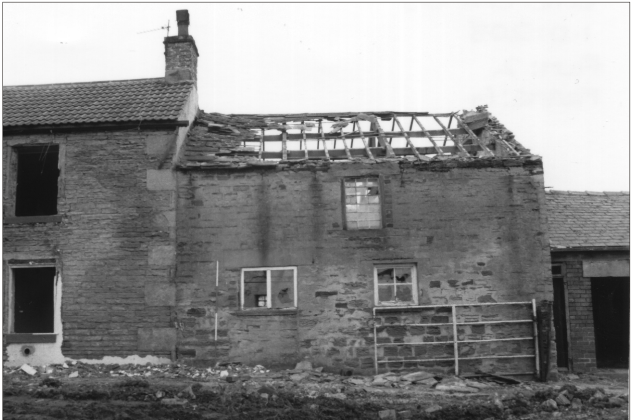
Plate 26 Lane Head Farm South, Capitol Park, Barnsley: south facing elevation of stone barn
