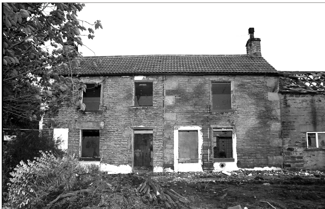
Plate 2 Lane Head Farm South, Capitol Park, Barnsley: main farmhouse after render removed clearly showing 'cottage' and western extension
