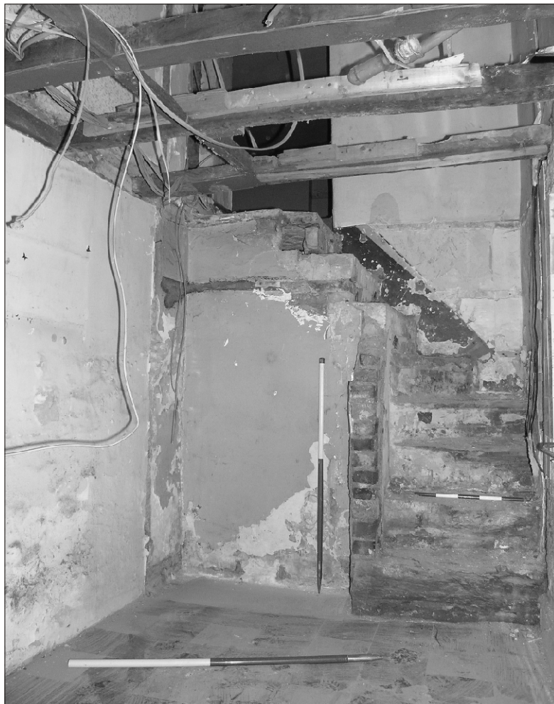
Plate 24 Lane Head Farm South, Capitol Park, Barnsley: staircase to first floor located on west side of outshot
