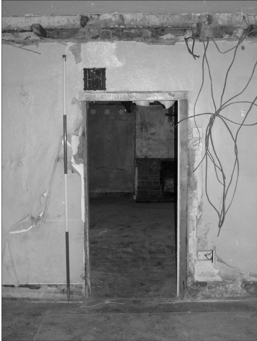
Plate 5 Lane Head Farm South, Capitol Park, Barnsley: connecting door between the 'cottage' and the western extension
