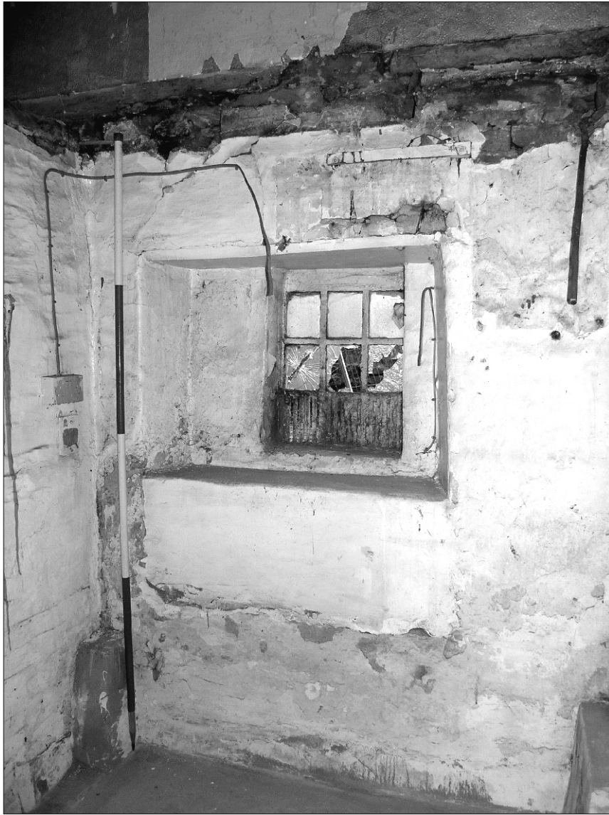
Plate 17 Lane Head Farm South, Capitol Park, Barnsley: north facing window in scullery (partially blocked)
