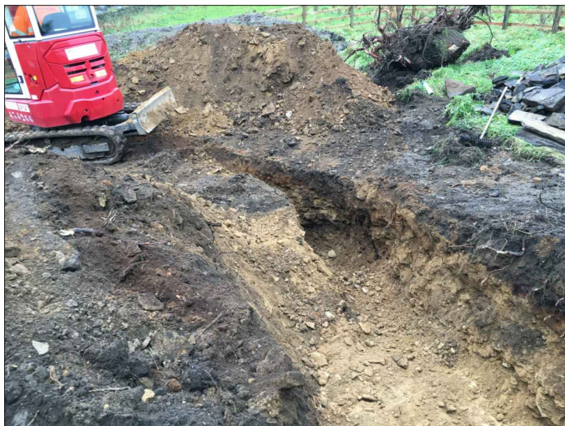
Plate 3: pipe trench in field showing topsoil over natural Ryecroft Road, Hainworth, West Yorkshire: plates
