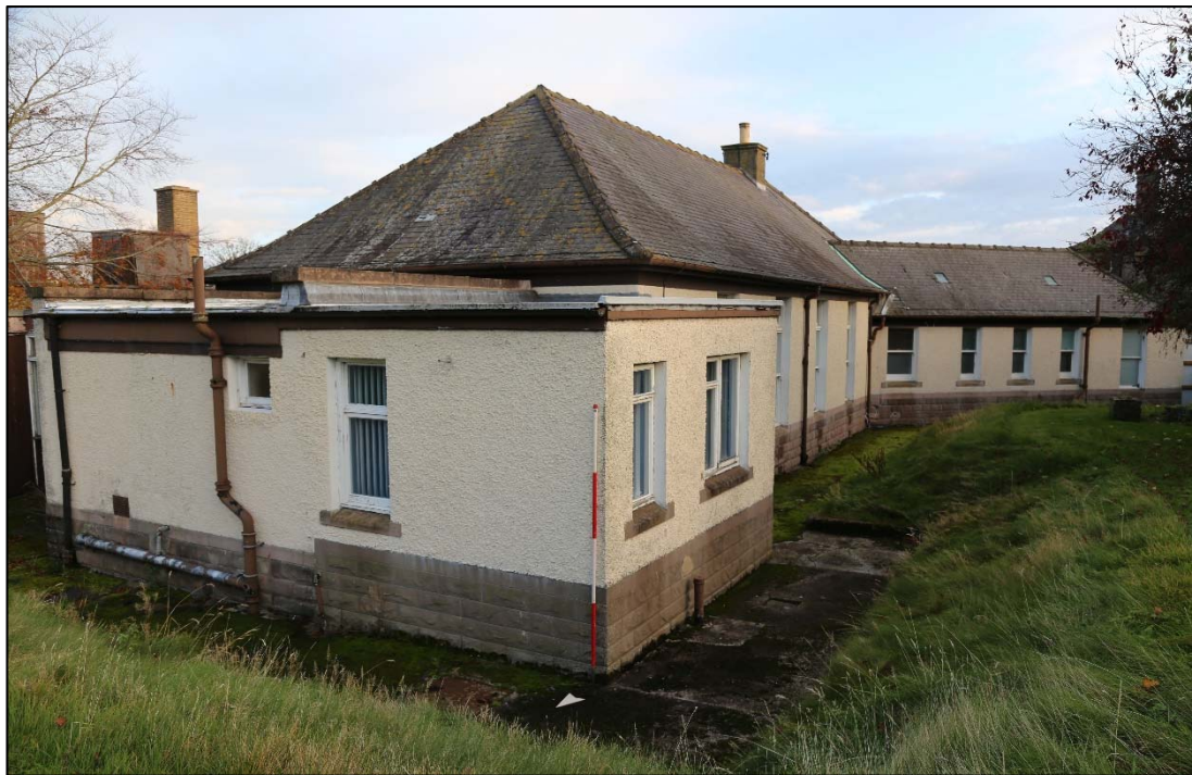
Plate 13: photo looking south, showing the later additions to the Richardson ward in the foreground and the original ward in the background.
