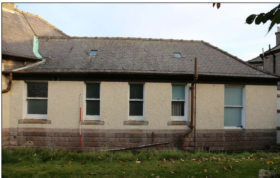
Plate 14: northwest-facing elevation showing examples of original windows within one of the arms of the Jane Richardson Ward – elevation 1120.
