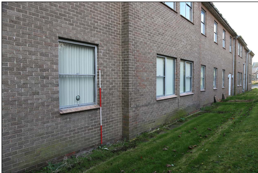
Plate 34: north-facing elevation 4200, showing some of the recessed areas and some of the windows.
