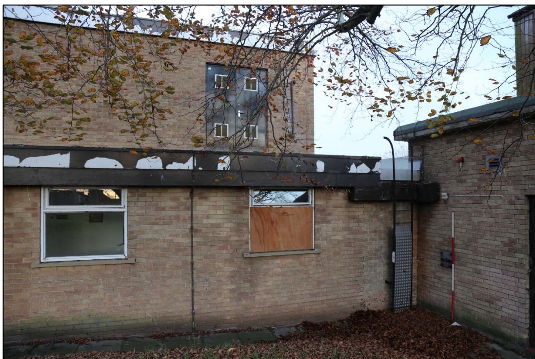
Plate 28: the east end of the operating theatre building showing its full height (2400), and the single-storey corridor (2001), the vacuum-plant room (2500) can be seen to the right.
