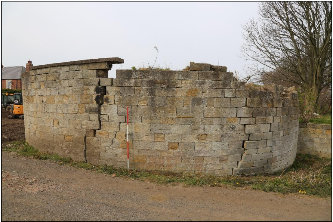
Plate 4: east side of the south-west bastion, looking north-west, showing large vertical cracks and a bulge on the right-hand side.
