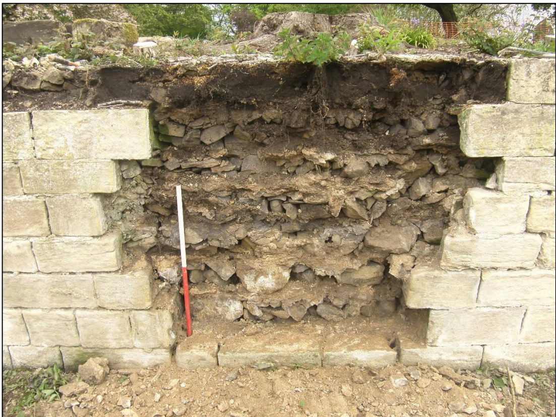
Plate 31: Section 6 of the west ha-ha after the removal of the ashlar facing.
