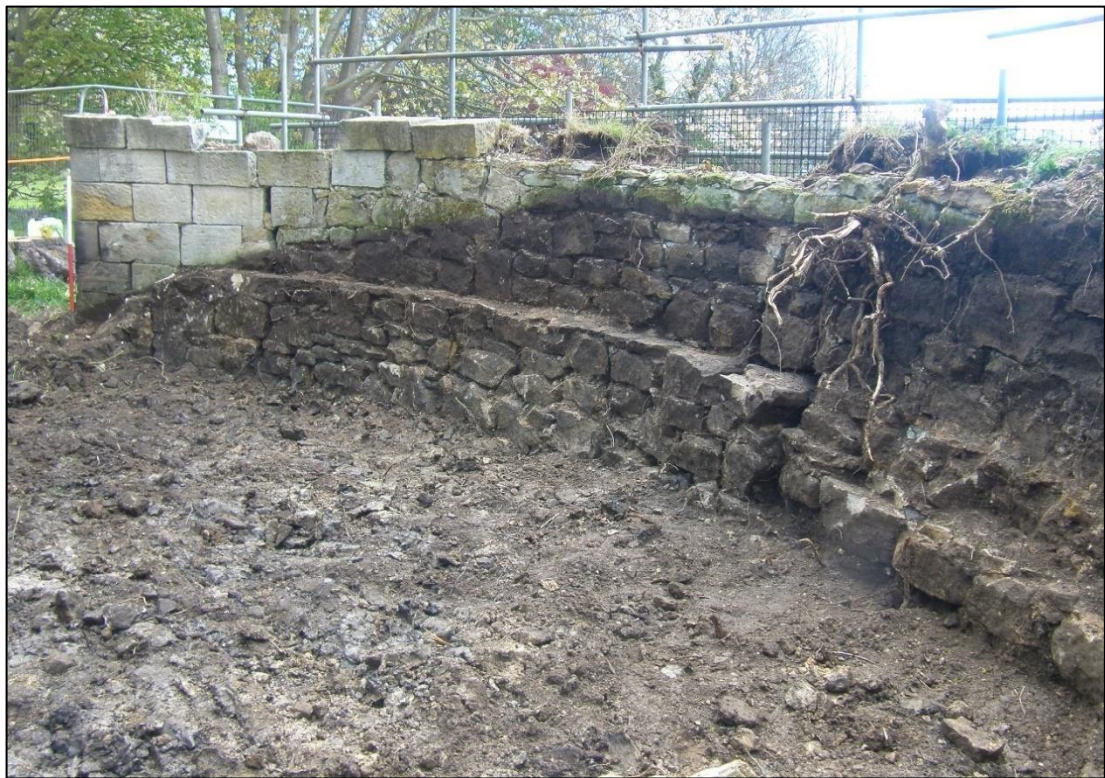
Plate 11: internal elevation of the east side of the south-west bastion, showing partially exposed foundation step, mid-section, and upper ashlar courses. The original level of the internal deposits is denoted by the dark staining.
