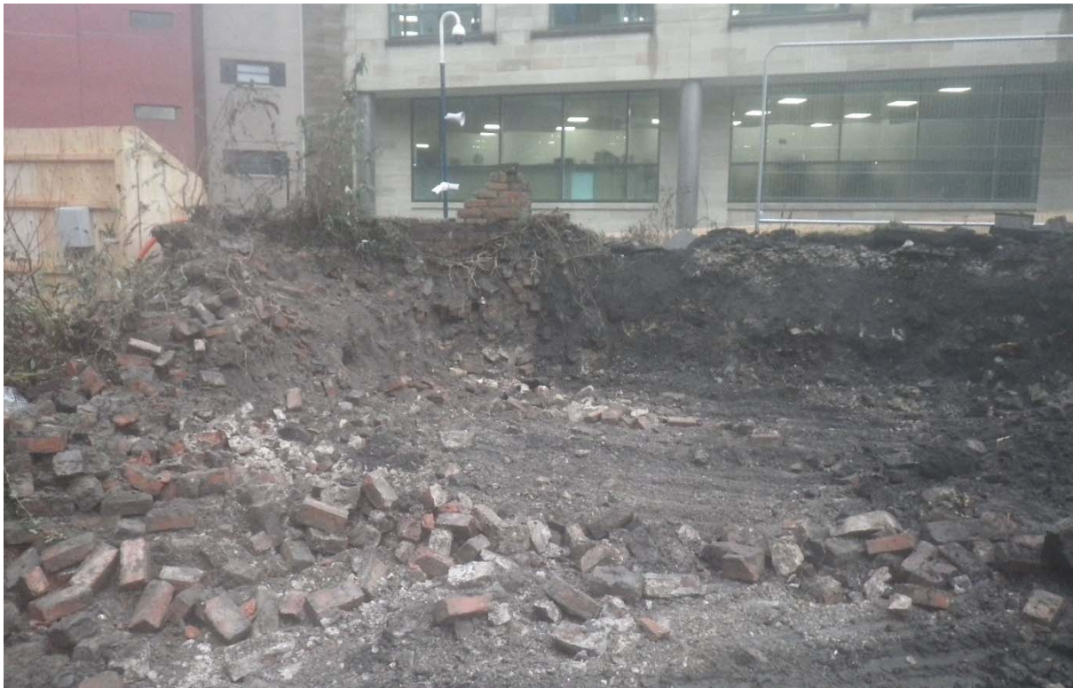
Plate 7: demolition of the 19th-century midden and removal of the modern earth bank in the southeast on the development.
