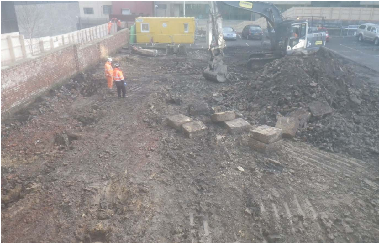
Plate 5: natural boulder clay beneath the concrete yard surface, with stone pillar supports for the sawmill during removal.
