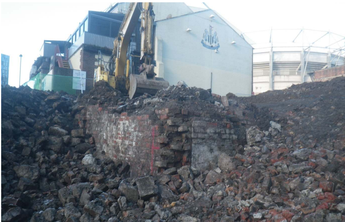
Plate 1: brick retaining wall for 19th-century properties to the east of The Strawberry in Plot A.
