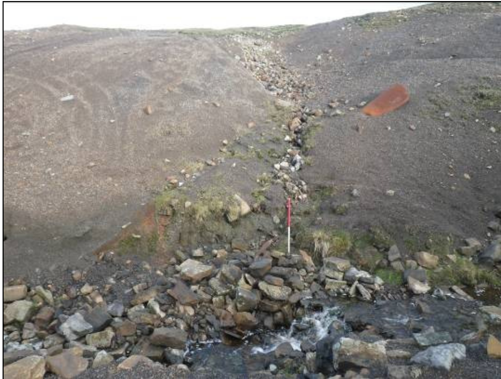
Plate 60: Water runoff from quarry track with collapsed section of culvert in foreground. Note large quantities of material behind remains of culvert wall.
