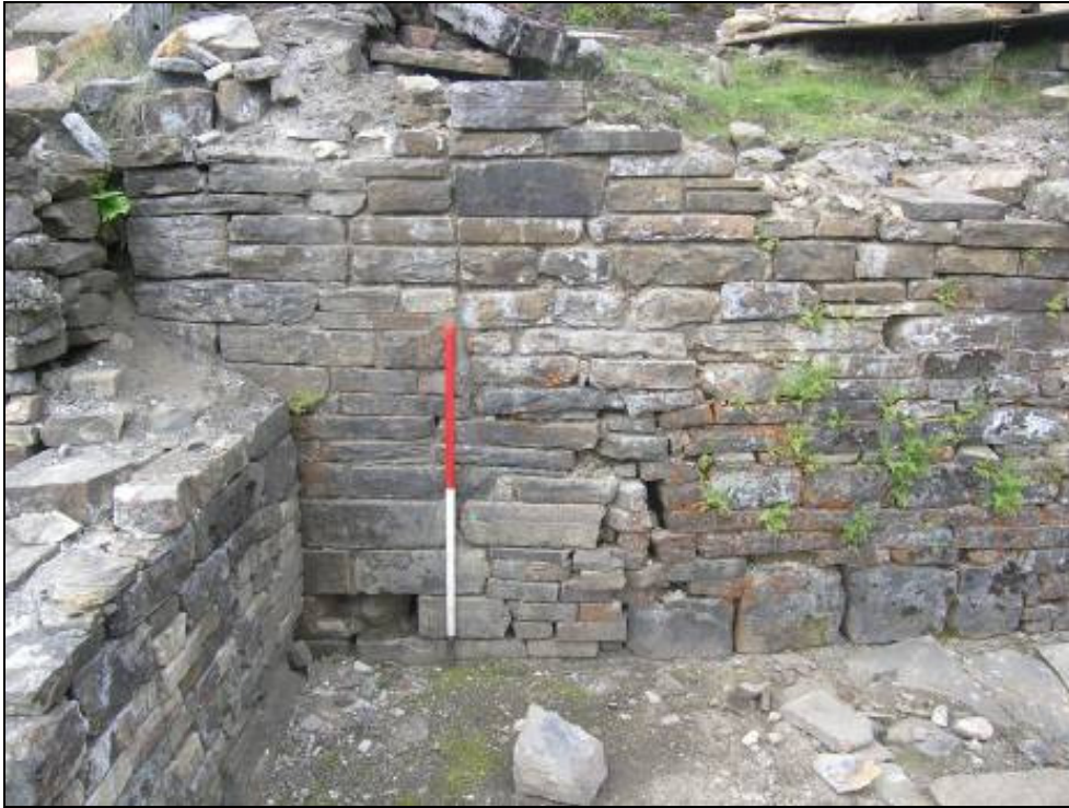
Plate 8: Smelt Mill Feature 5. Note two voids either side of ranging pole. Wall of Building A butting against.
