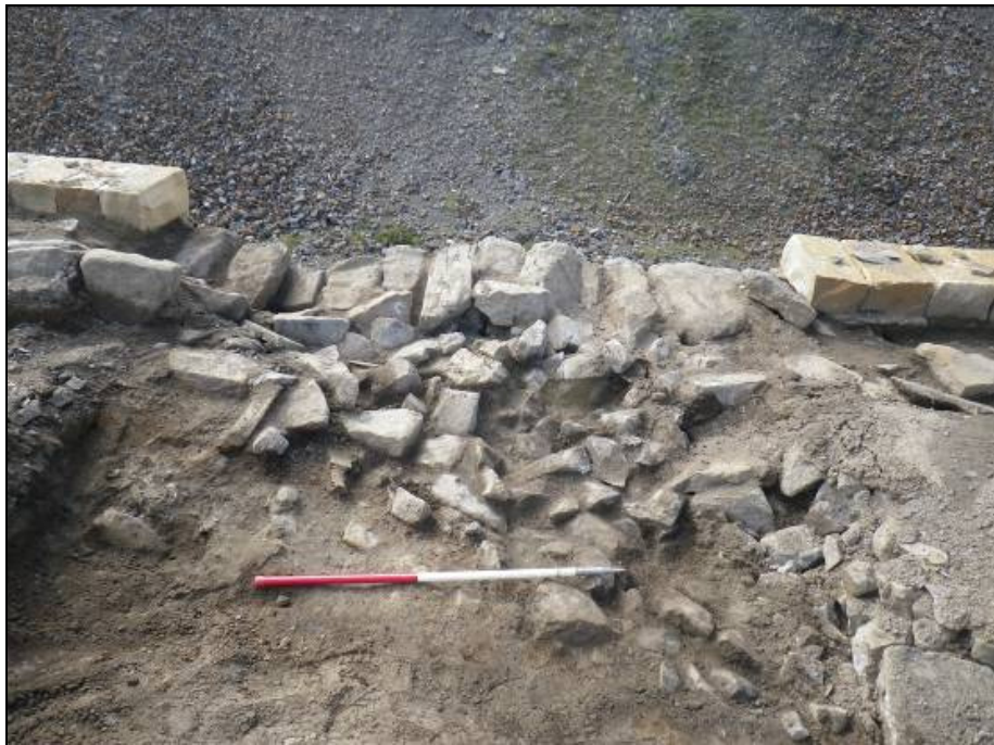
Plate 71: Large deposit of limestone blocks used to repair edge of dressing floor.
