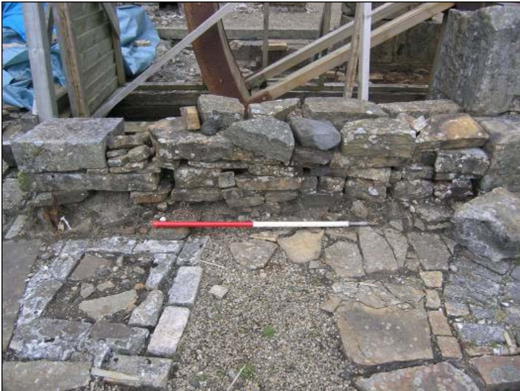
Plate 1: Smelt Mill Feature 1 pre-intervention image of section of wall to be dismantled and rebuilt.
