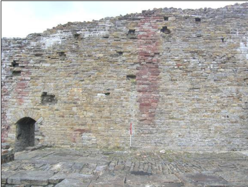
Plate 30: Spine Wall Feature 2 pre-intervention.
