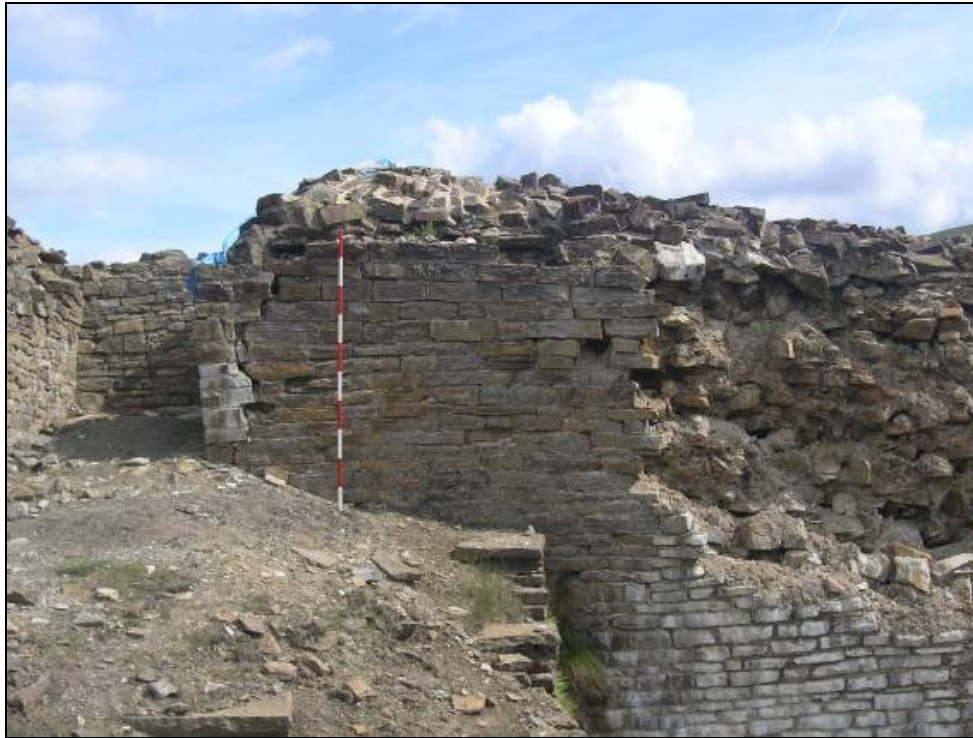
Plate 29: Spine Wall Feature 1 pre-intervention.
