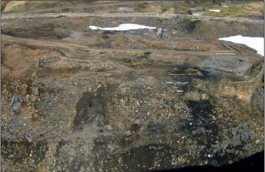
Plate 65: Section of retaining wall to left of image pre-consolidation. Note consolidated retaining wall to the right of the image.
