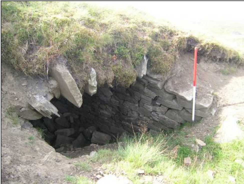
Plate 51: Flue 06 downhill portal showing areas of subsistence.
