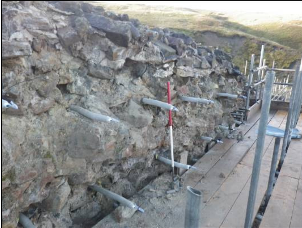
Plate 45: Section of spine wall facing northwest showing series of anchor holes.
