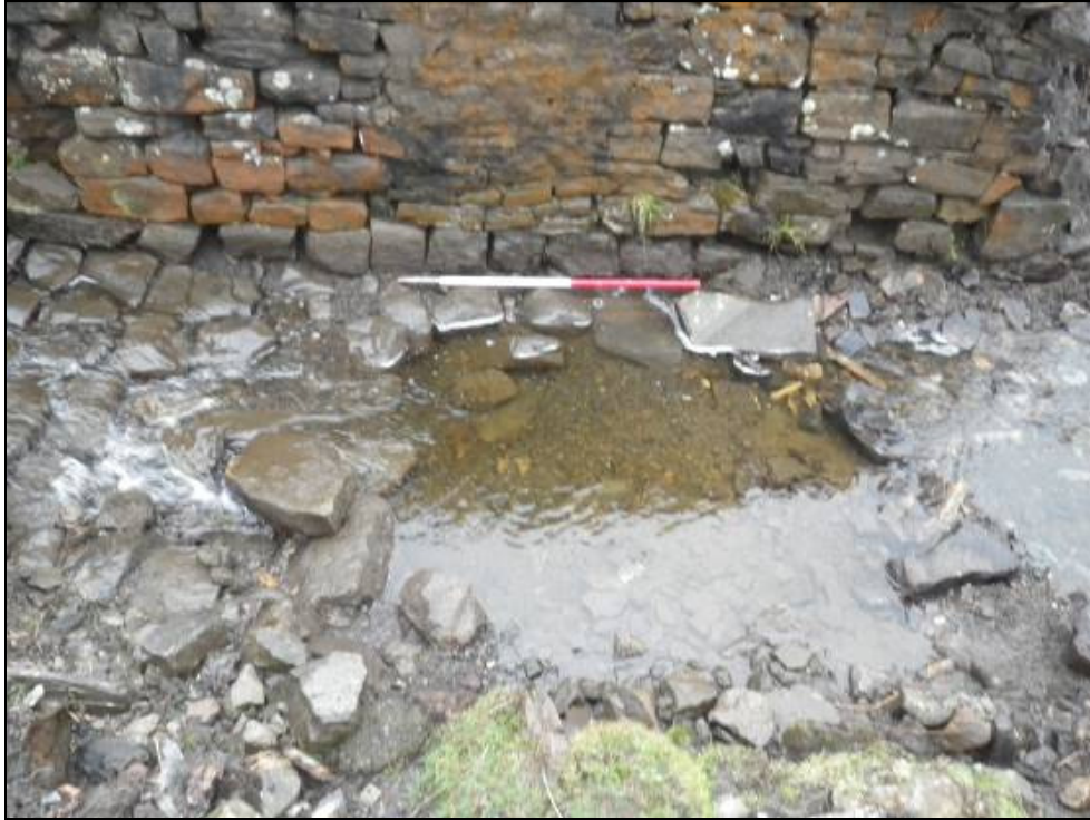
Plate 61: Section of washed out cobbled base with washed out wall footing at bottom of image.
