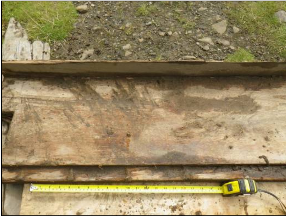
Plate 68: Radiating scratch marks at base of chute at side intake.
