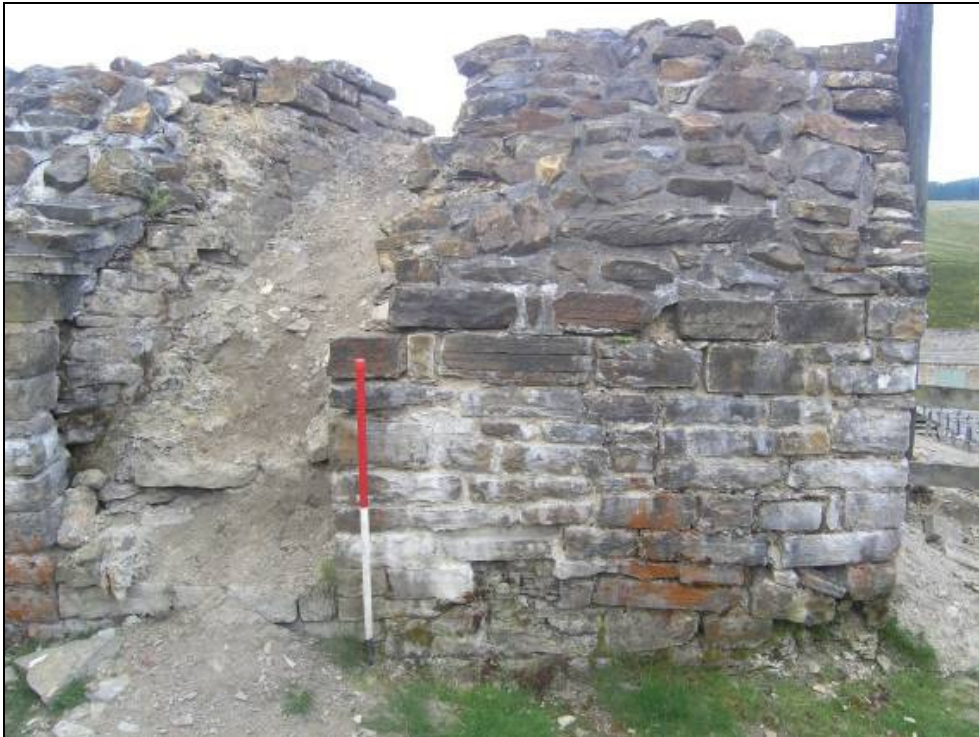
Plate 31: Spine Wall Feature 3 pre-intervention.
