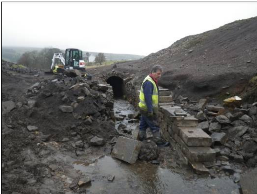
Plate 62: Photograph taken during rebuilding of collapsed wall. Machined section to the left of the image.
