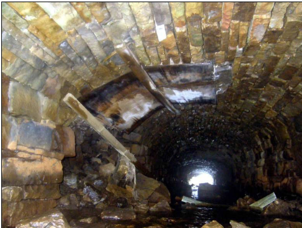
Plate 52: Collapsed voussoirs and side walls with previous NPHT repair above.
