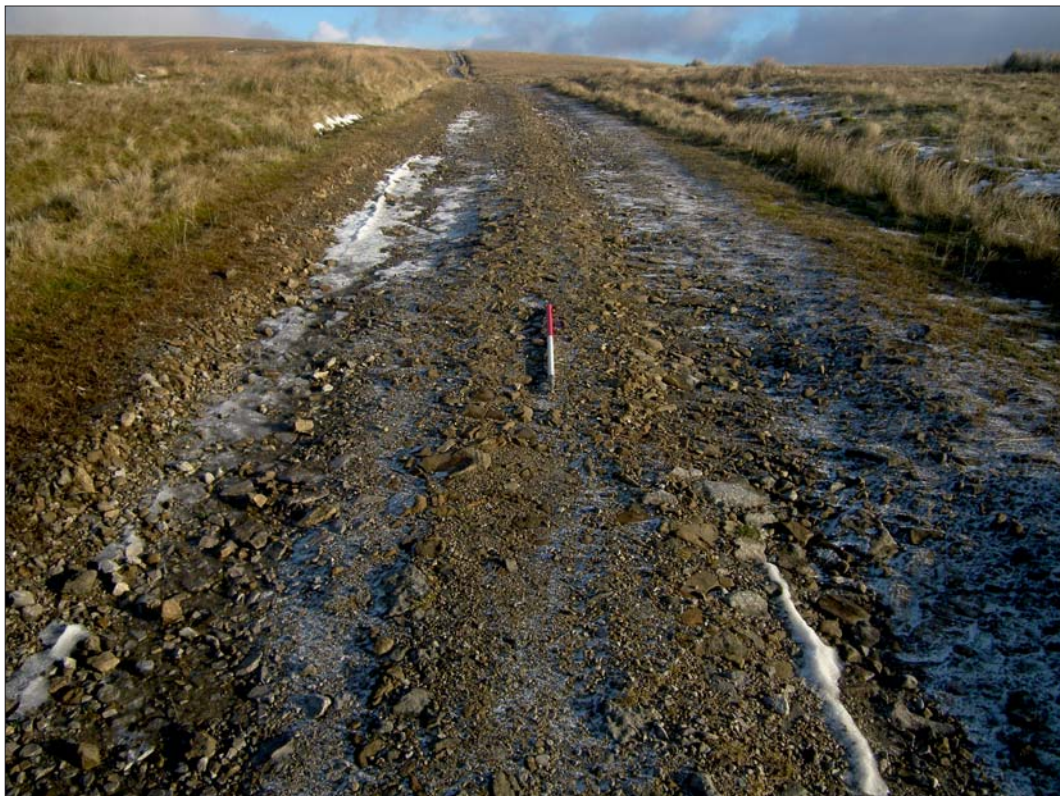
Cam High Road, Yorkshire Dales National Park: Dales Way - example of existing track surface and side ditches Plate 6
