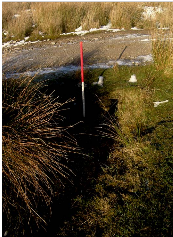
Cam High Road, Yorkshire Dales Plate 10 National Park: Dales Way - example of intact culvert
