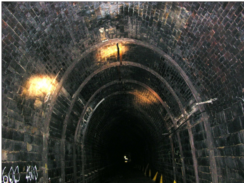
Plate 8 Woodhead Tunnel: General view of railway period steel and timber reinforcement of lined section of South Bore
