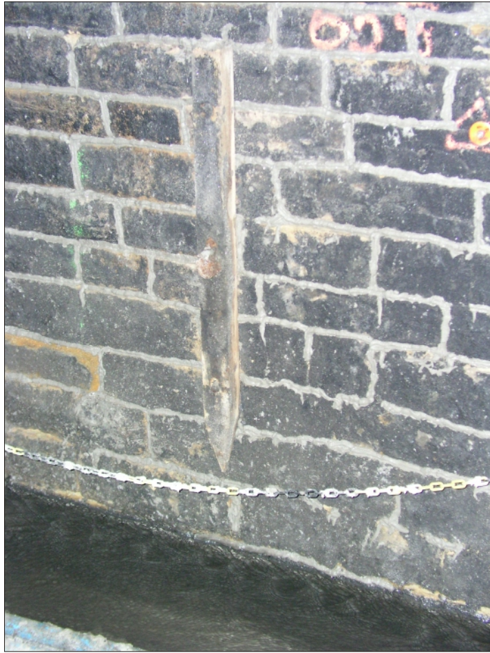
Plate 7 Woodhead Tunnel: Example of a short wooden post with wire pulley attached
