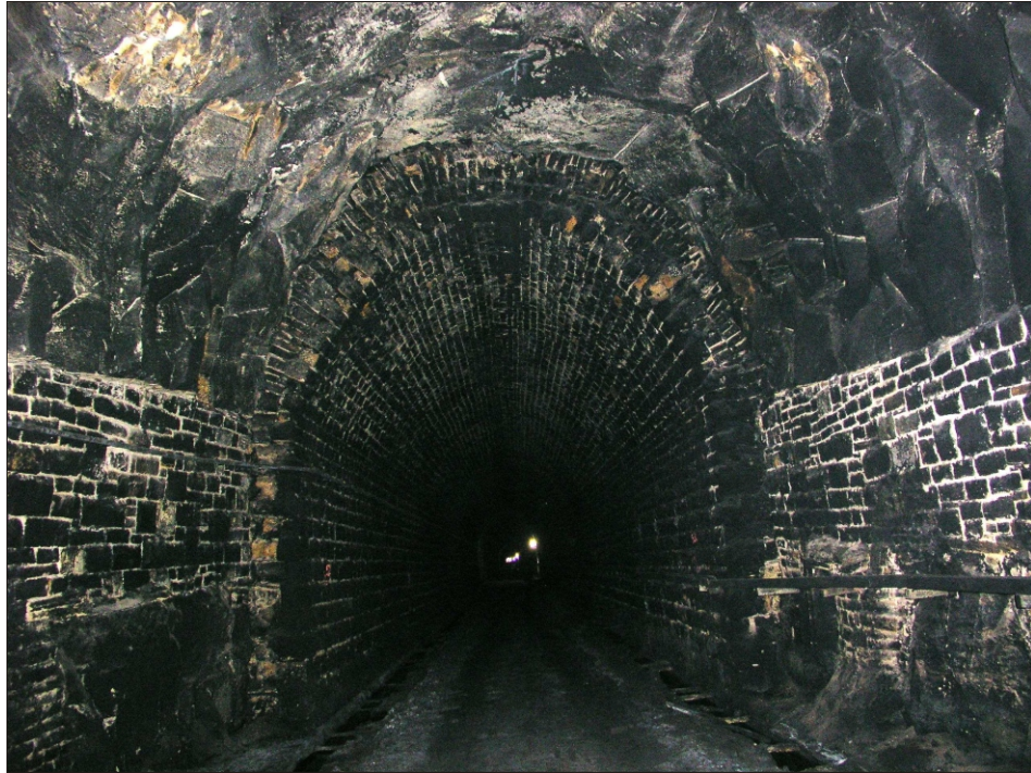
Plate 3 Woodhead Tunnel: Example of junction between lined and unlined section of South Bore
