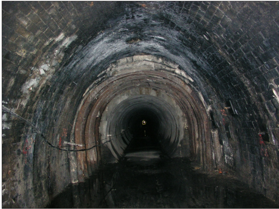
Plate 5 Woodhead Tunnel: Example where successive phases of reinforcement has narrowed the South Bore
