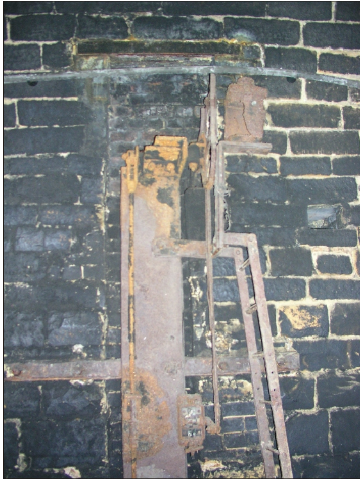
Plate 11 Woodhead Tunnel: Detail of signal lamp showing infilled cavity behind suggesting that apparatus was secondary in this position
