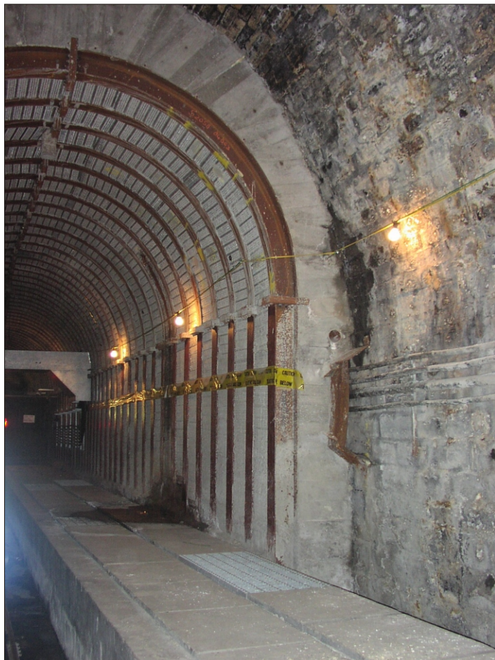
Plate 2 Woodhead Tunnel: Concrete and steel reinforcement to North Bore with cable conduit in foreground
