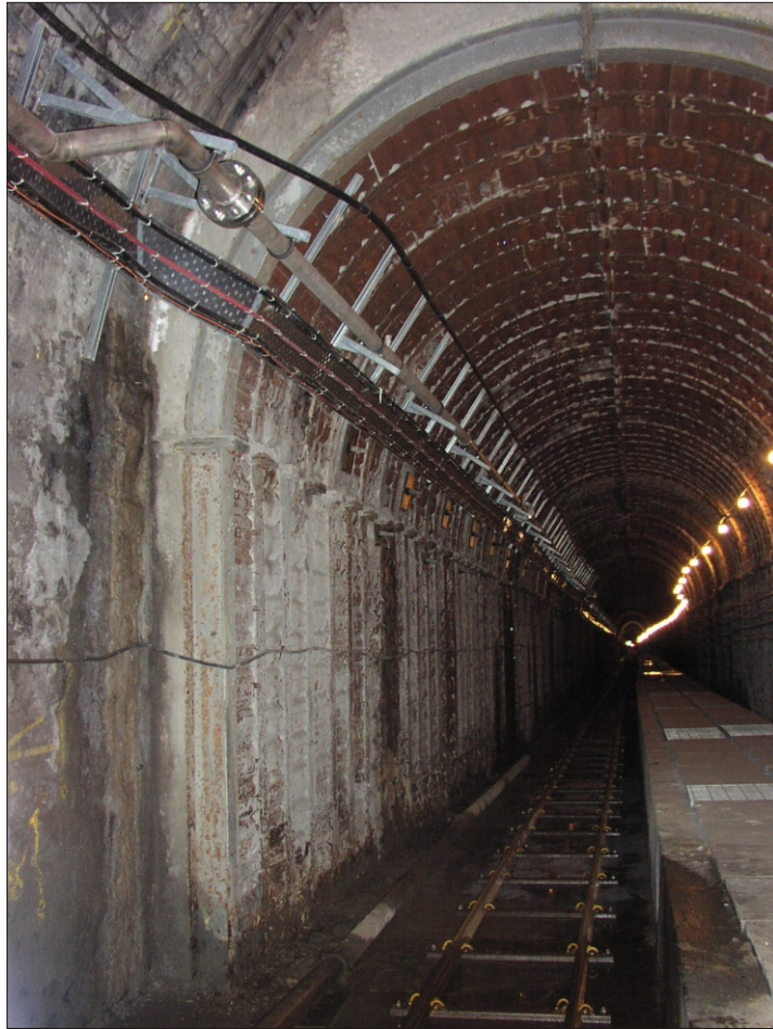
Plate 1 Woodhead Tunnel: Concrete and steel reinforcement to North Bore with access railway in foreground and cable conduit to right
