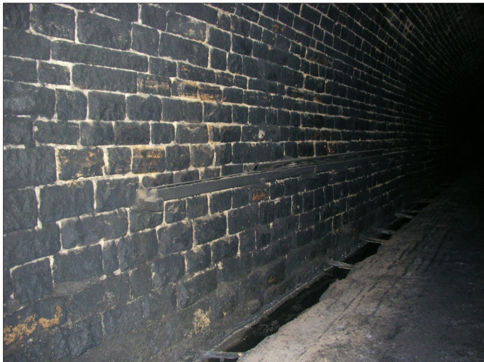
Plate 6 Woodhead Tunnel: Section of the wooden cable trunking and detail of timber lined drain below
