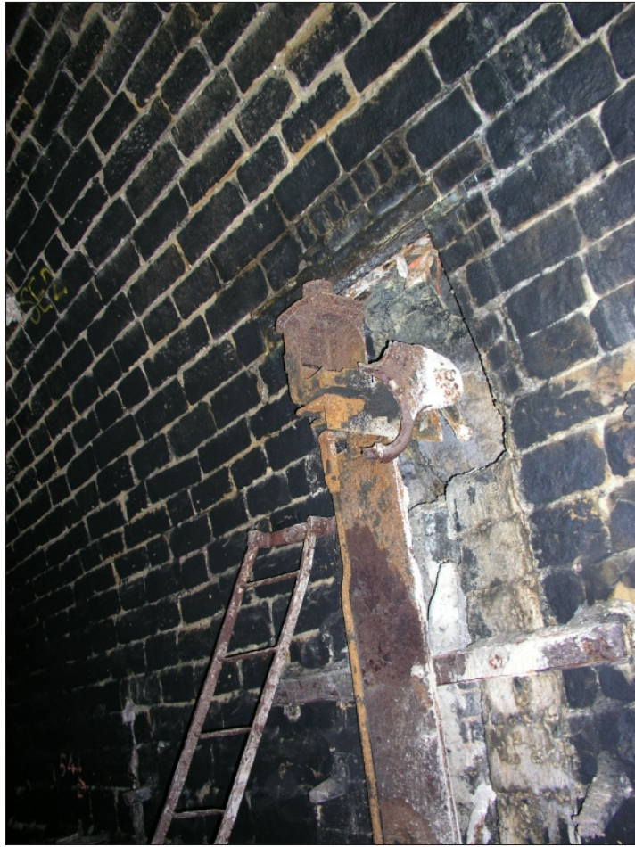
Plate 13 Woodhead Tunnel: Detail of signal lamp showing similar infilled cavity behind suggesting that apparatus was also secondary in this position
