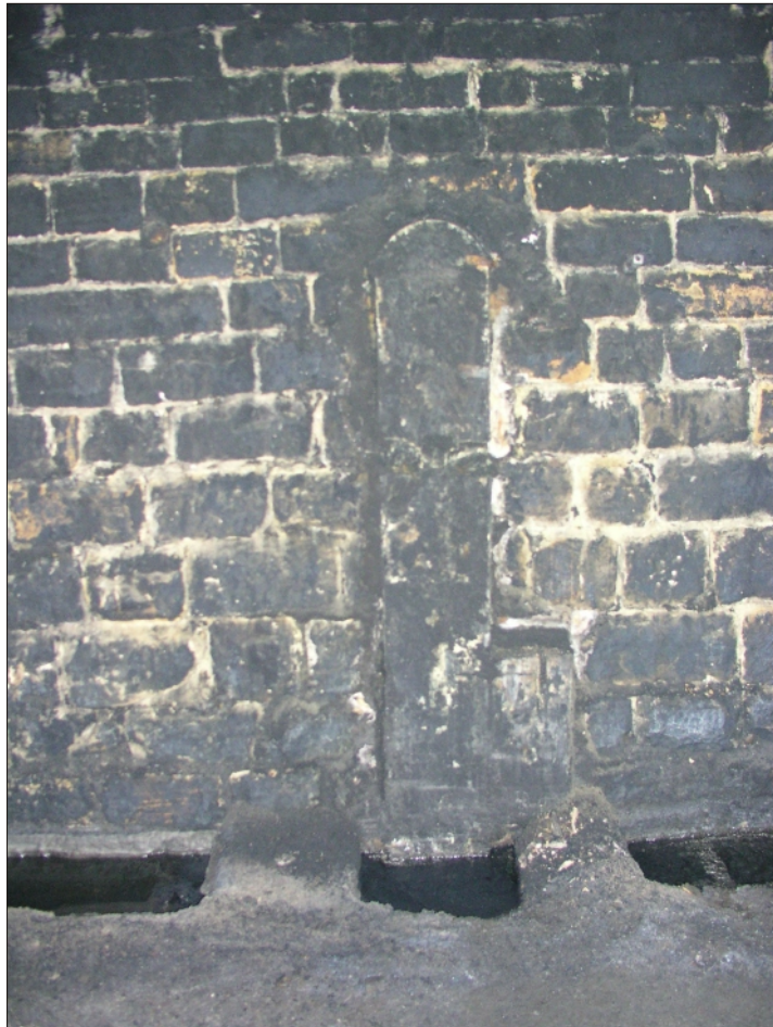
Plate 14 Woodhead Tunnel: Tall shallow recess in stone lining possibly for an earlier signal
