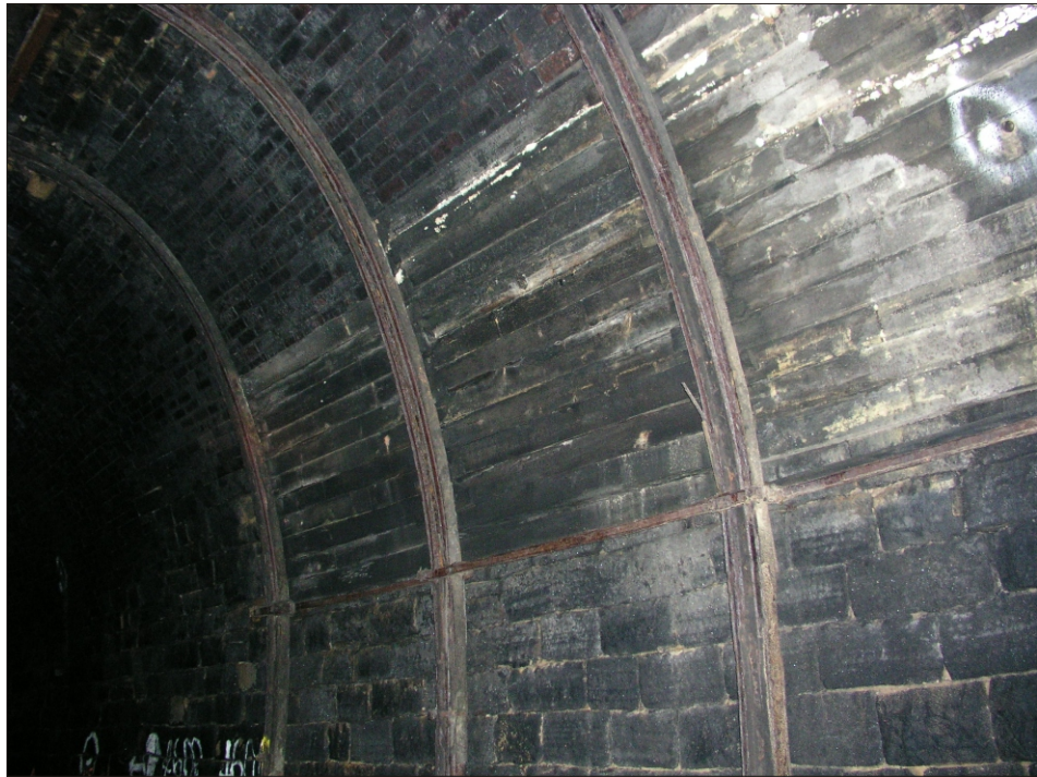
Plate 9 Woodhead Tunnel: Detail of steel and timber reinforcement comprising arched sections of rail and partial timber shuttering
