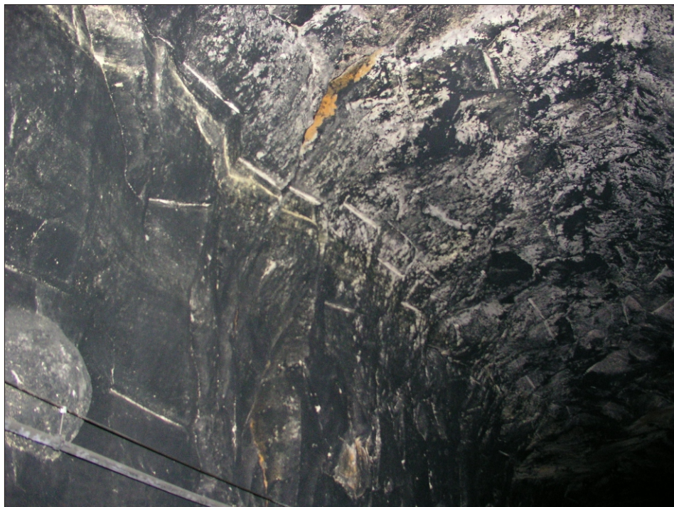
Plate 4 Woodhead Tunnel: Linear drill marks on the rock cut roof and side wall
