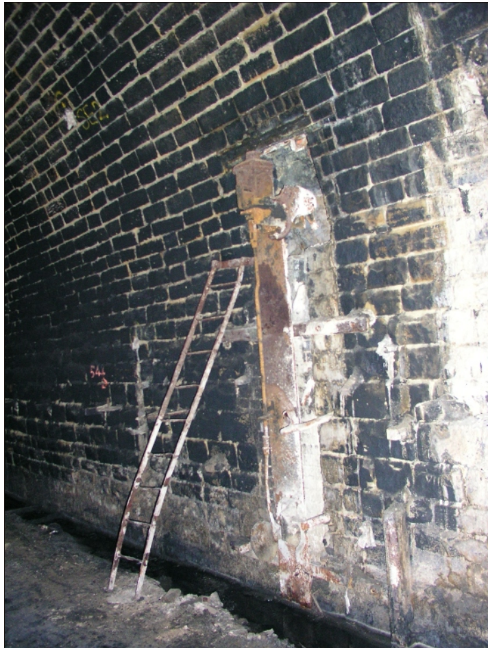
Plate 12 Woodhead Tunnel: Signal Lamp (20th century) and access ladder on north side of South Bore. Lamp faces east
