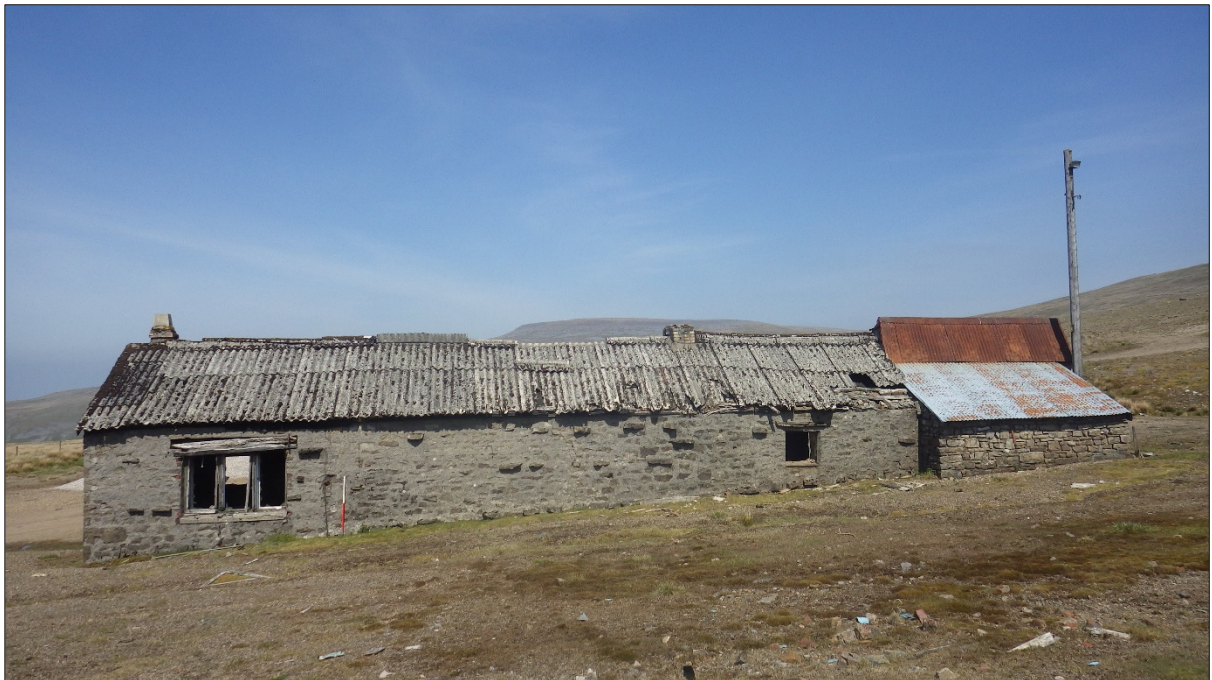
Plate 14: The mine shop, facing west; the building shows multiple phases of construction
