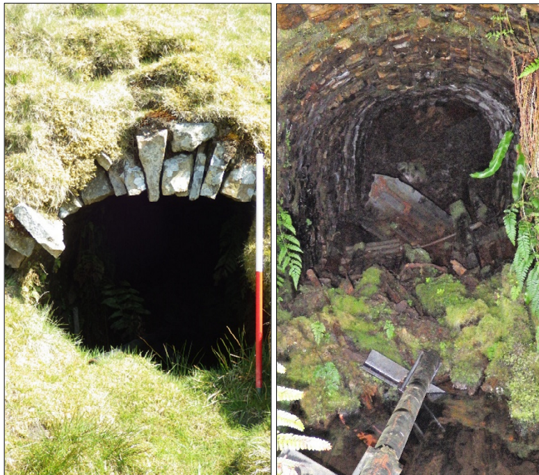
Plate 16: The Low Level, facing north-east; the picture on the right shows the blockage
