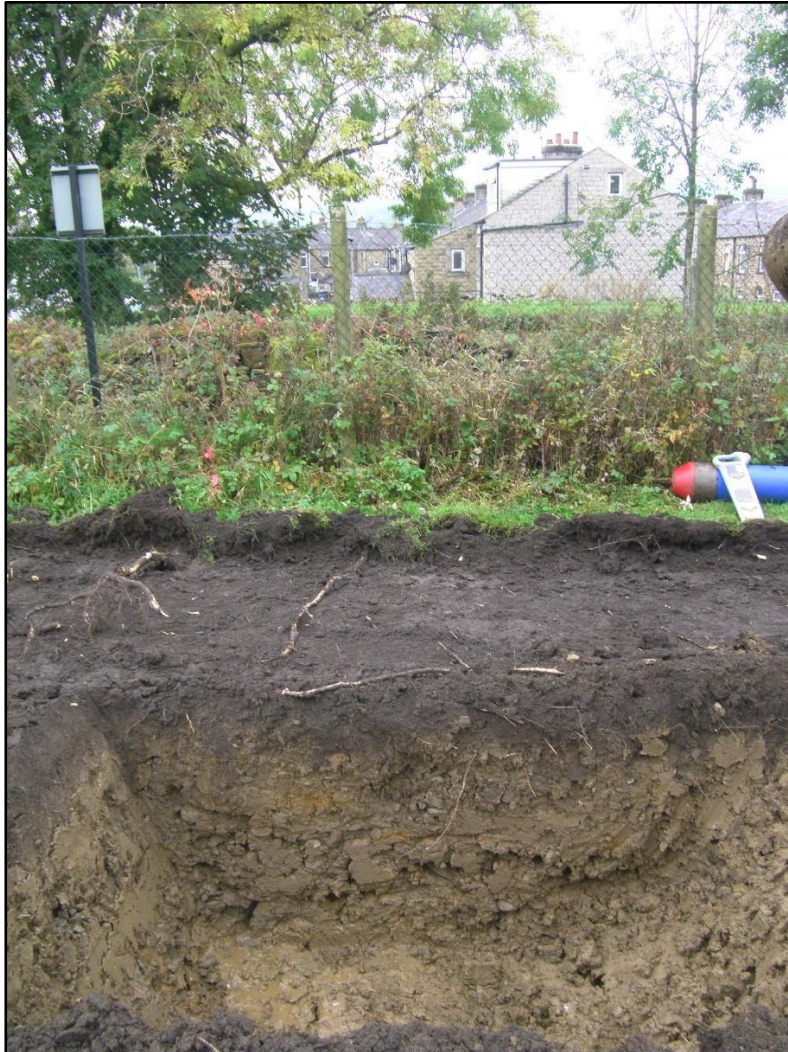
Plate 2: Reception Pit 1 showing accumulation of topsoil and subsoil. Looking south across the Leeds and Liverpool Canal towards the launch pit on Greenfield Street.
