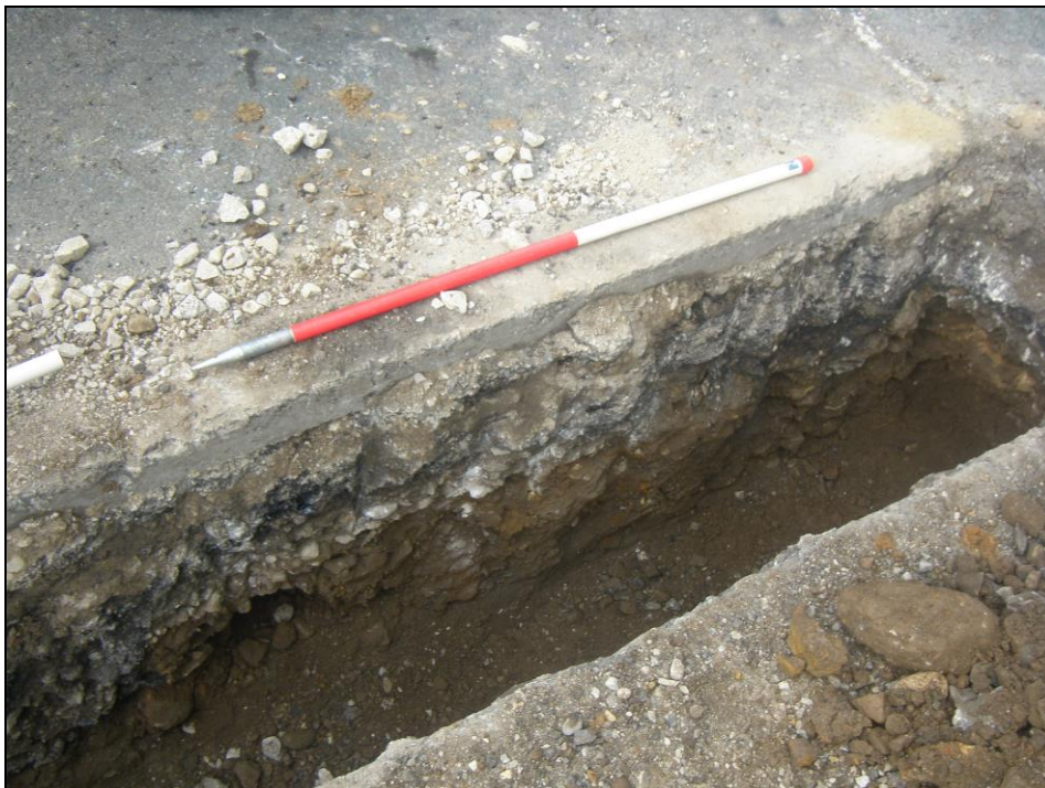
Plate 4. East facing section of Trench 3, cut through the south-west bound carriageway of Bowes Road (A67).
