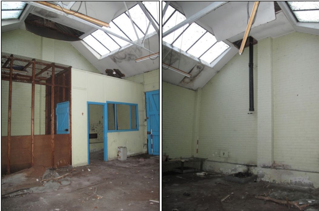
Plate 11: the office space inside Building 4, looking south-east (left), and the western wall of Building 4, showing the former position of a stove and blocked vents (right)
