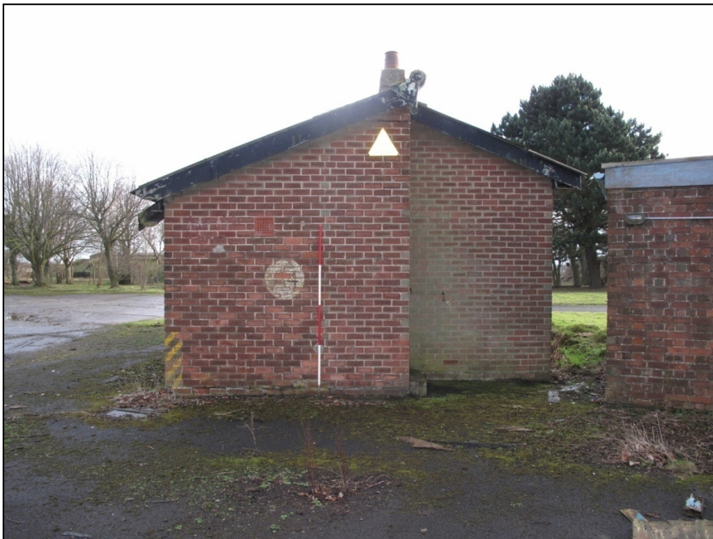
Plate 54: the north-western elevation, showing the asymmetrical roof slopes. Building 19 can be seen to the right
