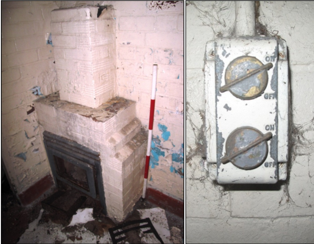
Plate 63: the stove on the southern wall, showing the small dividing wall to the east (left), and a covered switch inside Building 19 (right)
