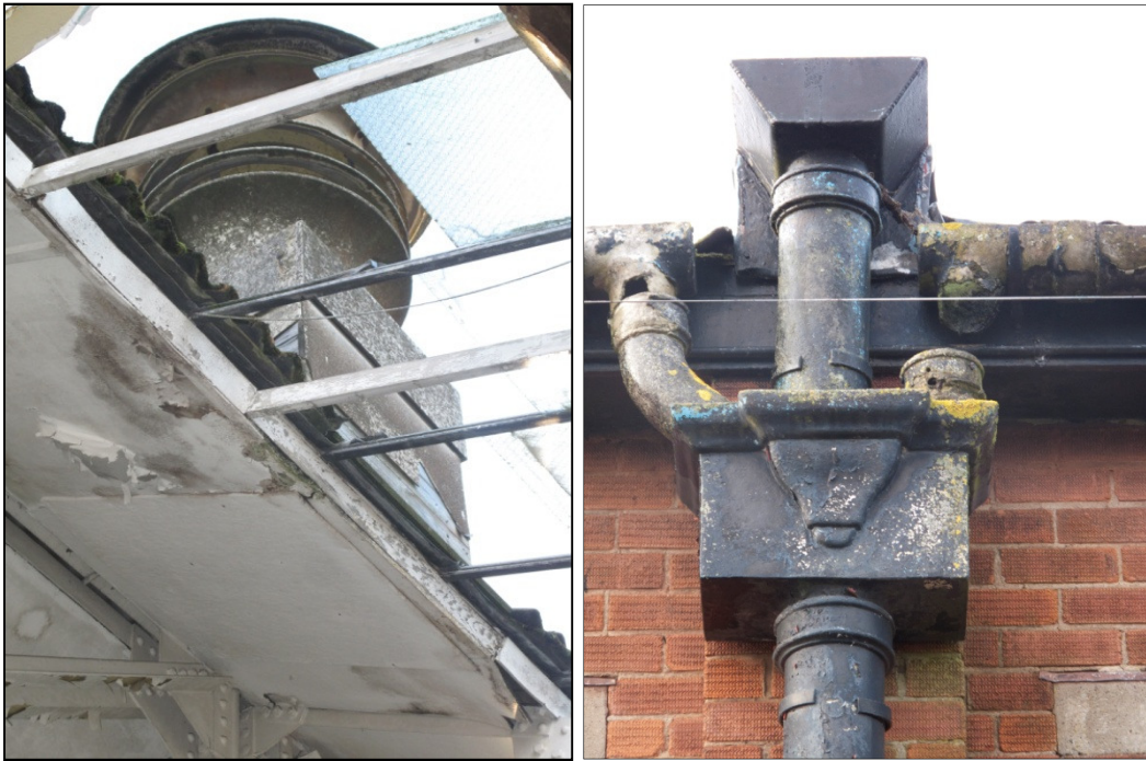
Plate 27: (left) one of the ventilation stacks on the roof of Building 12, with interior access blocked. (Right) decorative trough on down-pipe, connecting valley gutters and eaves guttering
