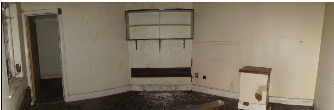
Plate 48: the main reception area; angled fireplace (now blocked) in the corner; doorway leads to southern half of building (compare with Plate 49)
