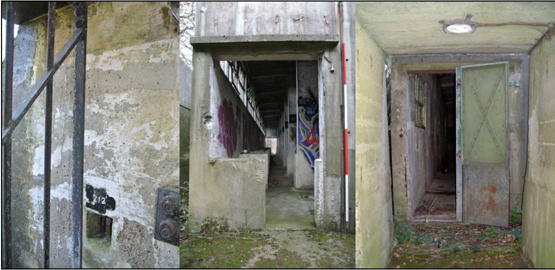
Plate 67: (left) lock box for padlock, and gate, Bunker A; (centre) blast door fittings, Bunker B; (right) cantilevered blast doors, Banstead, Surrey, in 2003 (courtesy Roger Thomas)
