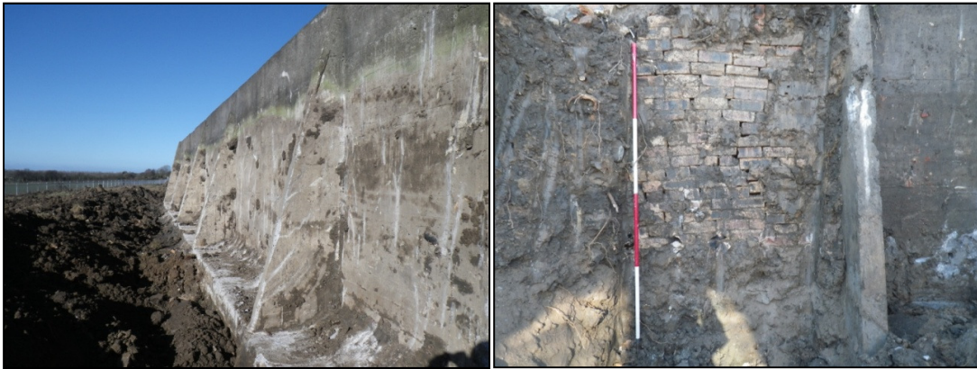
Plate 69: south facing elevation of retaining wall after removal of bund (left) and stacked bricks against retaining wall (right)
