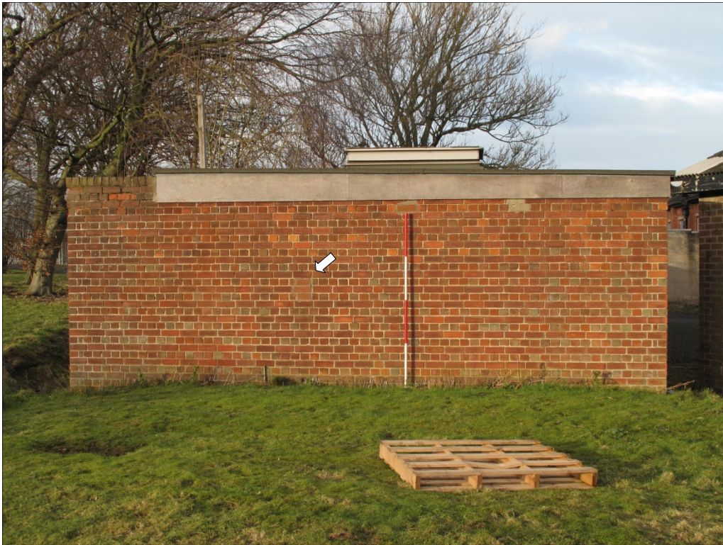
Plate 61: the southern elevation of the toilet block; note blocked hole (centre left) for flue pipe
