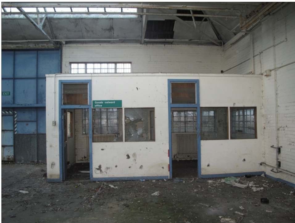
Plate 32: the office in the north-eastern corner of area 12B, showing the ground floor windows in the external wall, radiators within and the modern Area Health Authority signage
