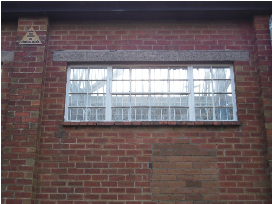
Plate 25: an original window with a pebbled concrete lintel and brick sill. Some brick patching can be seen below it
