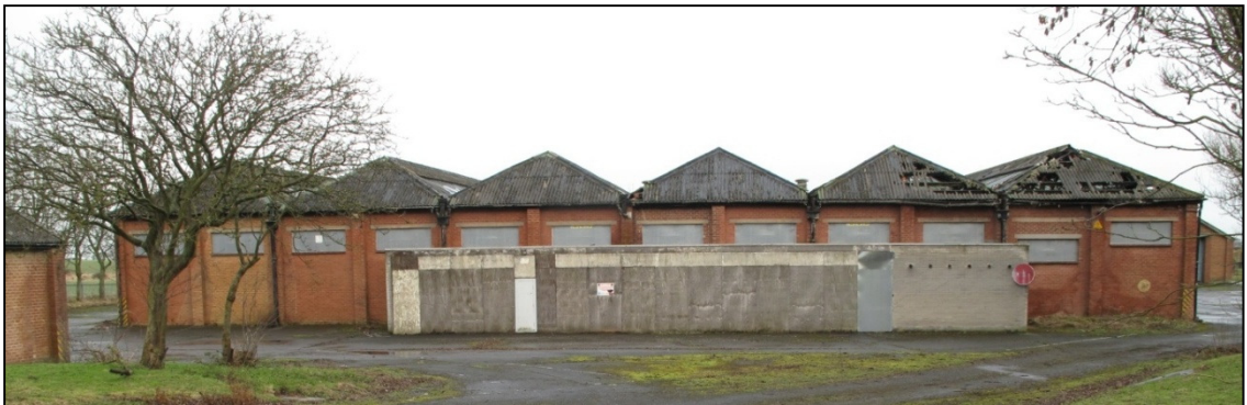
Plate 22: the west elevation of Building 12, with the non-original extension in the foreground, and the altered window second from the right
