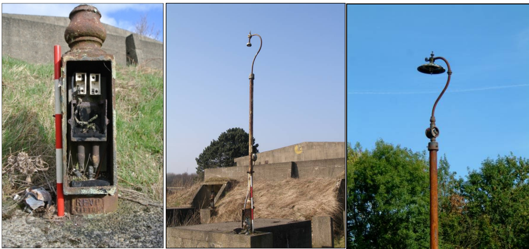
Plate 75: stamped base of lighting column, Bunker B (left) and full lamp-post (right); comparative lamp post from Banstead, Surrey, in 2003 (courtesy Roger Thomas)
