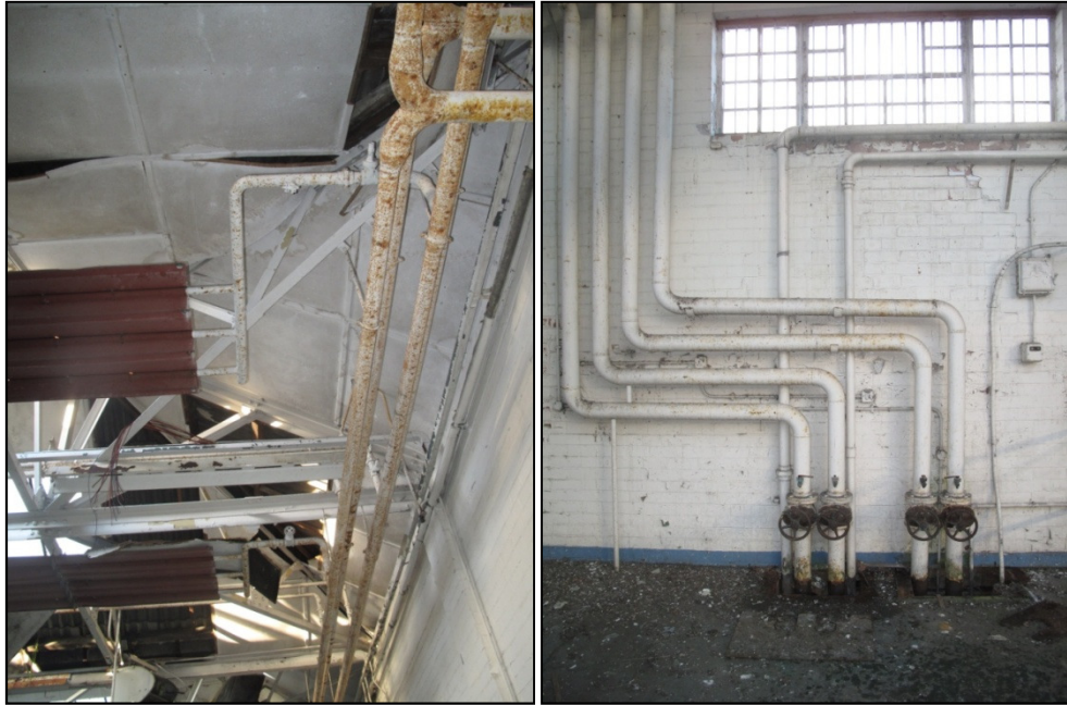
Plate 34: the ends of the overhead radiators, connecting to the heating system (left) and the main heating pipes entering the building to the east, from Building 10 (right)
