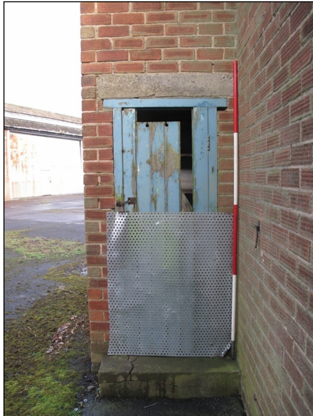
Plate 55: The south-west facing door in the north-west projection of Building 17, giving access to storage
