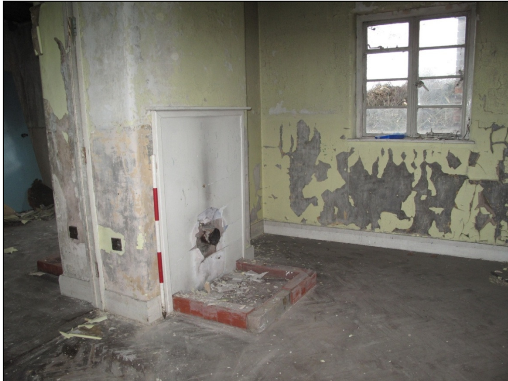
Plate 58: inside Building 17, looking south towards the central wall, and through the smaller of the rear windows
