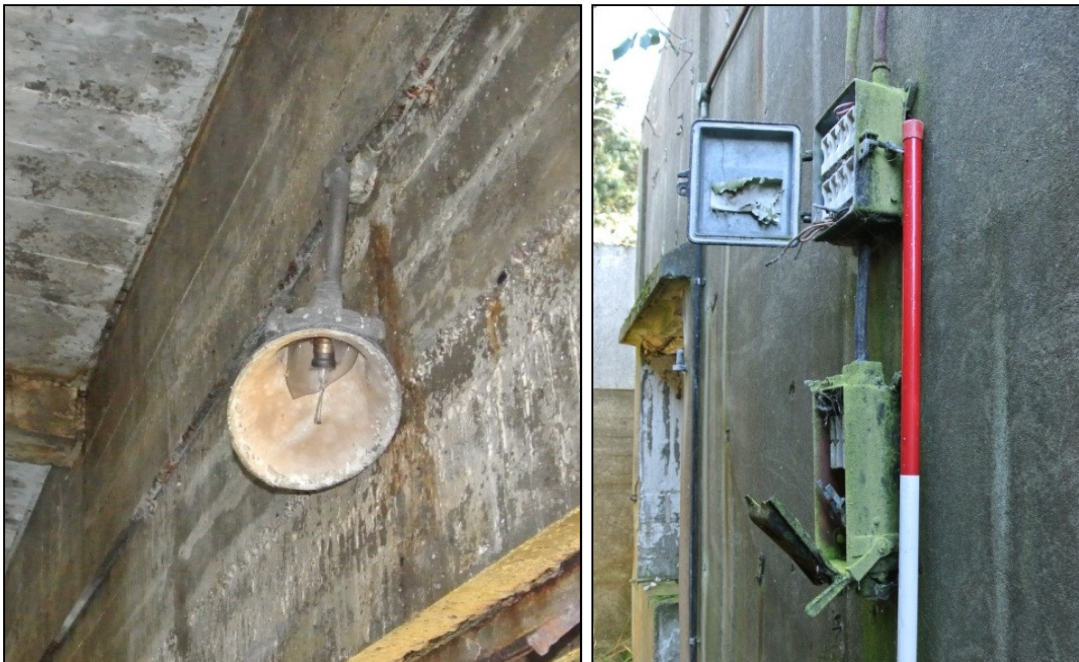
Plate 70: the light fitting (left), and -preserved fuse box (right), Bunker A
