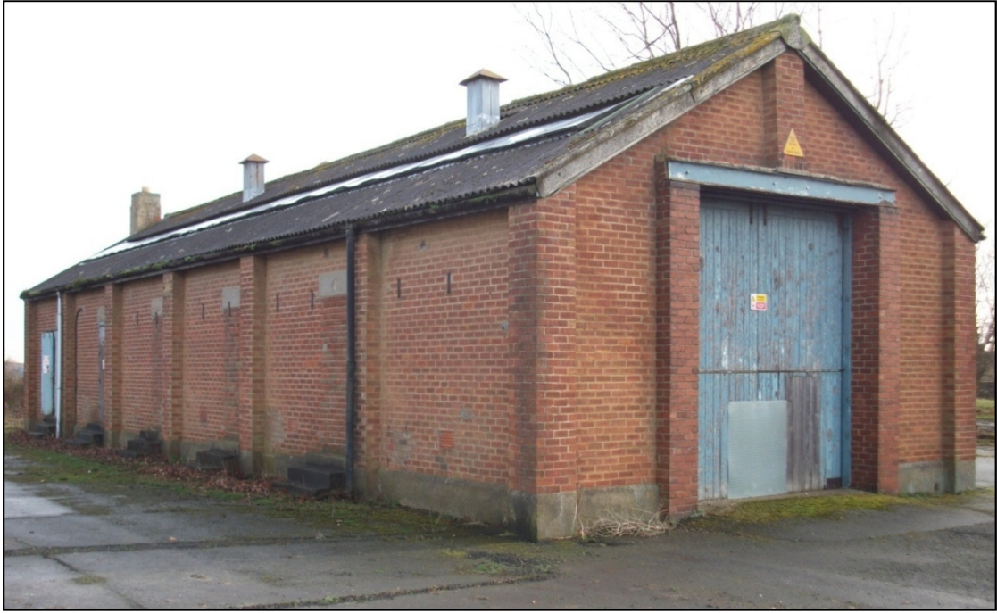
Plate 36: the north-west corner of Building 14, showing the blocked pedestrian doorways on the northern elevation, and the vehicular access door to the west
