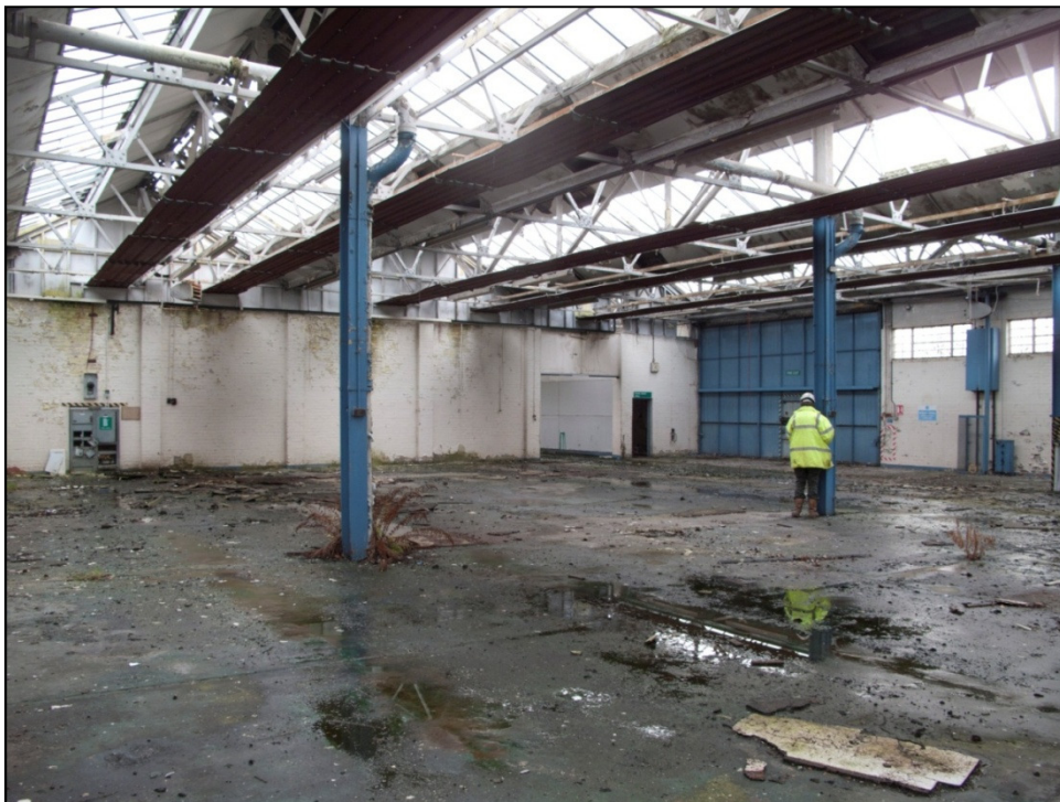
Plate 28: Area 12A, looking south-east toward the central vehicular access door and partition wall. Note down-pipes from valley gutters connected to RSJs, and integrated radiator panels in the roof space
