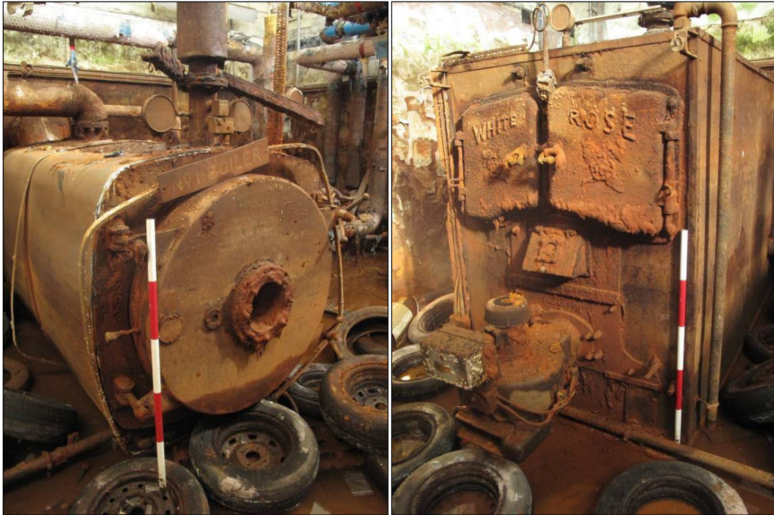
Plate 19: 'Boiler No. 1' (left) and 'Boiler No. 2' (right), facing east
