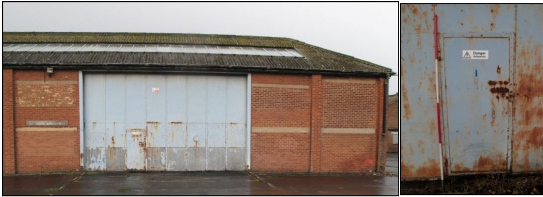
Plate 24: the south-eastern vehicular access door (left), and a detailed view of the pedestrian access (right). The brick panels surrounding the door had been significantly altered
