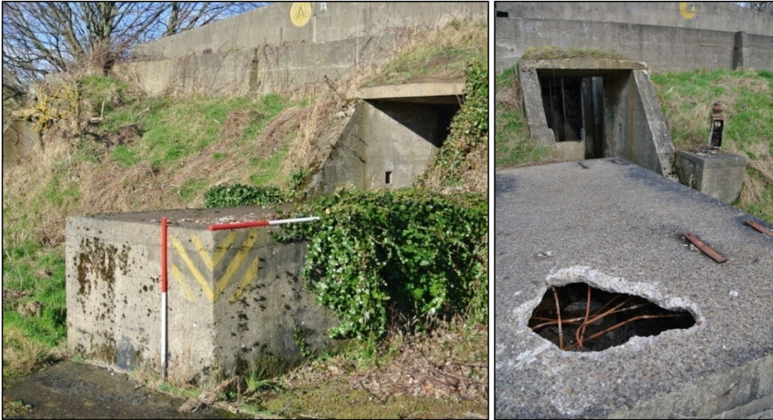
Plate 66: a loading platform outside Bunker A (left). (Right) the damaged loading platform outside Bunker B, revealing the internal reinforcement. Note base in background supporting lamp post
