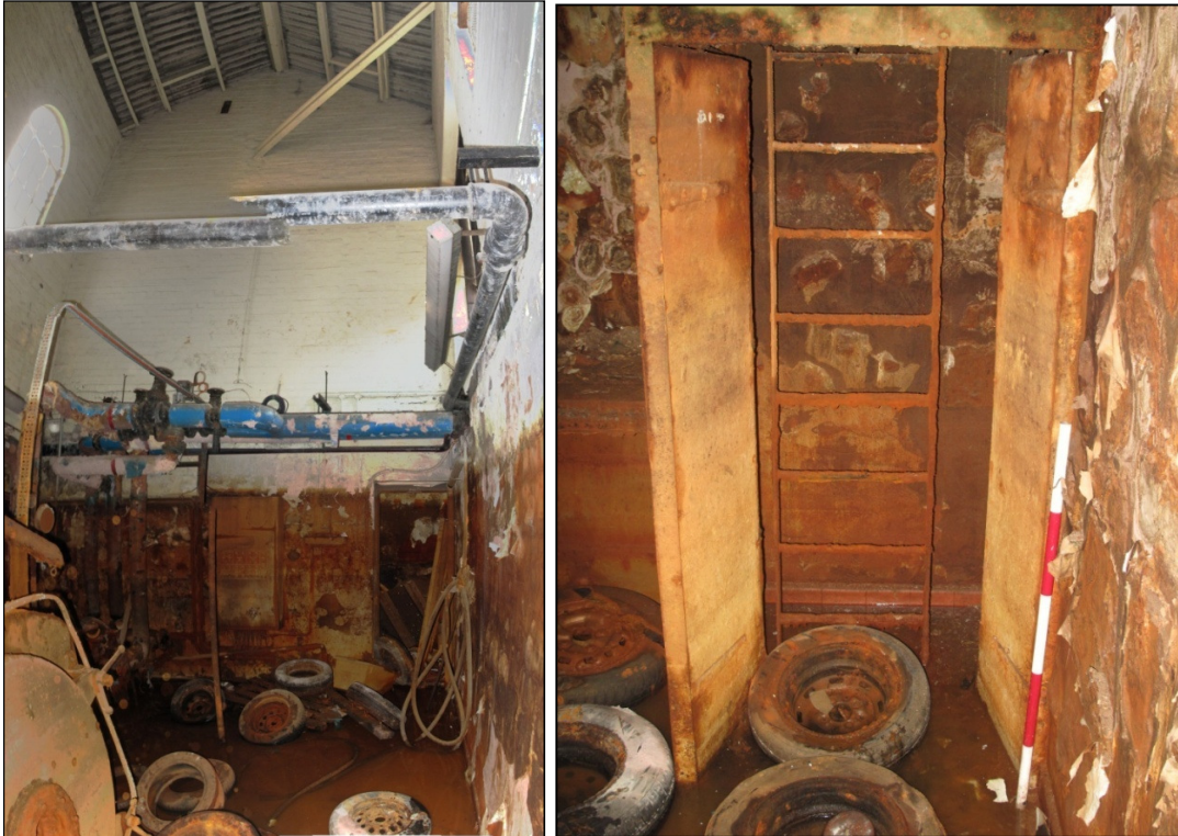
Plate 18: south-facing photomontage of the interior of Building 10, taken from below ground floor level (left), and fire escape ladder in the north-west corner, facing west (right)
