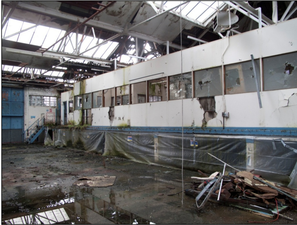
Plate 30: the western end of Building 12, showing the raised platform supported on brick columns, with wood and plasterboard office walls above
