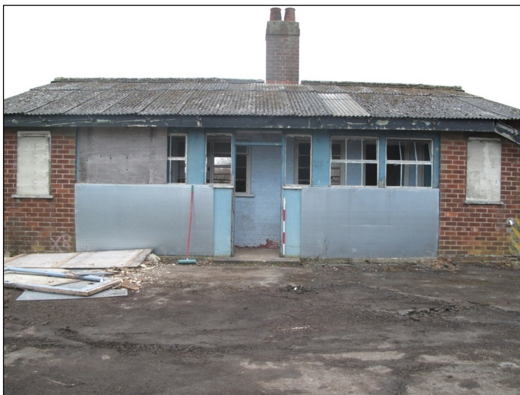
Plate 53: east-facing elevation of Building 17, showing the main entrance, and blocked windows of the rooms either end of the corridor
