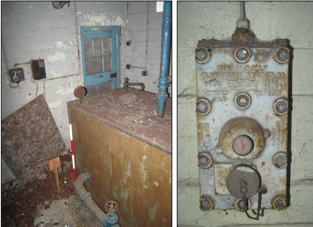
Plate 44: (left) the northernmost room of the later extension, the boiler room, looking south-east. (Right) a flameproof switch plug in Building 14
