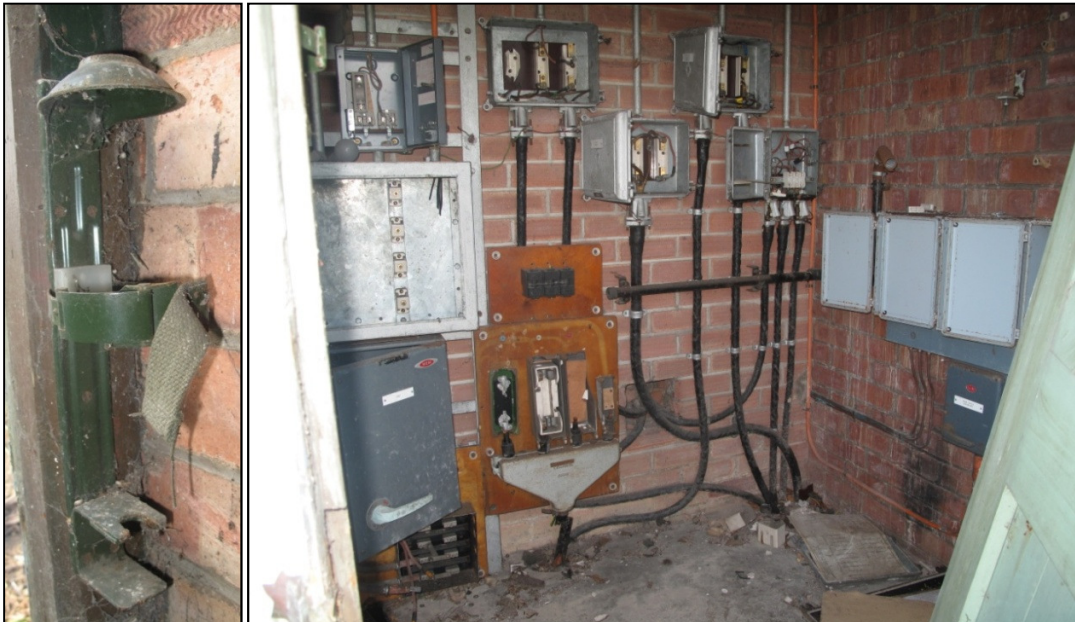
Plate 52: fire extinguisher bracket (left) and circuitry (right), extension, Building 16
