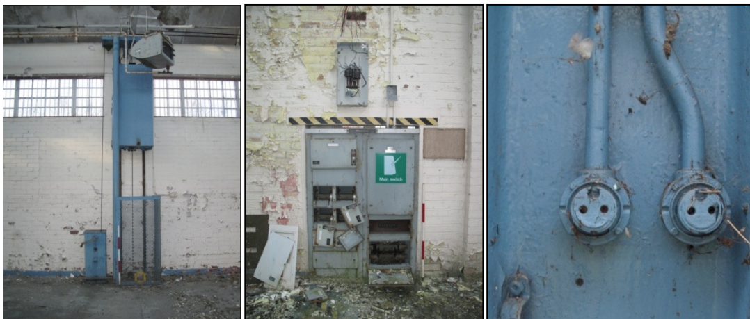
Plate 35: one of the door lift mechanisms (left), the main switchboard (centre) and some electrical sockets installed on an I-section beam
