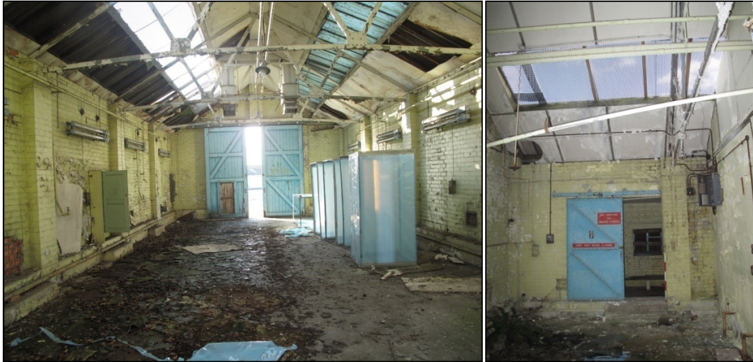
Plate 42: (left) inside Building 14, looking west towards the sliding doors. (Right) surviving sliding door on the easternmost opening in the south wall, with later blocking wall to right of photo
