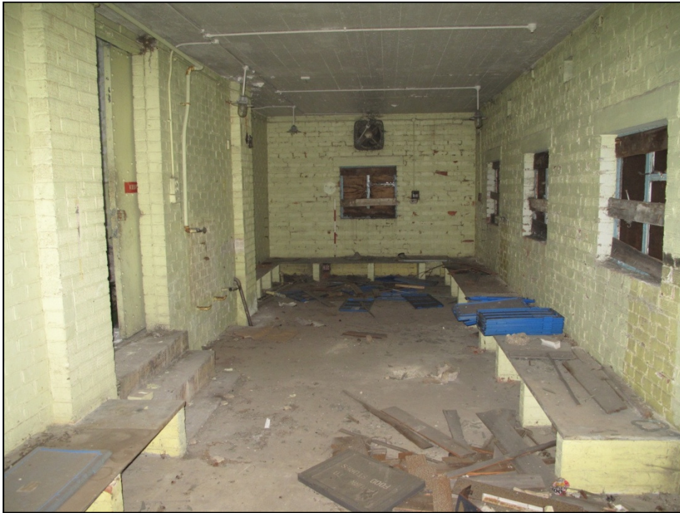
Plate 43: inside the later extension, looking east. Note radiator fittings on wall (left)
