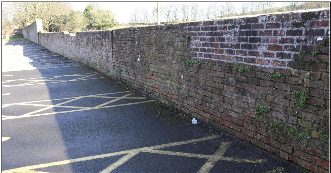
Plate 47: north-facing elevation showing rebuilt section of wall at the west end, associated with the demolished glasshouse.
