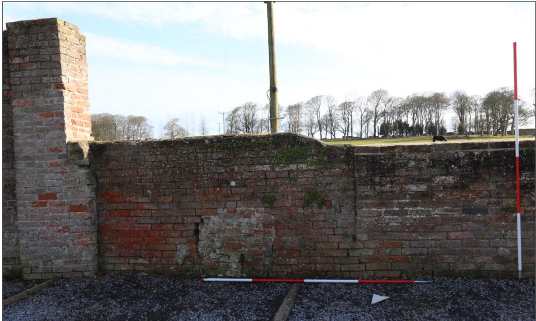
Plate 42: north-facing elevation of the south wall showing wall pier 422 and vertical joint with section of blocking to the east ( 415 ).
