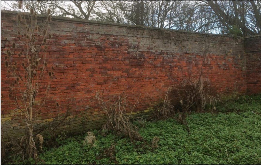
Plate 50: north section of the west wall (500); internal east-facing elevation (north end). Reproduced with kind permission Mosedale Gillatt Architects.
