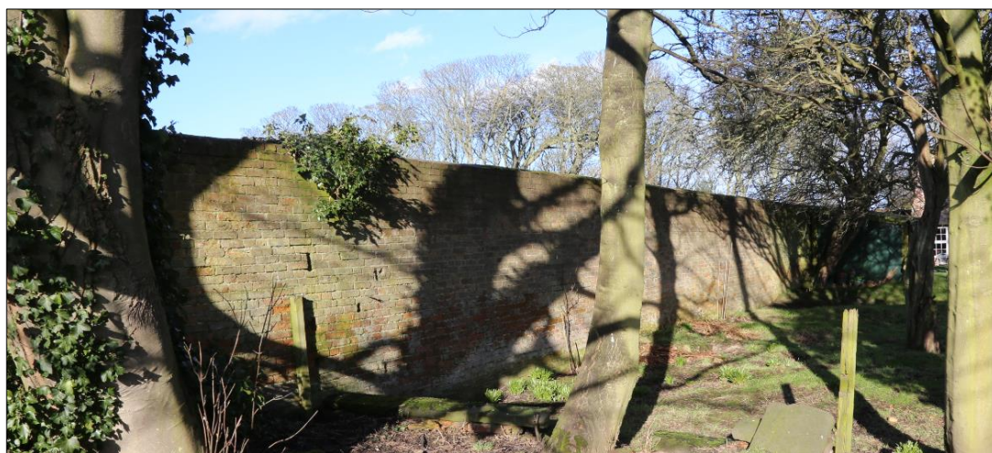
Plates 34: east end of south-facing elevation (410) of south wall (400). Section forms the rear wall of the Gardener's House gardens.
