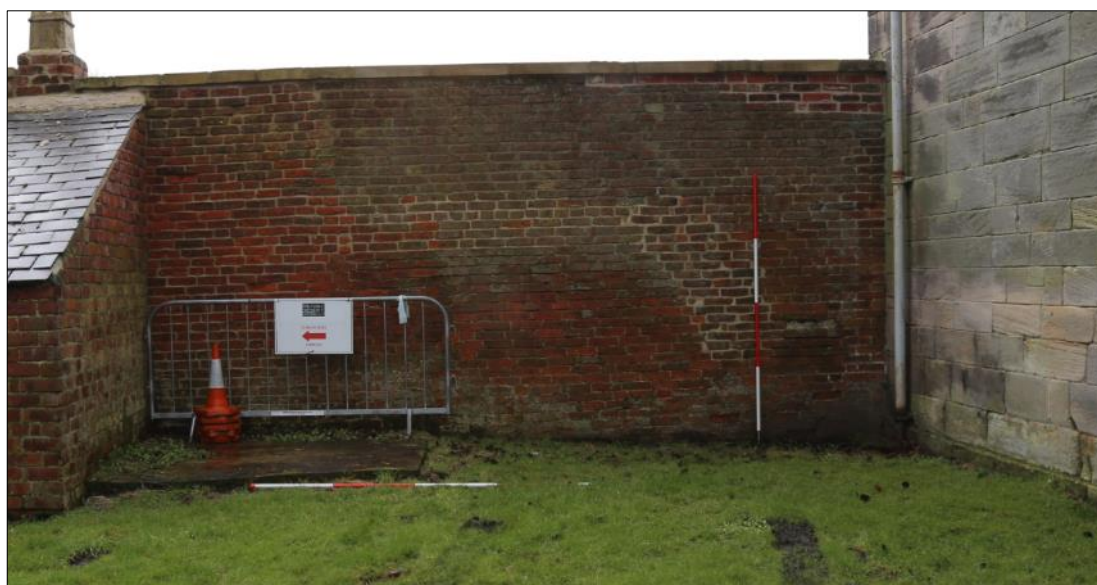
Plate 17: section of wall east of the orangery (facing south) showing scarring associated with building on 1818 plan (221).
