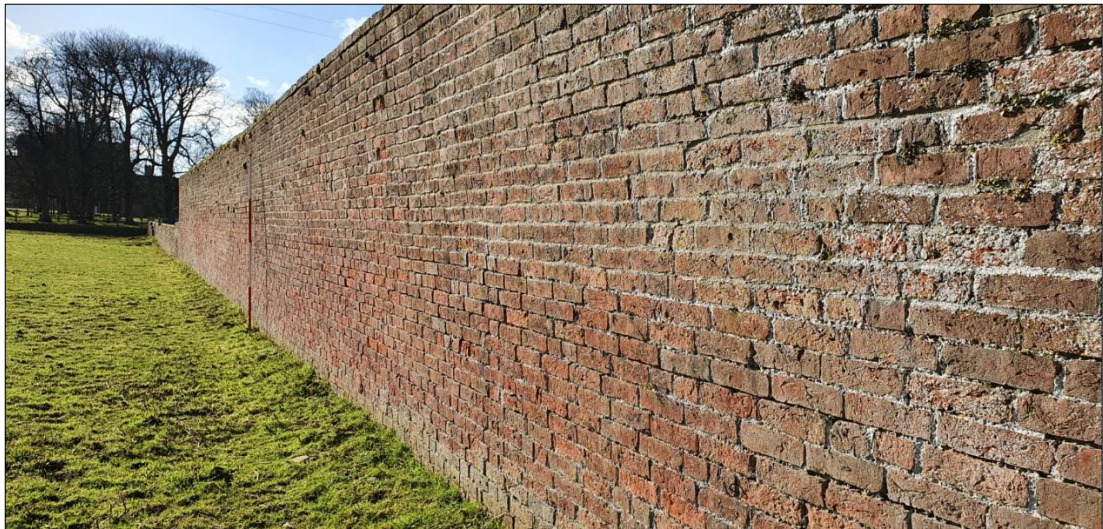
Plate 40: south-facing elevation of the south wall looking west with variation of wall height visible in the distance.
