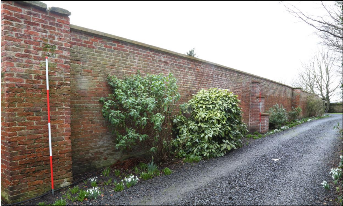
Plate 27: east-facing elevation (310) of east wall (300) with the two square buttresses visible (312, 313) and new stepped buttress in between.
