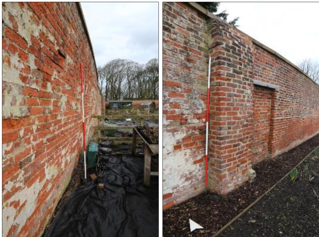
Plates 24 and 25: (left) wall leans inwards where the former 18th-century glasshouse once stood; (right) brick pier 242 with blocked door 221 beyond.
