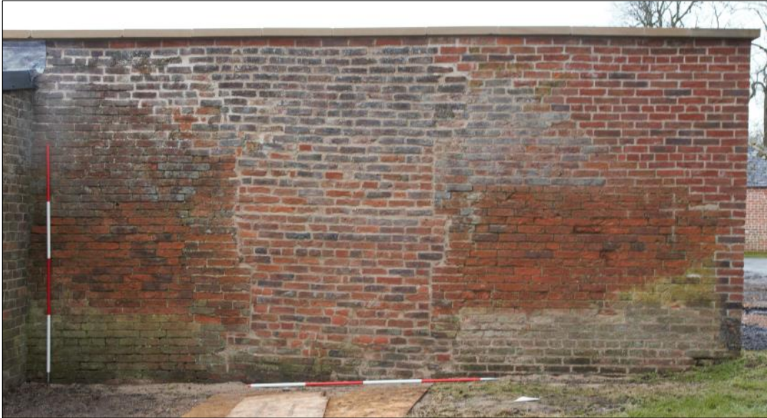
Plate 11: blocked doorway (211) at the west end of the north wall after consolidation.
