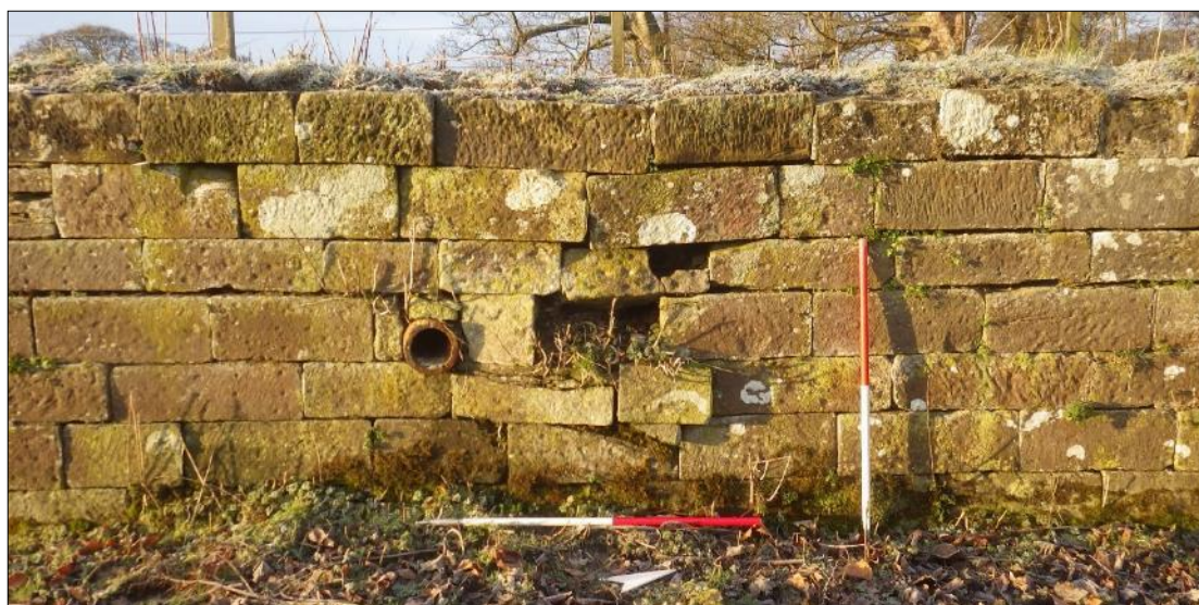
Plate 10: ceramic drain and damage to the south-east face of the ha-ha wall.
