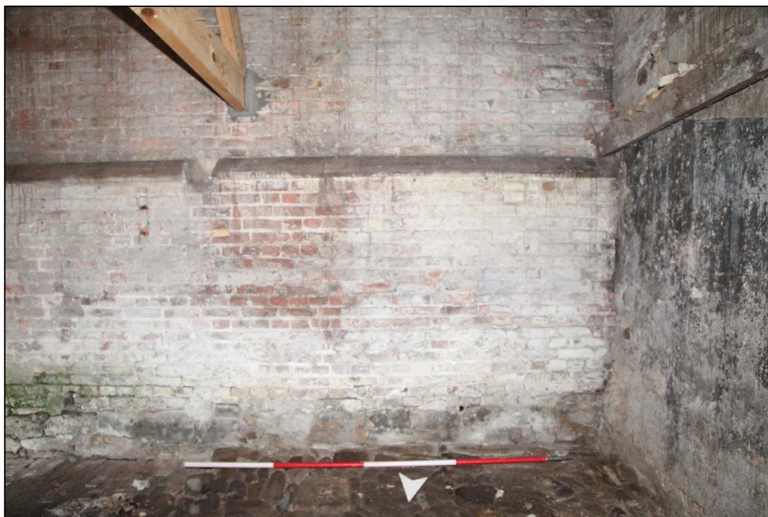
Plate 14: The rear wall of the Potting Shed (300) pre-dates the main building. Note the offset ledge that runs through the entire length of the structure.
