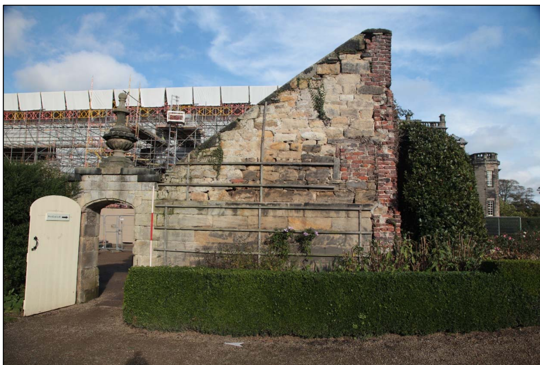
Plate 21: Clear evidence of stratigraphic phasing demonstrated in the west-facing elevation. The original redbrick garden wall (300) is abutted by the ashlar stone boundary wall (202) above which is the stonework (203) of the main structure.
