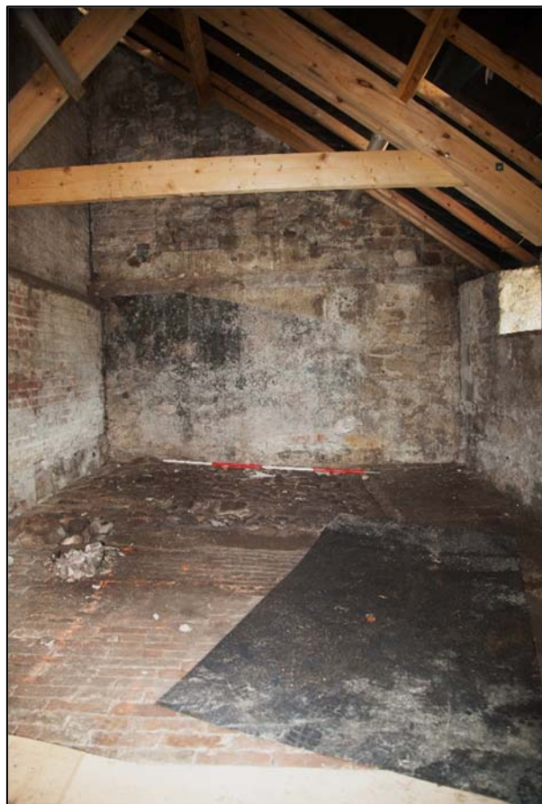
Plate 12: The south-east elevation. The blocked window is partially hidden by the truss.
