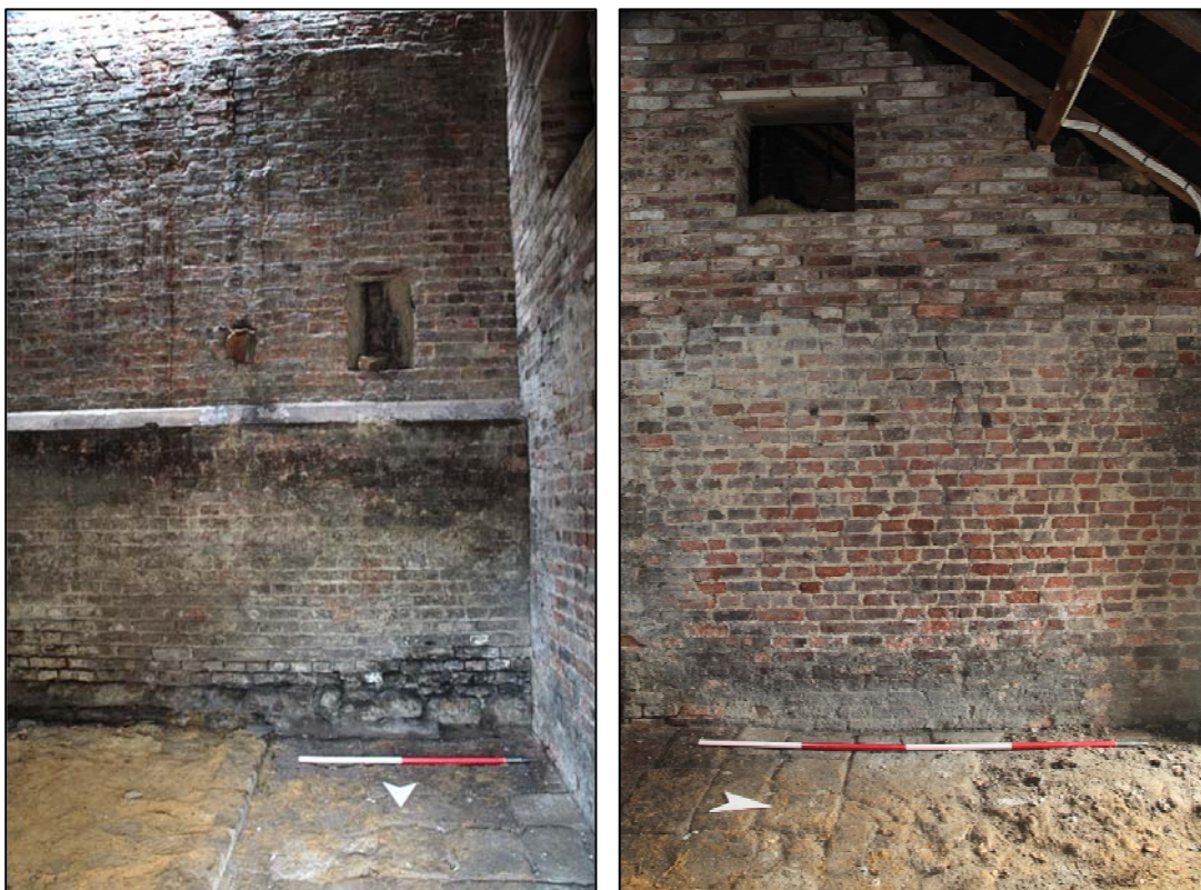
Plates 6 and 7: South wall of east-central room (left) showing the different floor surfaces and western ventilation slit (1213), and the western partition wall with first-floor opening (1221).
