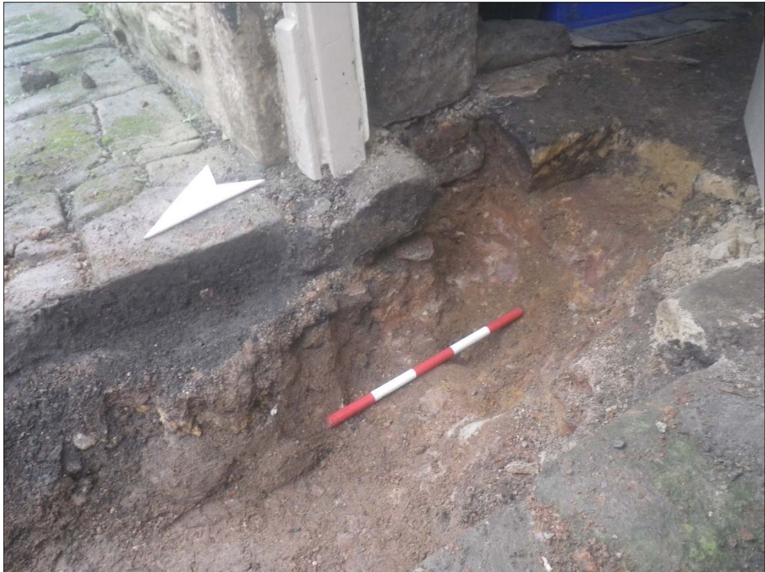
Plate 3: potting shed wall and floor bedded onto clay layer 3003, with foundation cut 3008 on the left.
