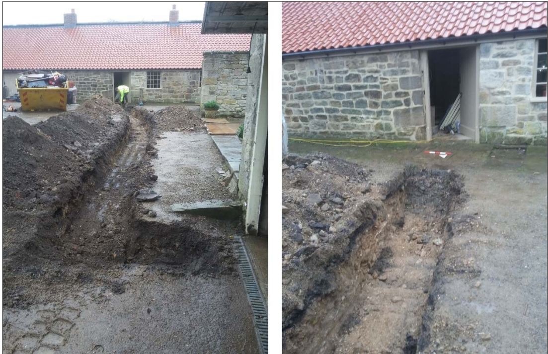
Plate 1 (left): service trench as excavated, with (deposit 3004 visible in its northern extent; Plate 2 (right): natural sandstone (3001) exposed at the southern end.
