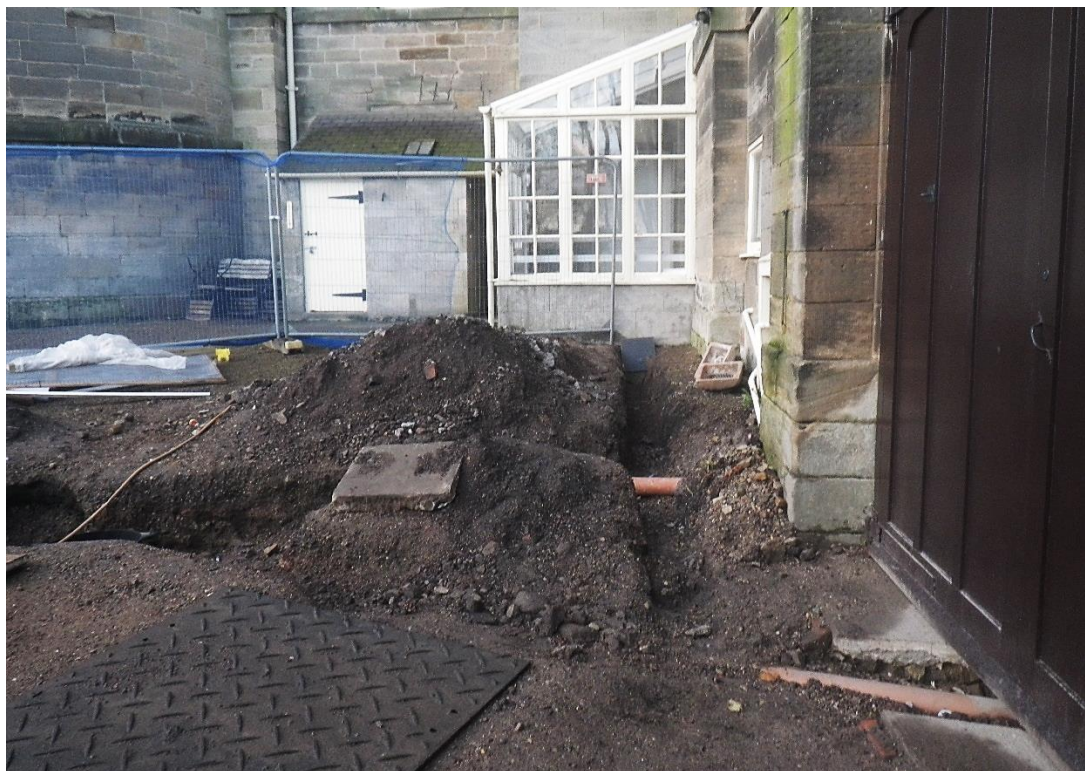
Plate 1: electrical cable trench during excavation (and realignment of drainage in the stable yard), looking south-west. The lean-to structure is in the background.
