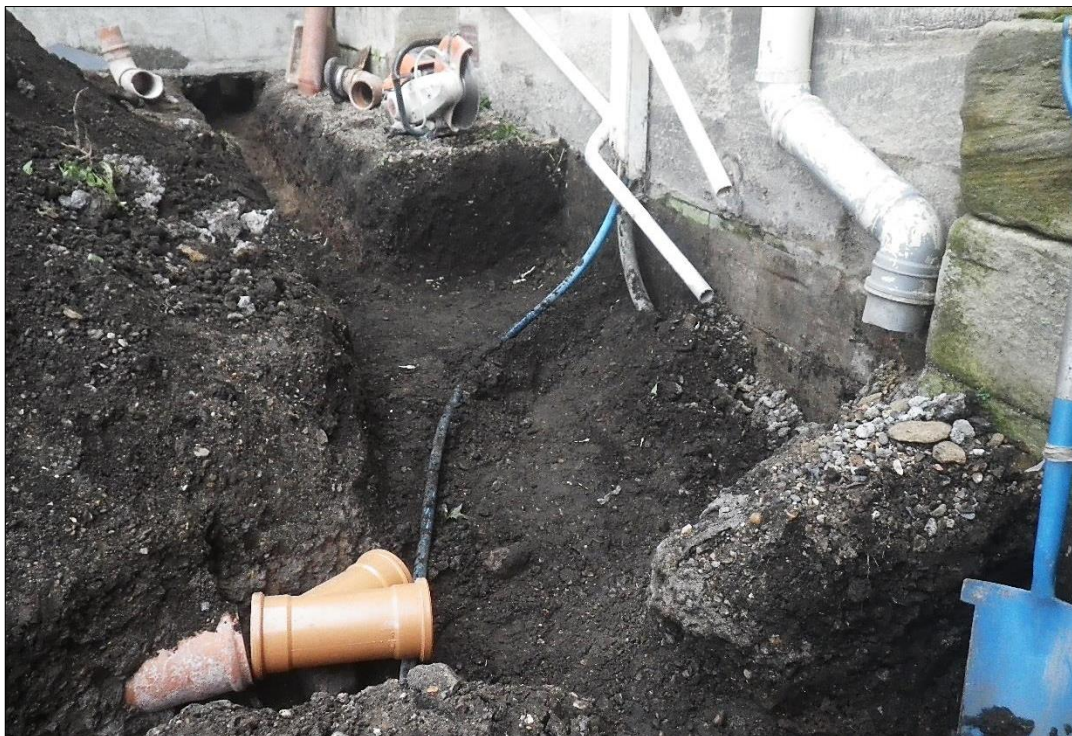
Plate 5: deposits in the stable yard after removal of disturbed modern deposits, with natural sandstone visible beneath the lean-to wall, looking west.
