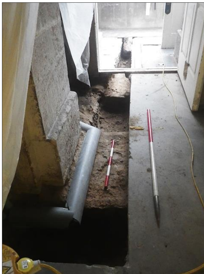
Plate 3: wall footings 1001 and 1002 in the East Wing north passage, with modern electrical cabling on the left of the photograph.
