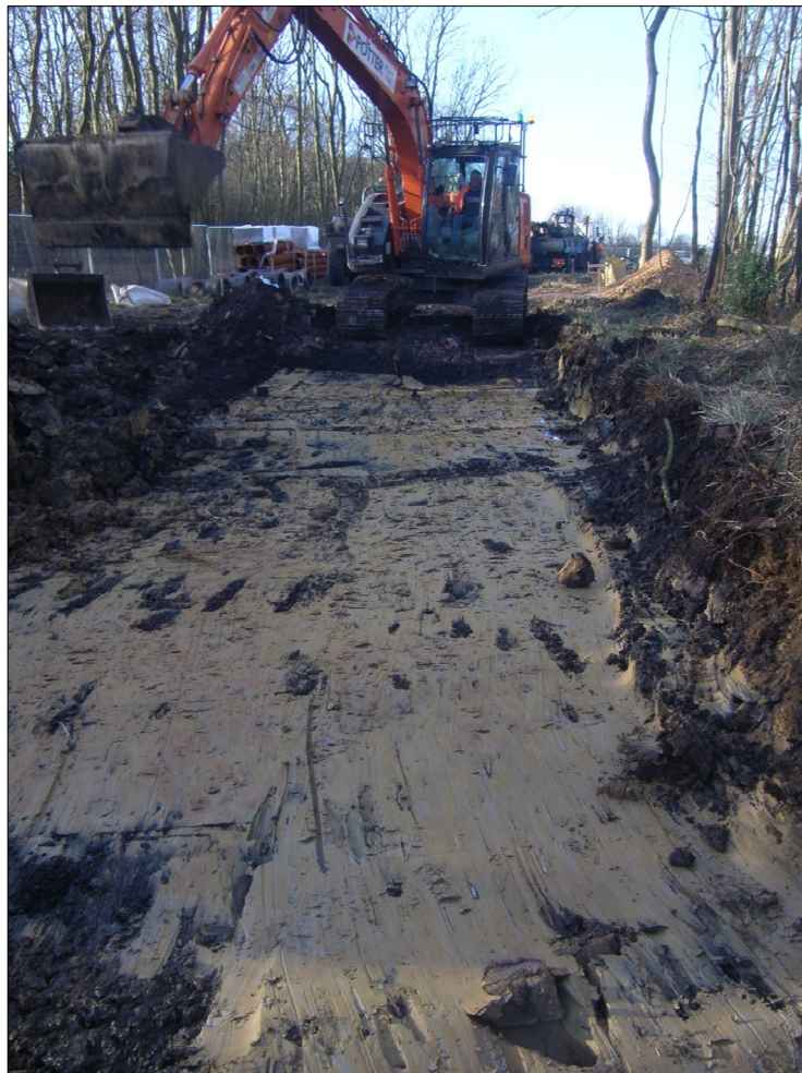
Plate 1: Excavation of the access track showing modern makeup of the track overlying the natural clay.
