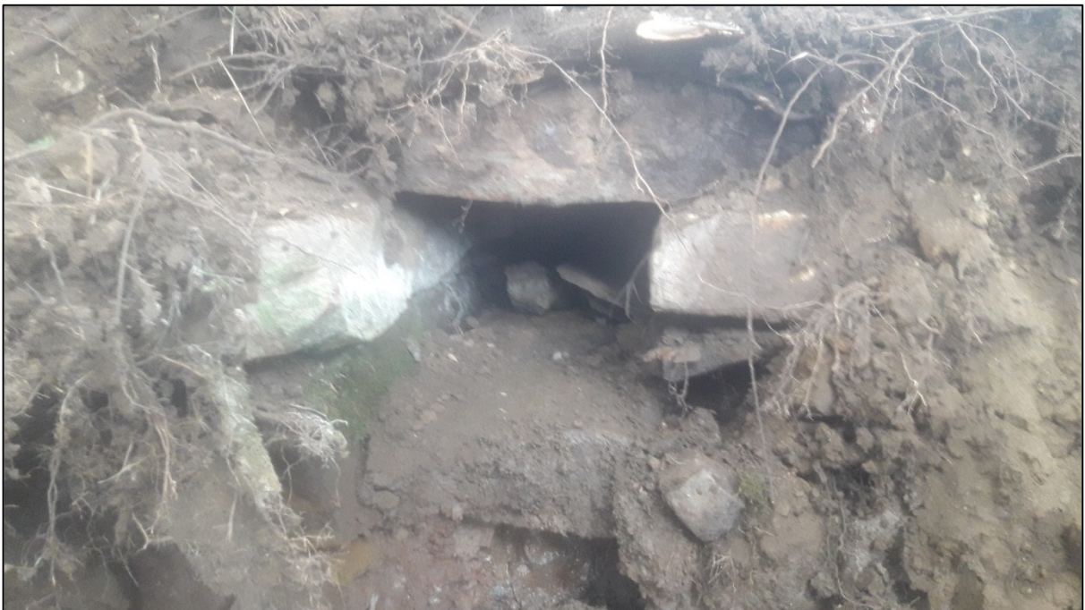
Plate 3: Heavily disturbed sandstone culvert.
