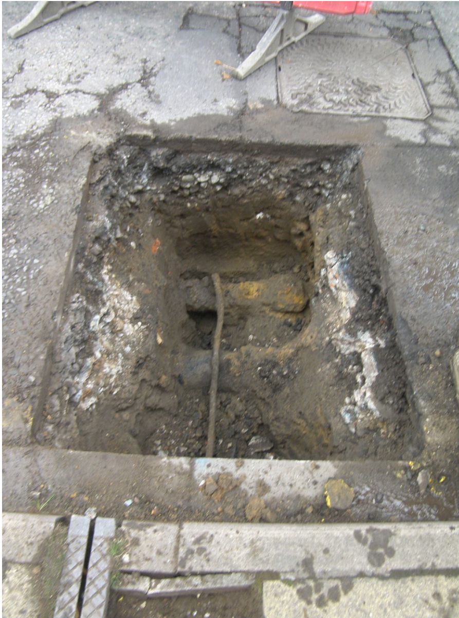
Plate 1. Typical lead replacement pit (Clifton Green) showing two cast iron water mains (one capped with concrete) and small diameter lead pipe. A further service is indicated by the manhole and the paler fill in the rear of the pit
