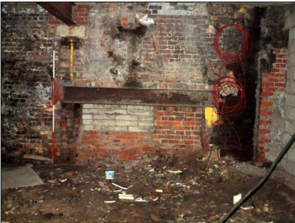
Plate 60: Blocked low opening in north wall
