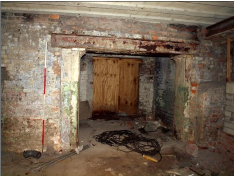
Plate 52: Area to the south of the hoist showing iron jambs and capitals
