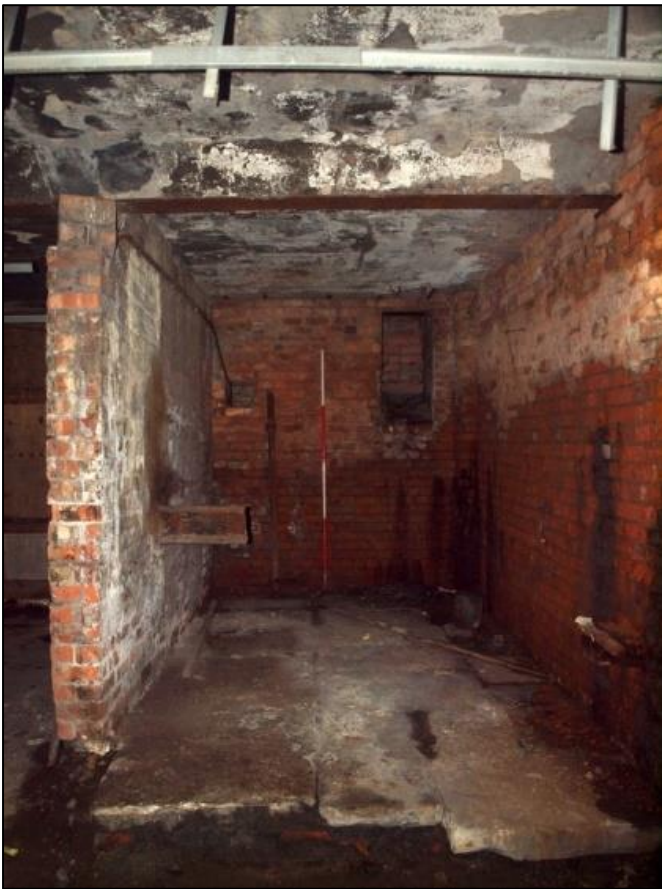
Plate 46: Southeast corner of mill showing small 'room' in south end of east wall
