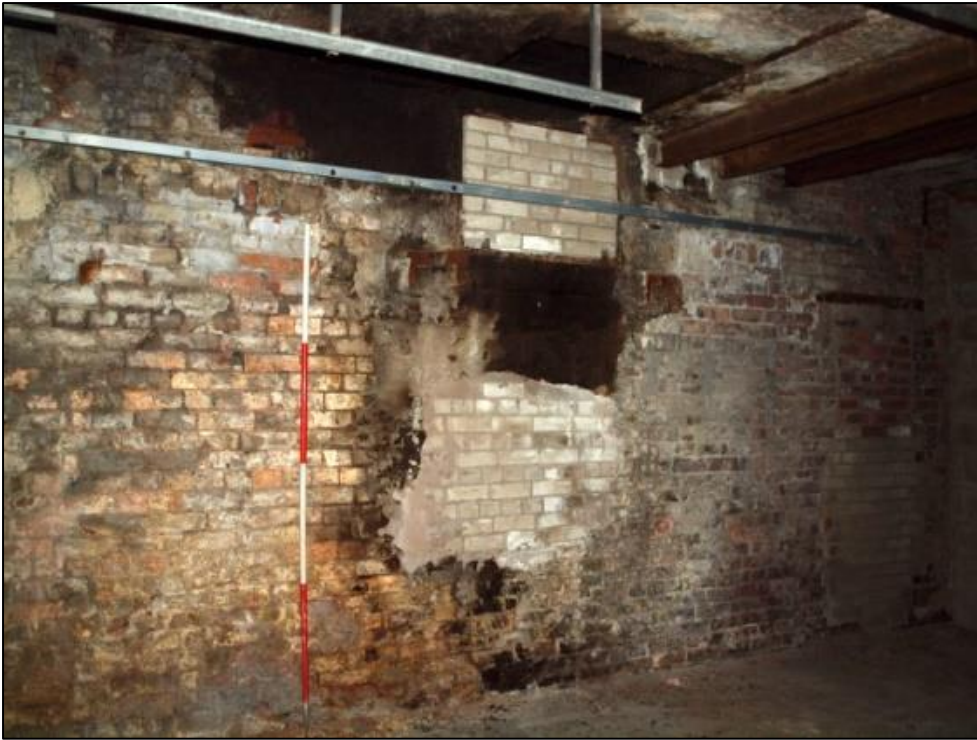
Plate 49: Transmission window in east wall of room above with hatch above and blocked door to the south (right)
