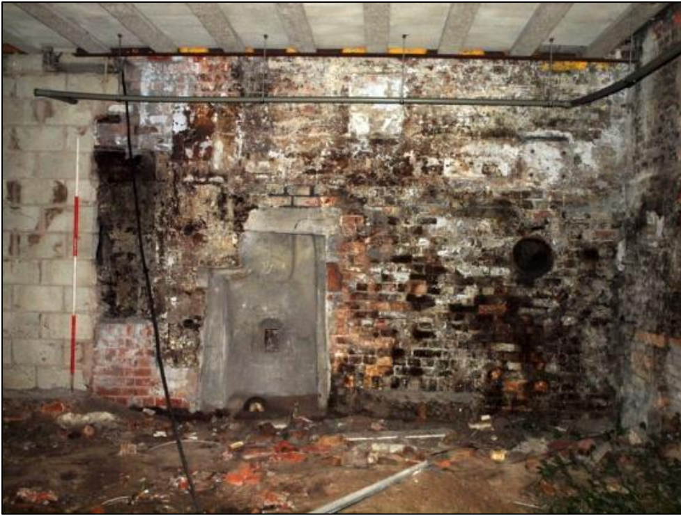
Plate 61: Detail of east wall showing blocked opening to the north (left) with adjacent sandstone blocks, rendered recess and brickwork (right)
