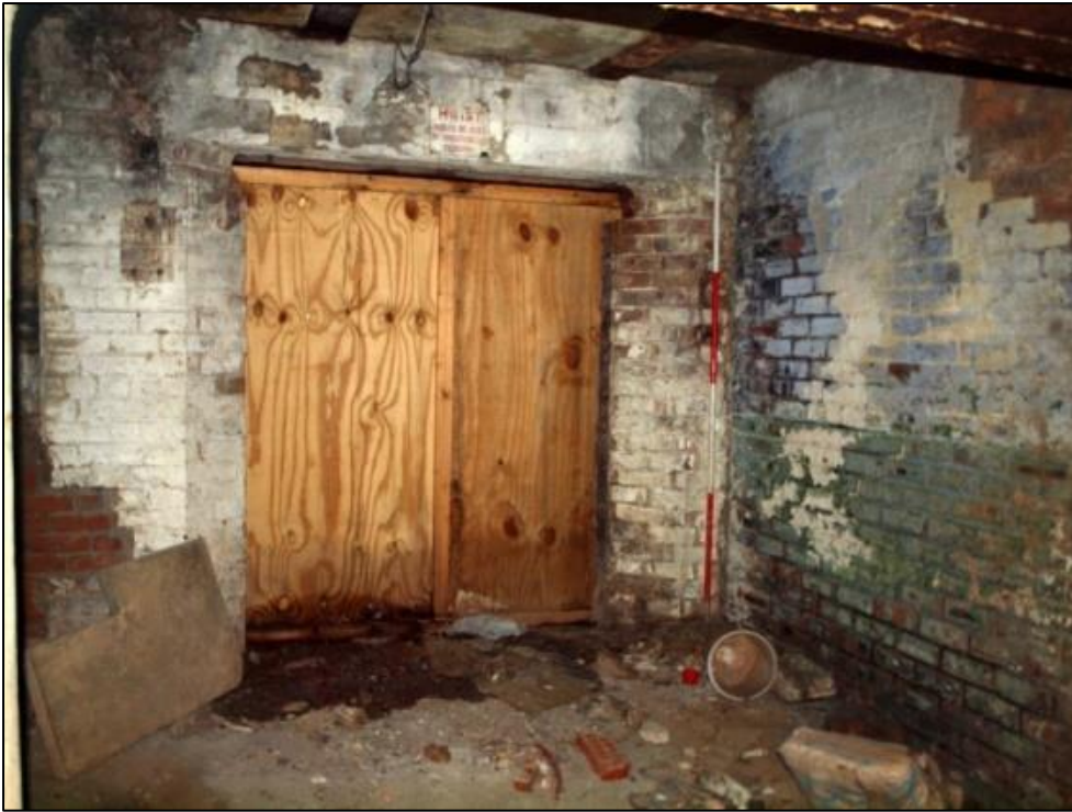
Plate 51: Blocked entrance to the hoist
