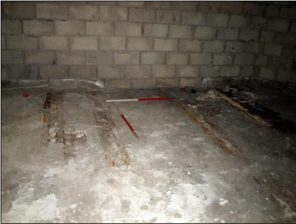
Plate 41: Iron rails set in concrete floor at southern end of room above
