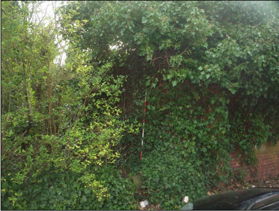
Plate 19: Overgrown north elevation
