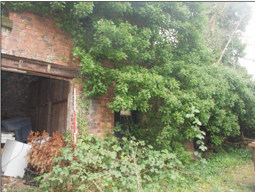
Plate 8: Overgrown northern end of east elevation showing loading door to bay 2
