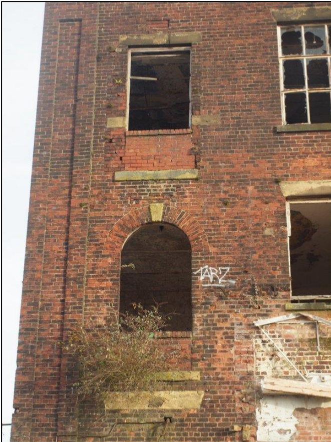
Plate 19: Detail of bay 1 showing doorway converted to window at first floor level, with rounded lintel and keystone, with doorway converted to window above
