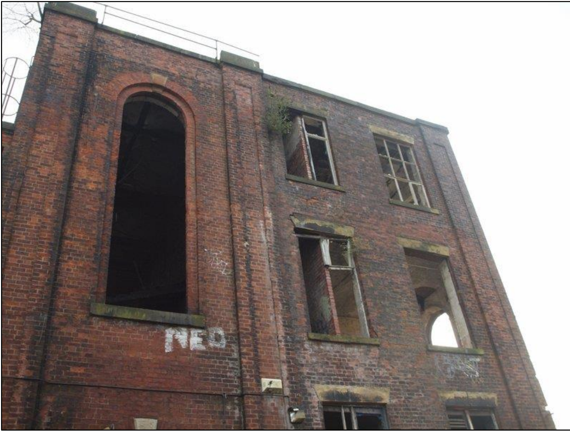
Plate 15: Boiler house upper floor windows shown in relation to the engine house window.
