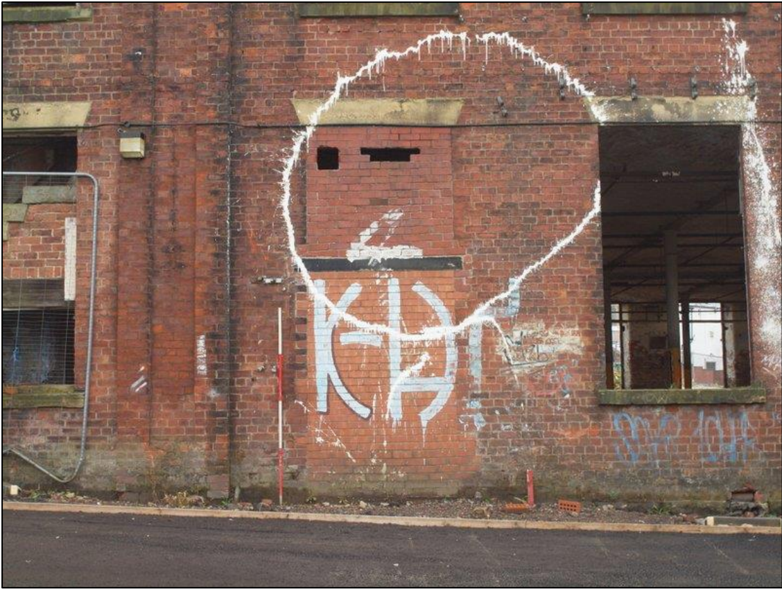
Plate 5: Detail of ground floor bay 2 showing blocked window with blocked inserted doorway
