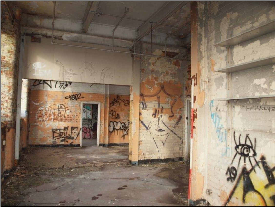
Plate 89: Inserted room in boiler house
