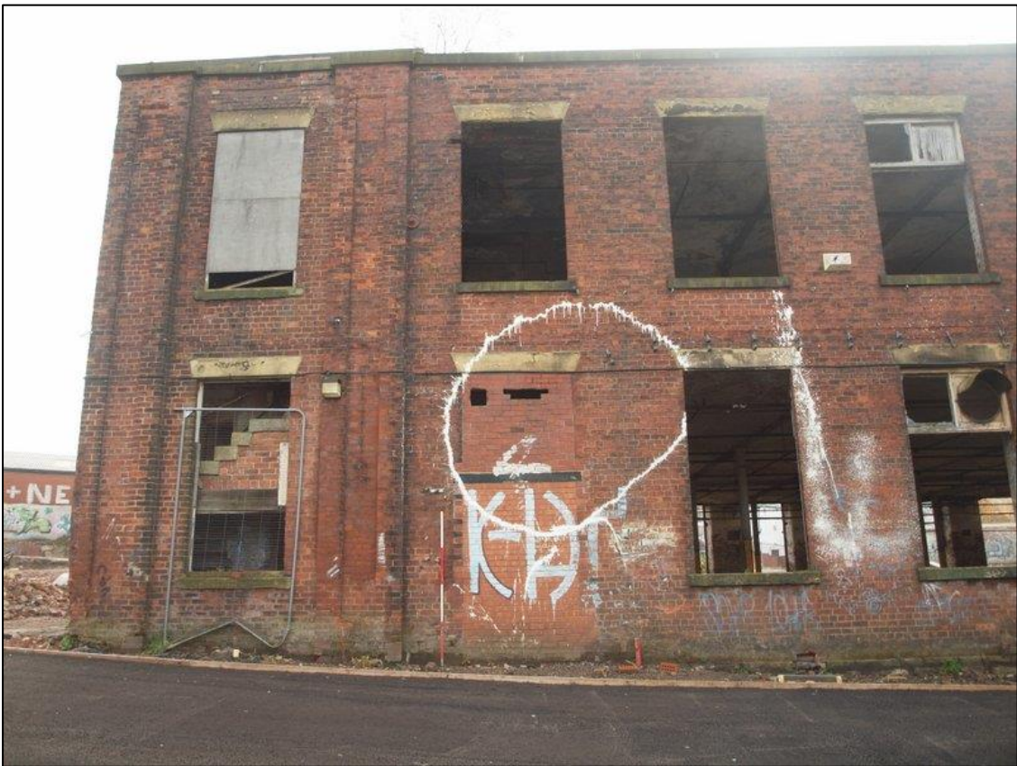
Plate 4: Northwest elevation bays 1 to 4, with staircase cutting across the bay 1 ground floor window.
