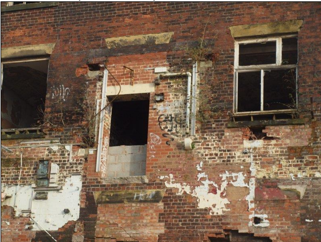
Plate 20: Detail of blocked window with doorway inserted in bay 3 at first floor
