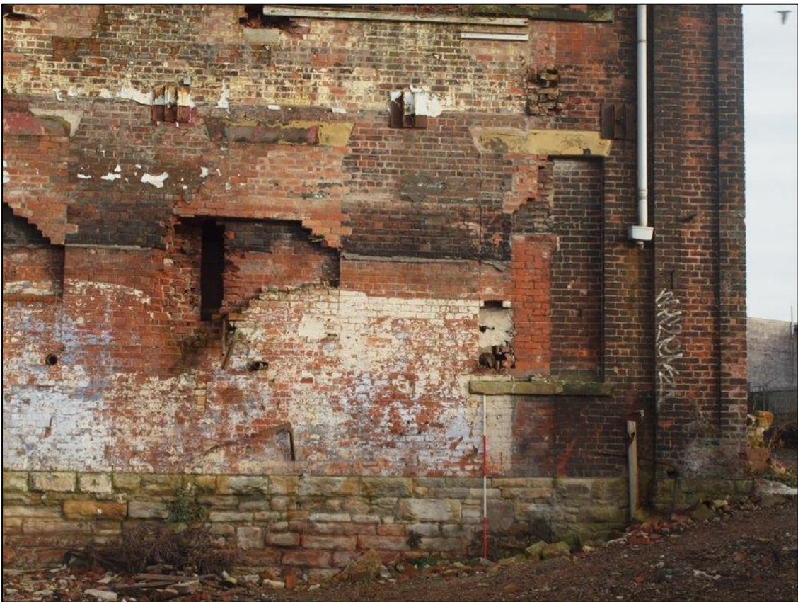
Plate 22: Detail of bays 5 & 6 at ground floor level showing blocked window and ghost of former building.
