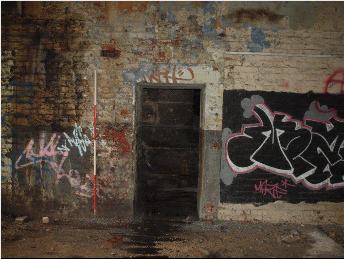
Plate 51: Doorway shown in plate 48 opening onto the stone face of the engine base
