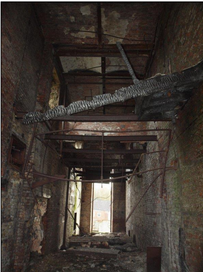
Plate 82: Upper floors of engine house showing collapsed floor
