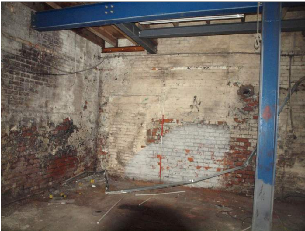
Plate 32: Personnel doorway inserted into blocked window at north end of east gable, also seen externally.
