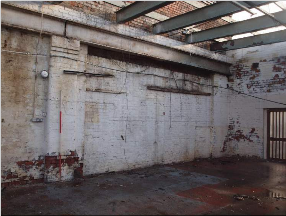
Plate 39: Large blocked opening in north wall showing blocked loading door and blocked personnel door within.
