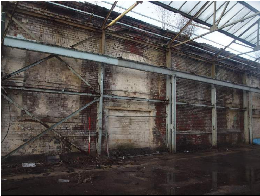
Plate 25: Blocked windows and inserted loading bay on south wall (former external wall of boiler house).
