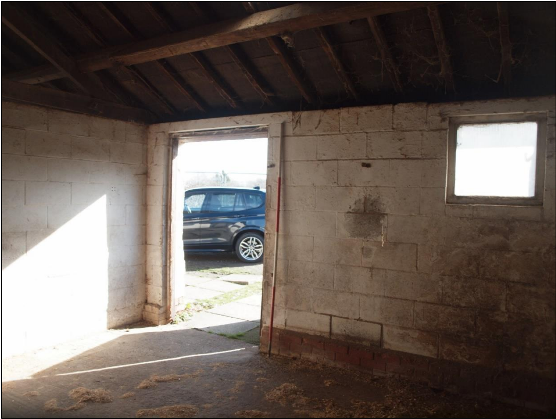
Plate 103: Inserted wall to main frontage
