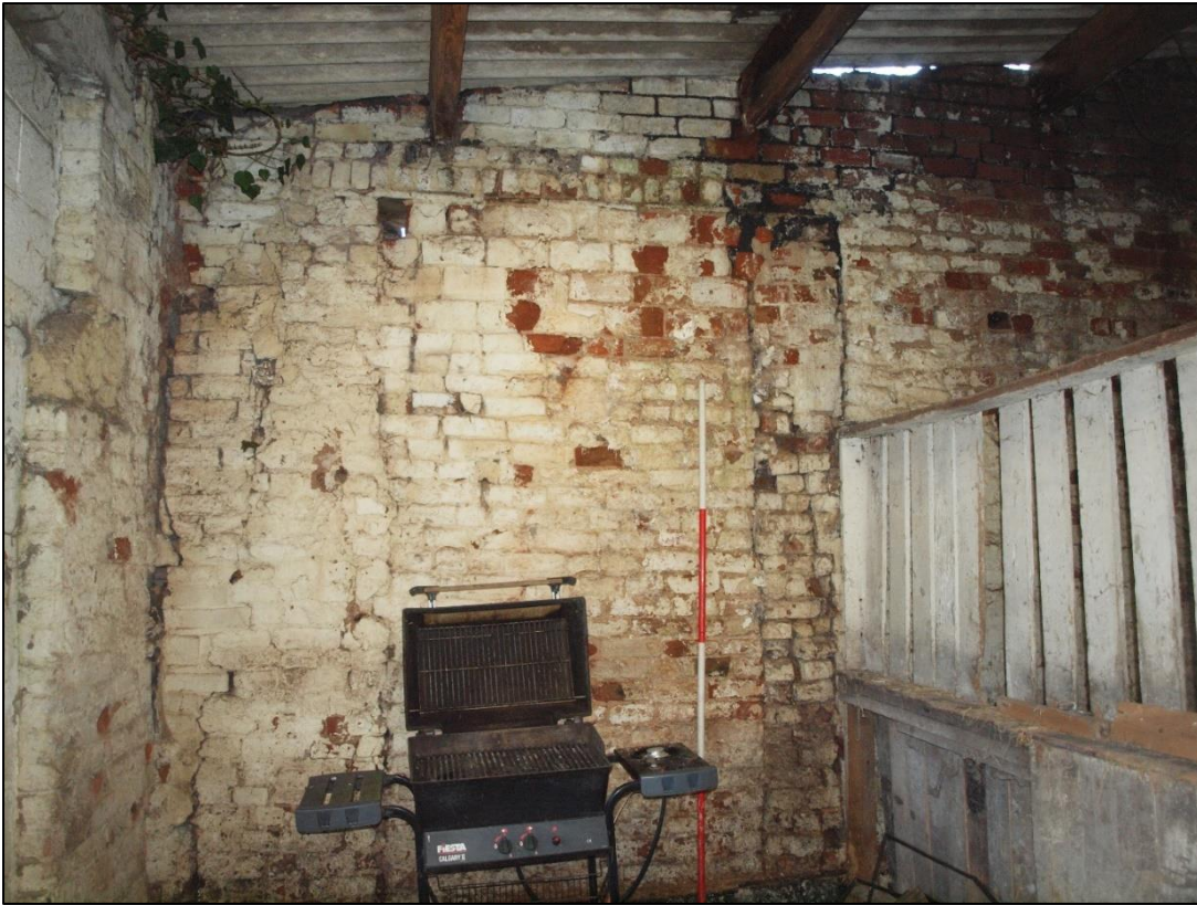
Plate 123: Large blocked opening from eastern unit with wall scar to the right
