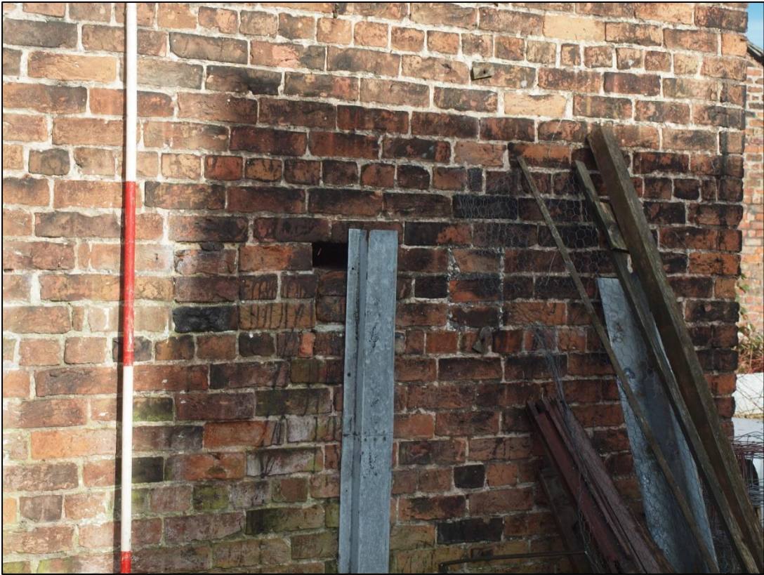
Plate 41: Blocked ventilation holes
