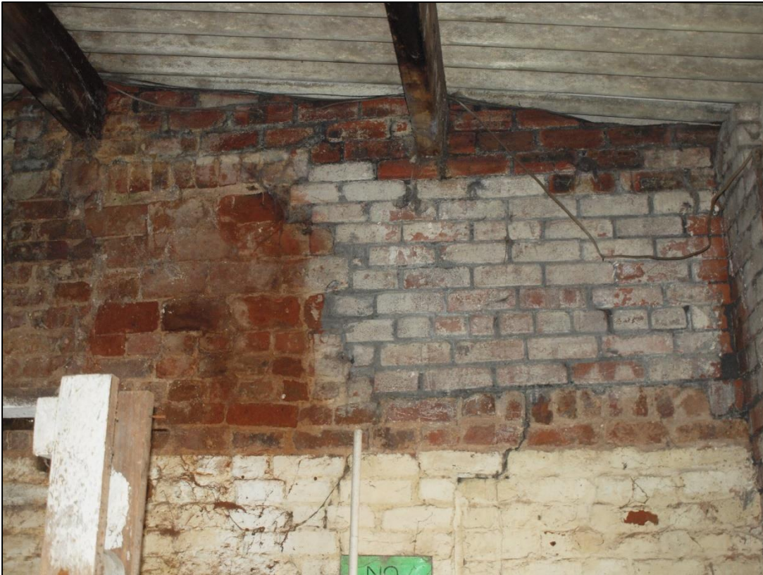
Plate 121: Blocked opening high in face to west of entrance
