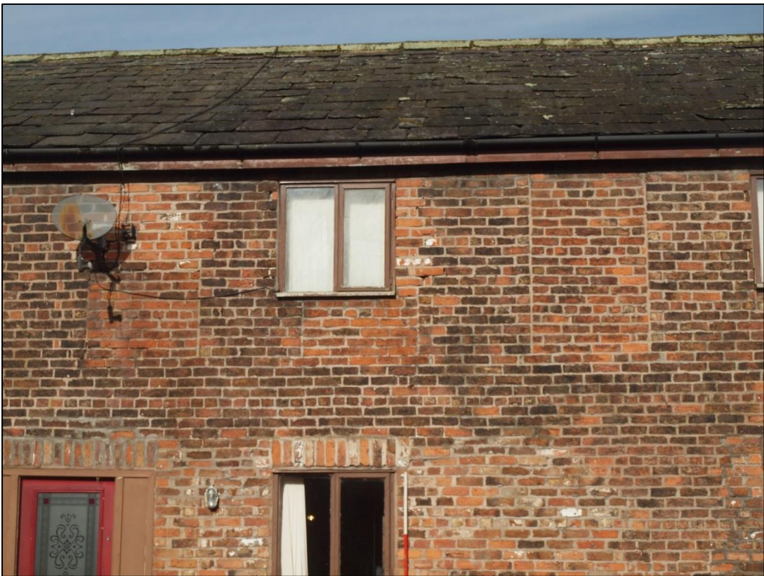
Plate 52: Blocked windows at first floor level
