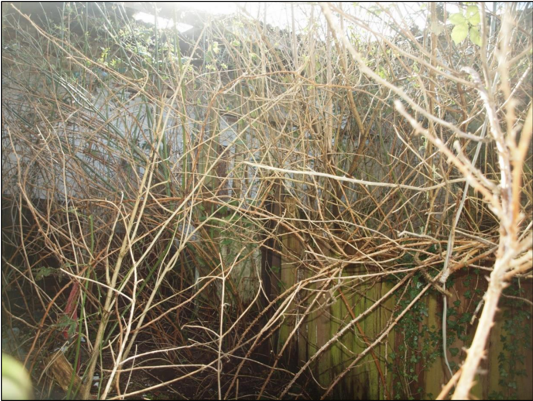
Plate 115: Derelict eastern unit showing timber stall
