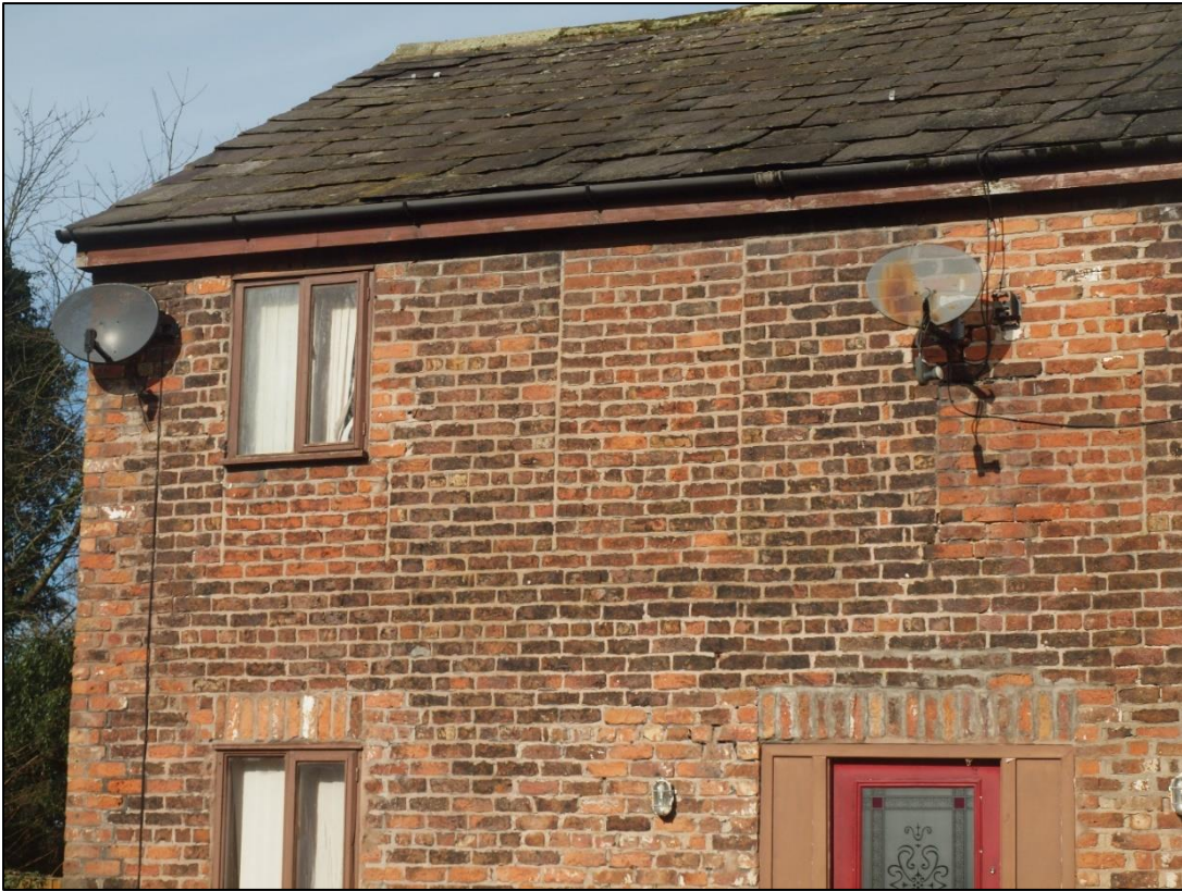
Plate 53: As above also showing rough joint to left where gable has been rebuilt
