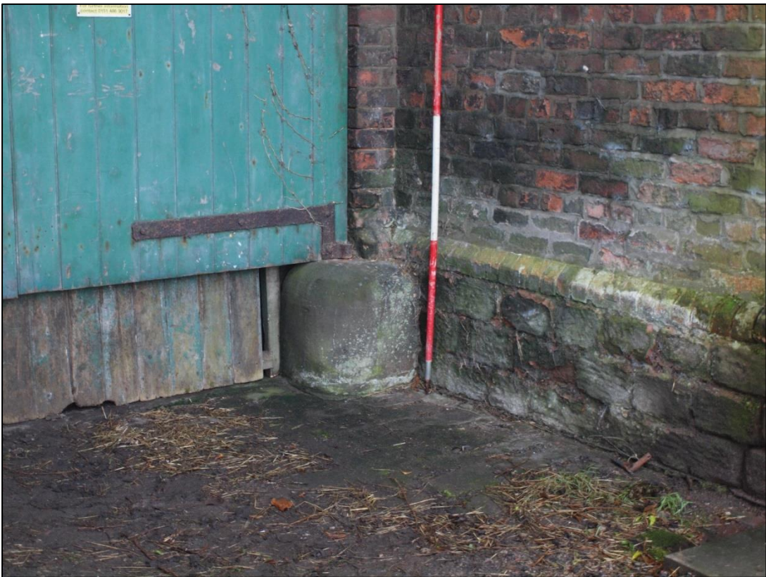
Plate 8: Detail of stone base to barn door jamb with groove containing timber board
