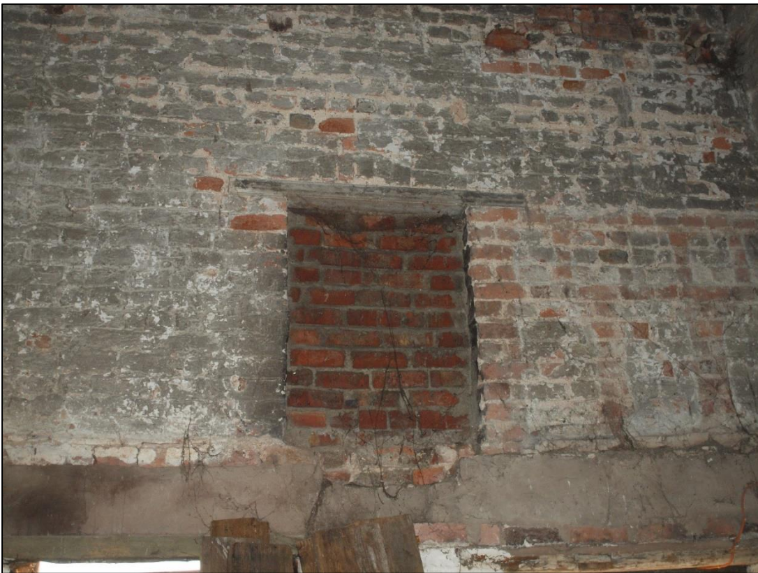
Plate 48: Blocked first floor opening
