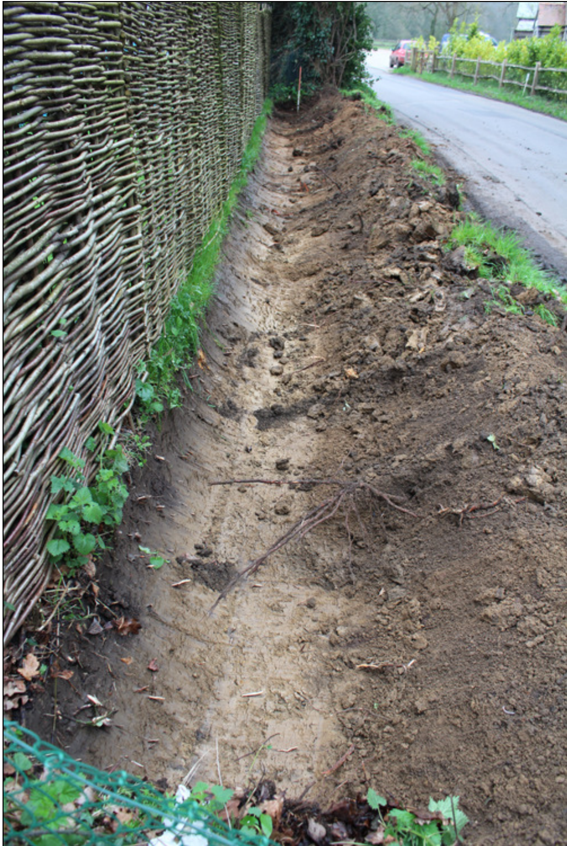
Figure 4 The trench for the new hedge to the front of the existing house (No.3 in Fig.2), looking south-east.
