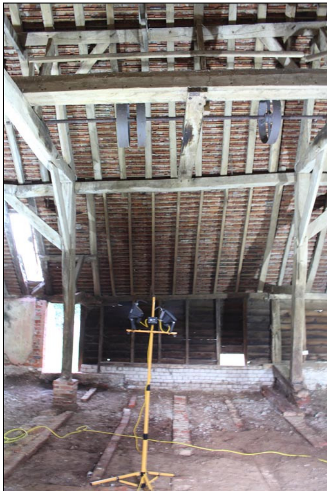
Figure 55 The northern threshing bay, looking east. The three later drive wheels can be seen in the roof space over the brick partitions set into the floor below
