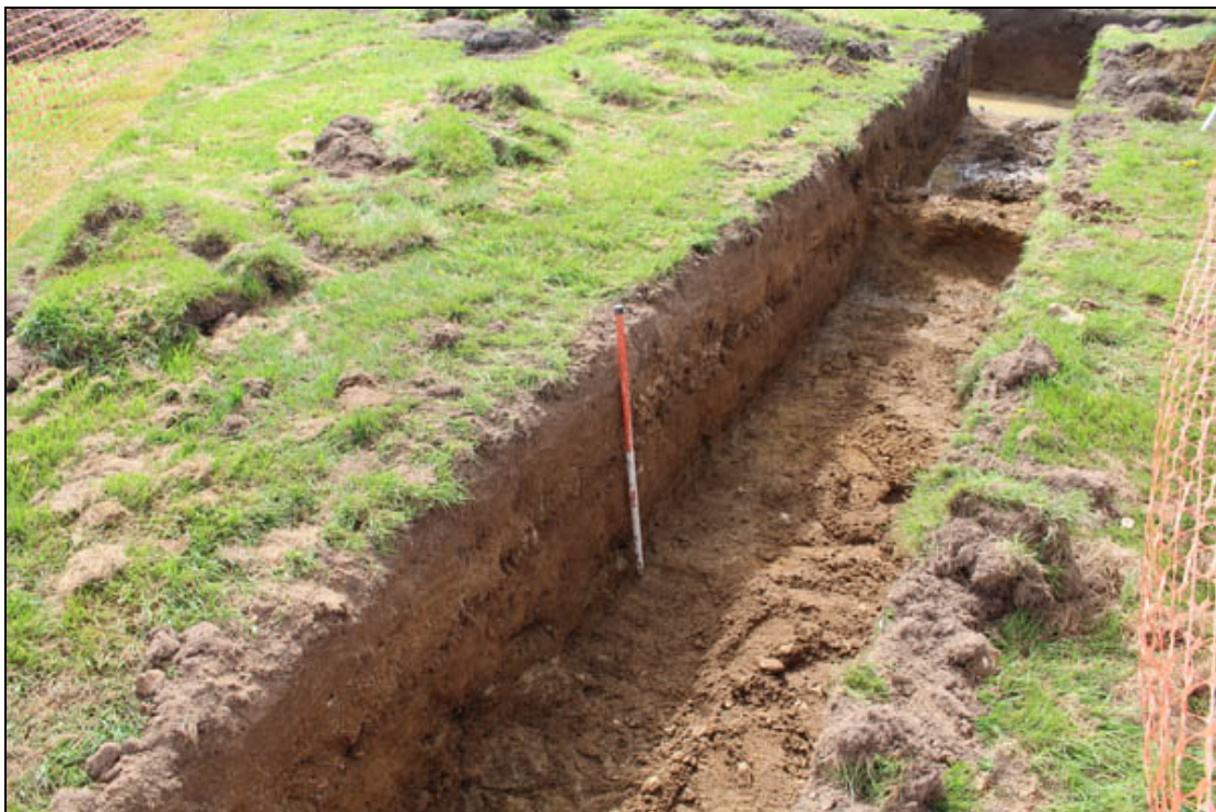
Figure 15 The spread of flint gravel (14) and wall foundation (16) beyond, within the Trench 3 extension
