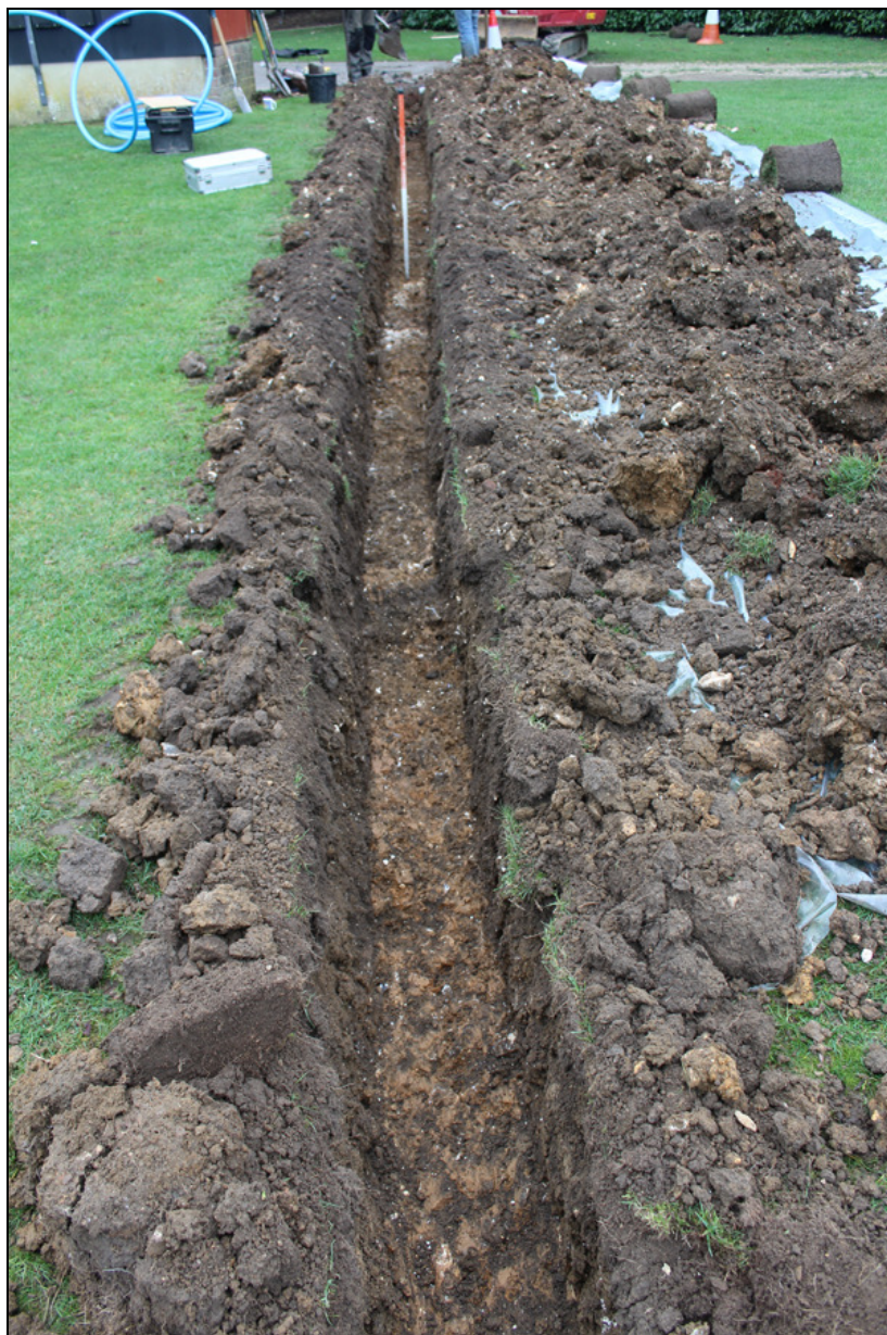
Figure 4 The water pipe trench north of the terraced slope, the pit/ditch lies just behind the 1m scale
