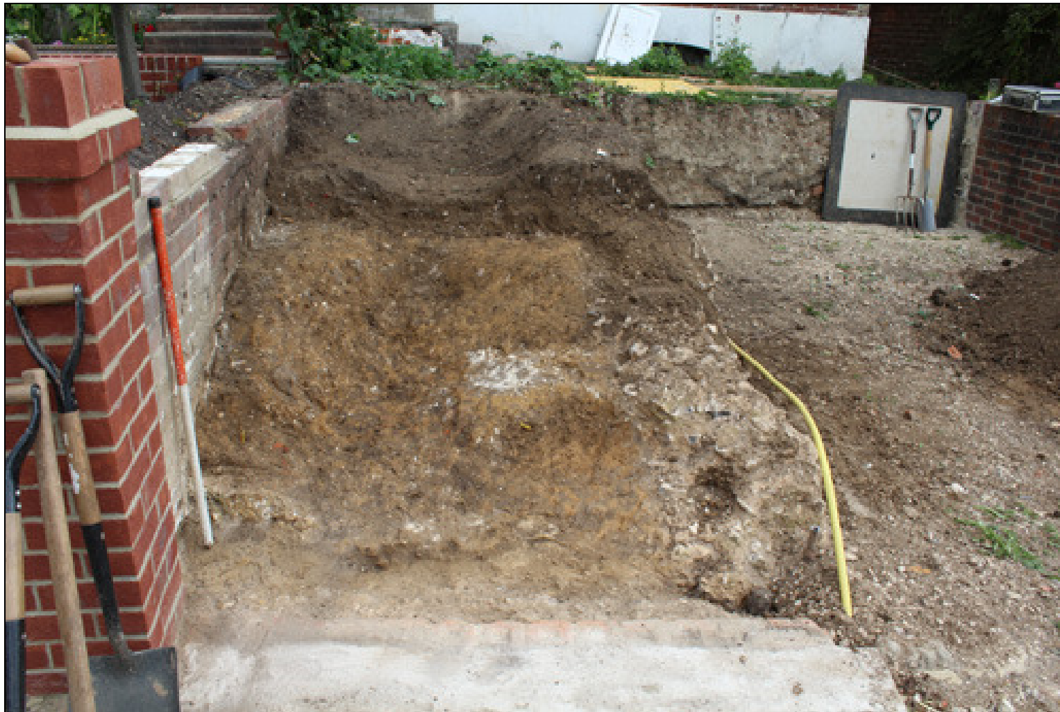
Figure 8 The excavated trench after the removal of the modern layers (1) & (2), looking north. The re-deposited brickearth (10) can be seen over the front edge of the eastern chalk floor (9)
