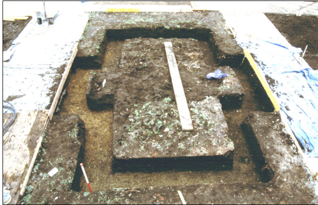
Fig.3 Photograph of the greenhouse foundation trench, indicating the layers revealed under the topsoil.
