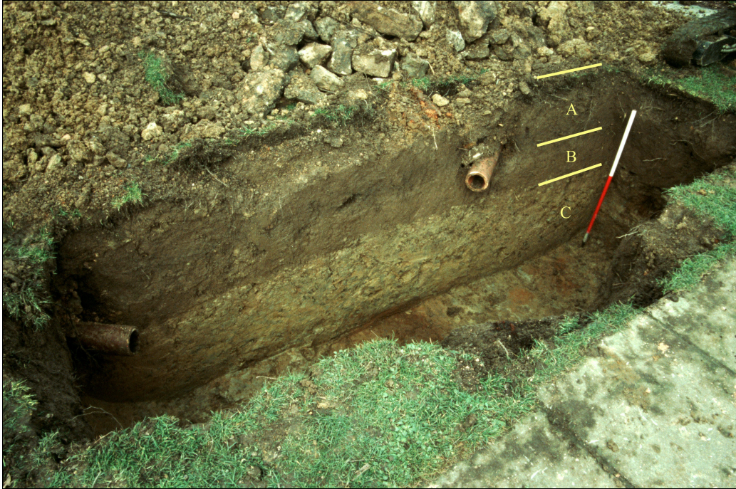
Figure 10 The north face of the soak-away trench in Room 13, showing the three layers. A is the topsoil, B is the possible early buried soil layer and C is the Upper Greensand. The scale is 1m.
