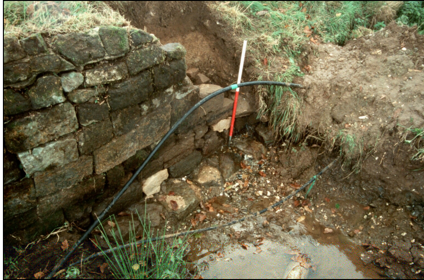
Fig.13 Photograph of the ha ha wall in trench 4, looking north-west. The scale is 1m.
