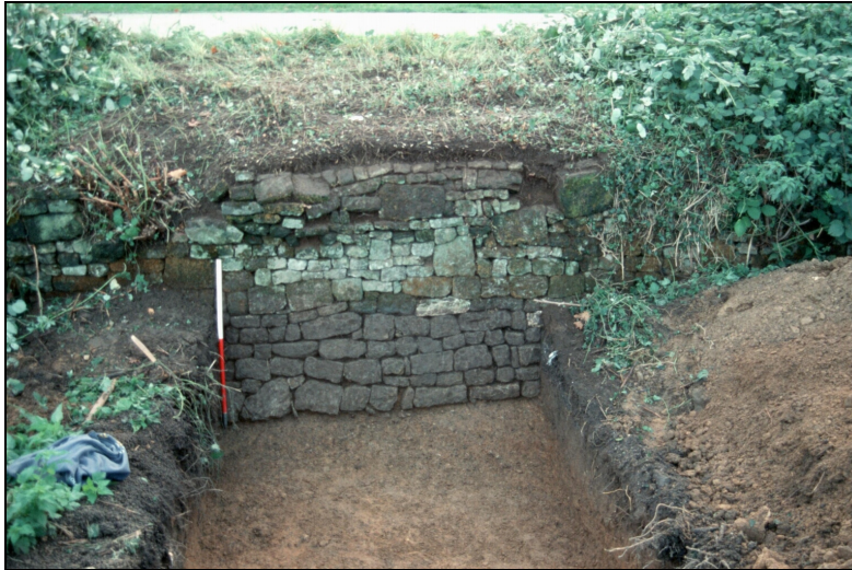
Fig.5 Photograph of the ha ha wall in trench 1, looking south-west. The scale is 1m.
