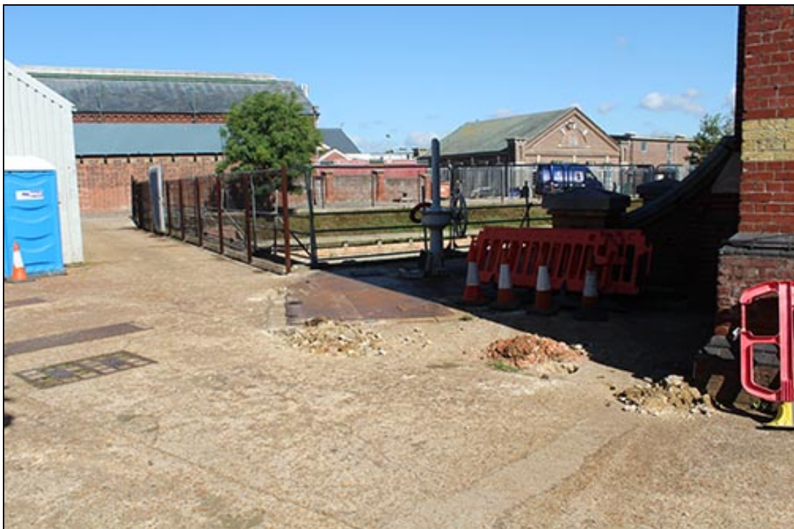
Figure 4 Site shot looking north-west, with the Post-holes 7 – 10 visible in the foreground and the newly erected posts within Post-holes 1 – 6 in the background
