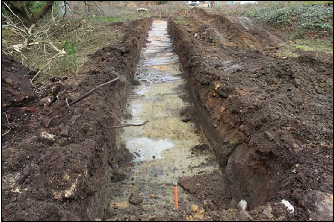
Figure 8 Trench 2 looking north, showing the deeper layers of both historic topsoil and redeposited clay silt & rubble at its south end. The dark patch in the middle ground is the effluent from the severed modern land drains
