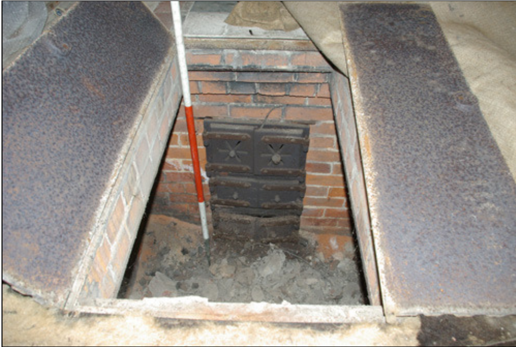
Figure 18 The brick chamber containing the front of the stove, looking north. The scale is divided into 0.5m sections.
