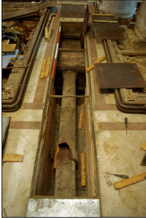
Figure 19 The exhaust pipe exiting from the boiler, looking south. The scale is 2m.
