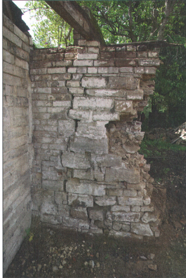
Figure 7 The surviving part of the north courtyard wall as re-used by a late 19 th century cart-shed, looking south.
